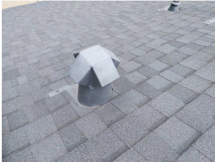
Unapproved roofjack used for dryer vent pipe
