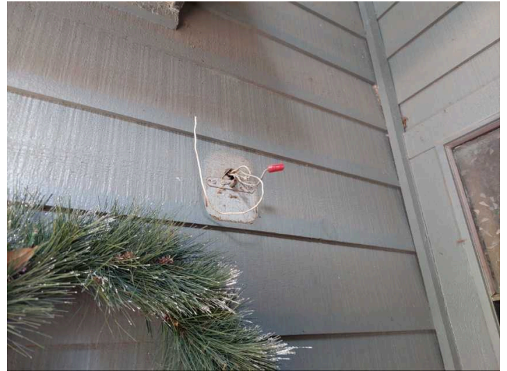
Missing front porch light
