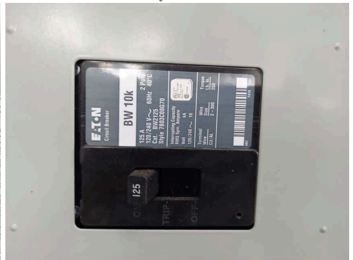
Main breaker (125A)
