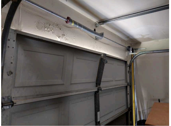
Garage door is damaged.
