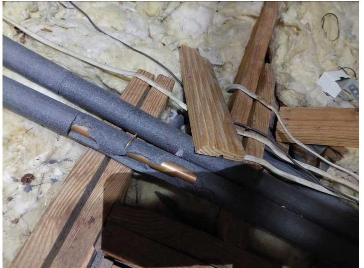
Picture of water supply lines - copper
