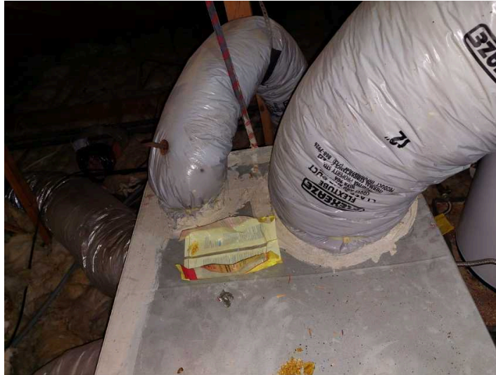
Picture of ducts in attic
