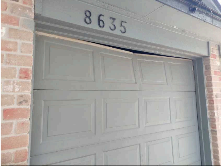
Garage door is damaged.
