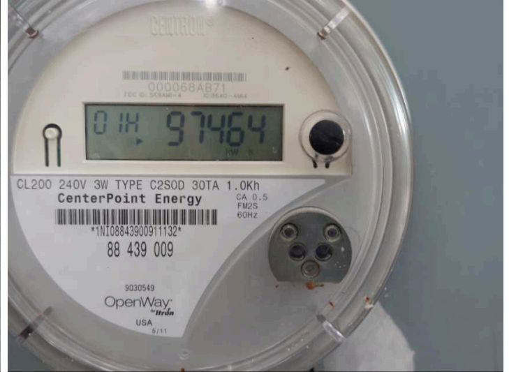
Picture of electric meter
