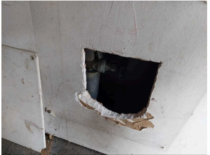
Main water shutoff valve
