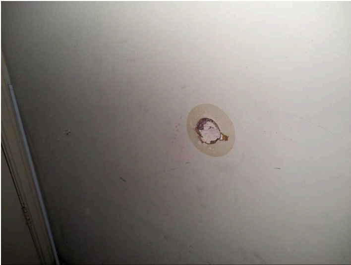
Interior wall damage in garage
