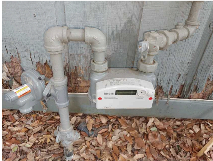
Picture of Gas Meter
