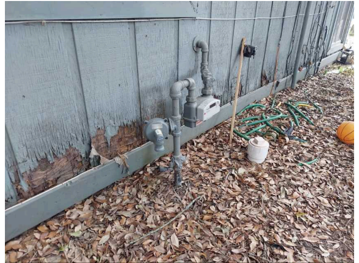
Damaged siding back side of house.
