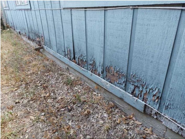
Damaged siding right side of house.
