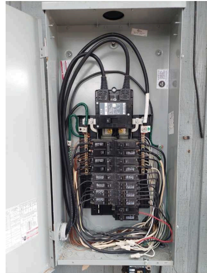
Picture with deadfront panel removed
