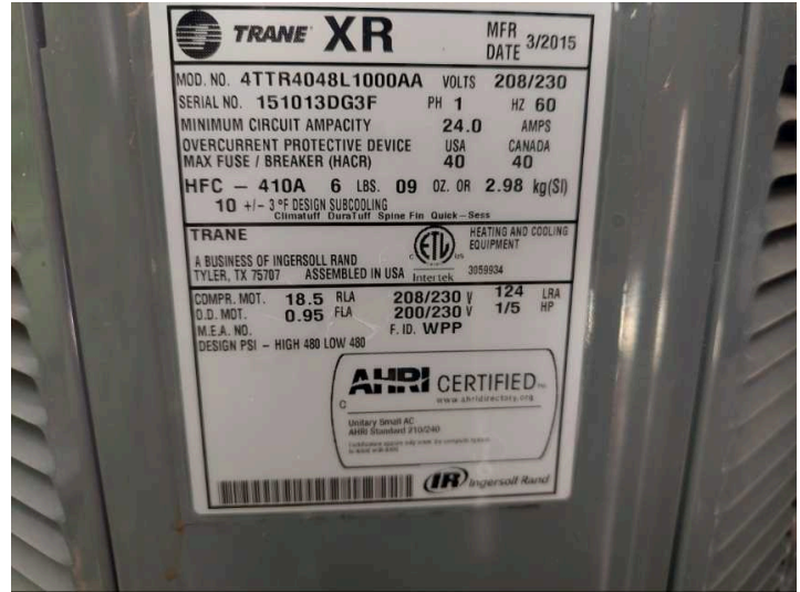
AC condensing unit data tag (2015)
