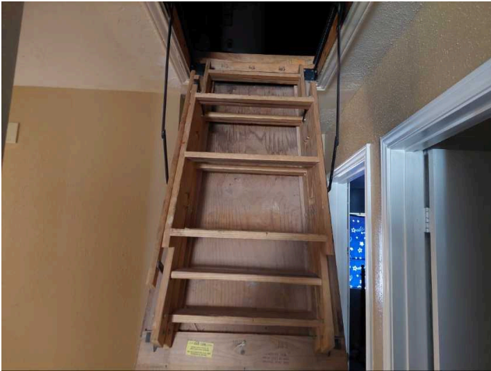
Attic access missing insulation.
