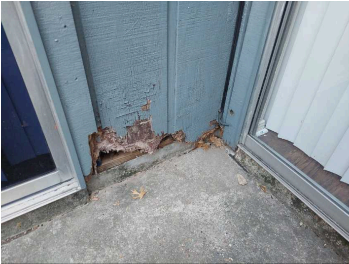
Damaged siding back side of house.
