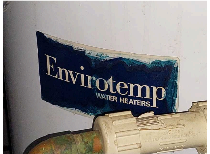
Water heater brand name
