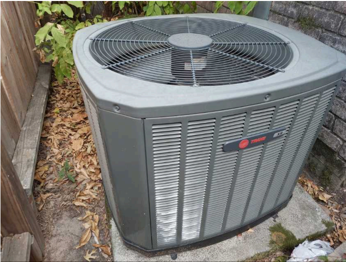
AC condensing unit
