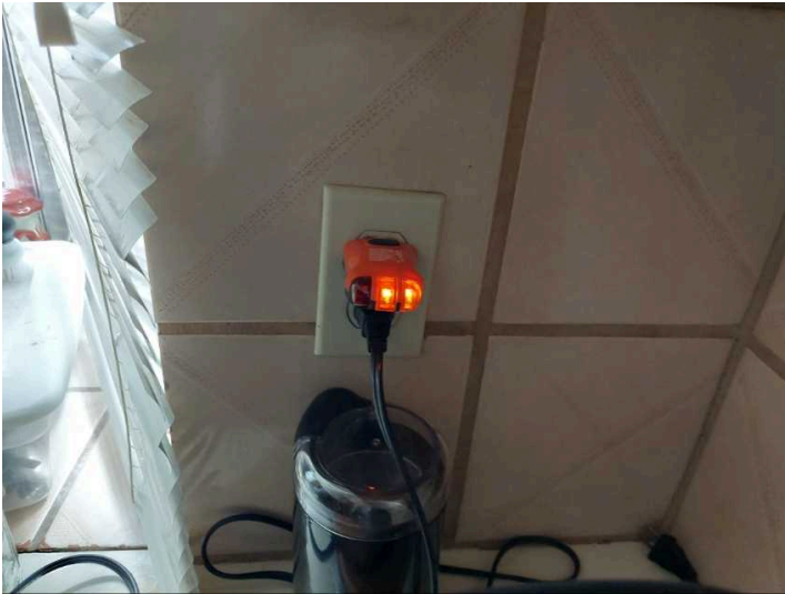
Kitchen electrical receptacle not GFCI protected
