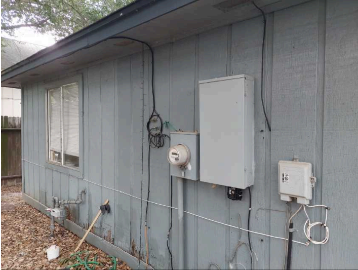
Picture of electrical service panel
