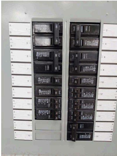
Picture of breakers
