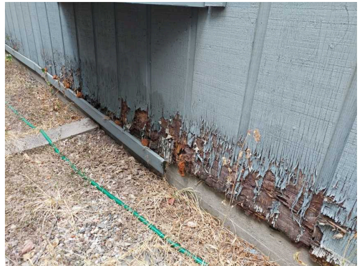
Damaged siding left side of house.
