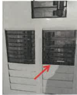
Missing knockouts on dead-front.
