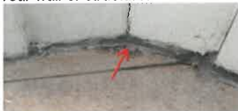
Sealant present along rear side of exterior siding, near porch.
