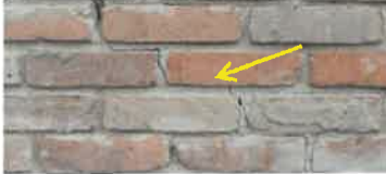
Under kitchen area, diagonal crack present on left wall of house.
