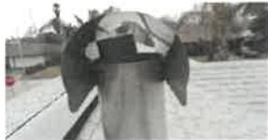
Improper furnace vent cover for type B vent.
