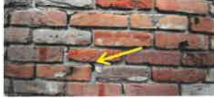
Diagonal cracks along left exterior wall of structure.
