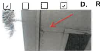
Damage present to soffit board along left side of structure near garage.
