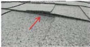
Pop shingles present in multiple areas on front half of gable roof.
