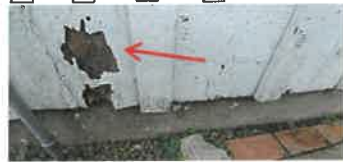
Damage to exterior siding on rear wall of structure.
