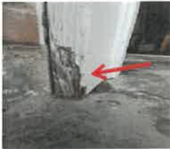
Damage to overhead garage door frame.
