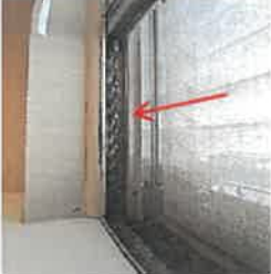
Window balance spring has fallen down in dining room window.
