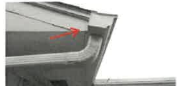
Loose gutter at back right corner
