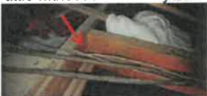
Electrical wiring is improper and runs over attic entrance.
