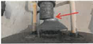
Vent pipe not attached to draft hood.
