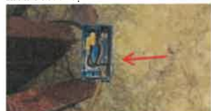
Junction box in attic lacks cover.
