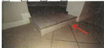
Steps in kitchen leading to breakfast area could create a trip hazard.
