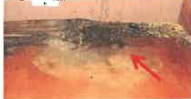
Damage to underneath kitchen
