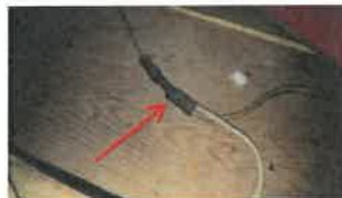
Electrical splice present in attic without the use of j-box.
