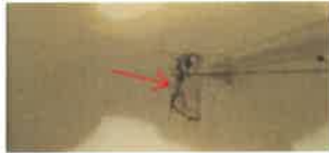
Wall covering damage in master bdrm.
