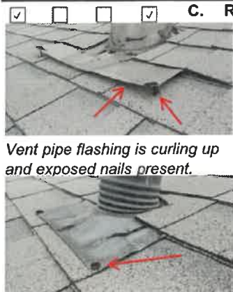
Vent pipe flashing is curling up and exposed nails present. Exposed nails present on vent pipe.
