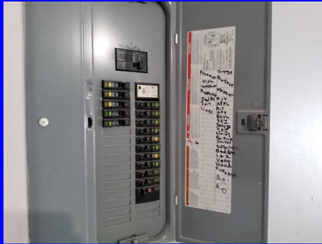
Electrical Main/ Service panel - Garage
