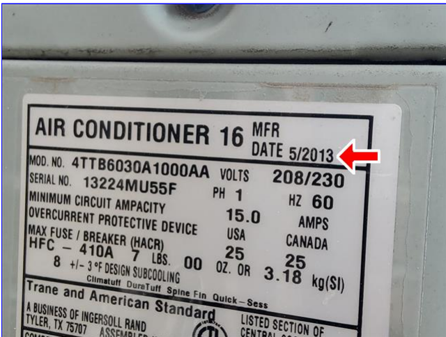
B. Item 3 (Picture) Condenser data plate
