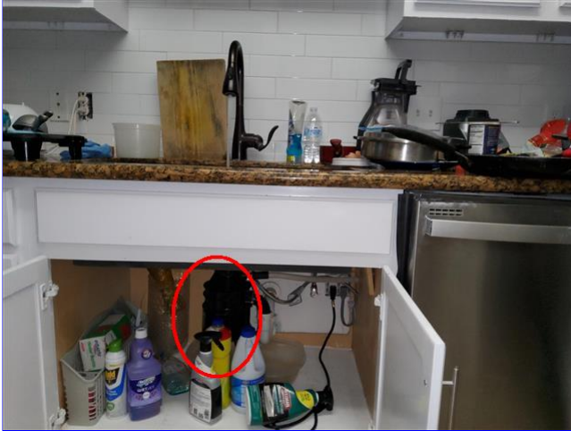
B. Item 1 (Picture) Garbage disposal -Tested
