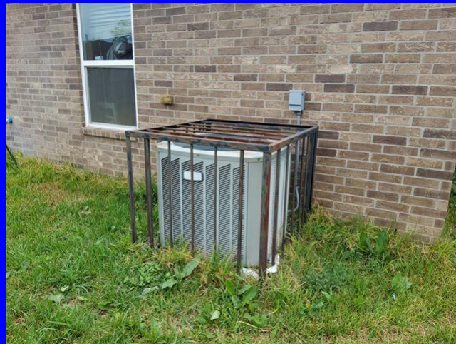
Condenser - Back side
