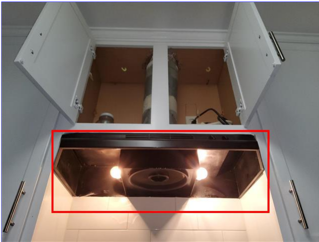
C. Item 1 (Picture) Kitchen exhaust fan
