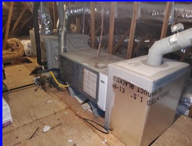
Furnace -Attic Space
