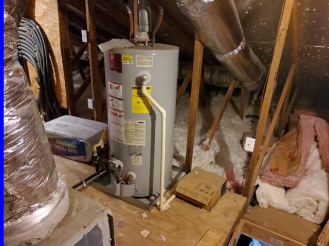
Water heater -Attic Space
