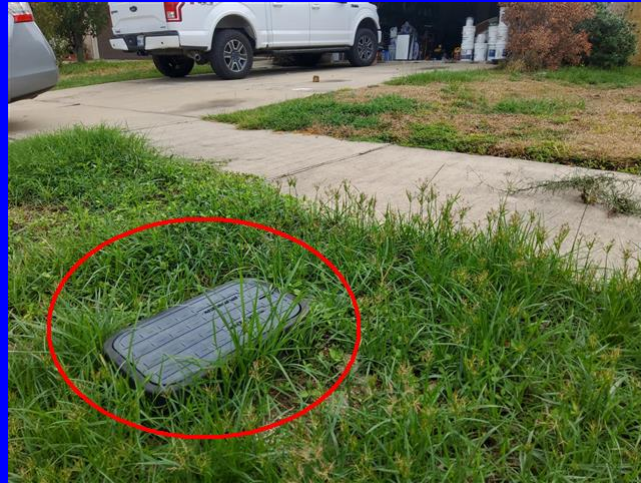
City meter water shut off - Front side
