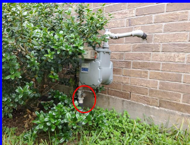
City meter gas shut off - Right side
