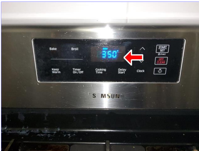
D. Item 2 (Picture) Oven -Tested
