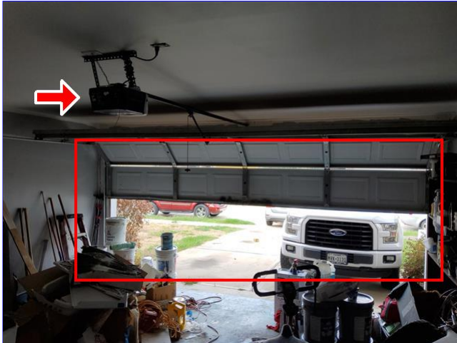
G. Item 1 (Picture) Garage door operator -Tested
