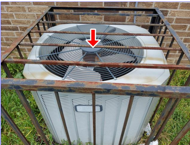
B. Item 2 (Picture) Condenser
