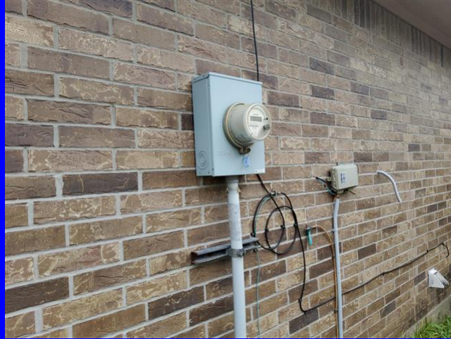
Electrical city meter - Right side
