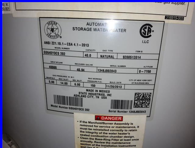
Water heater -Data Plate
