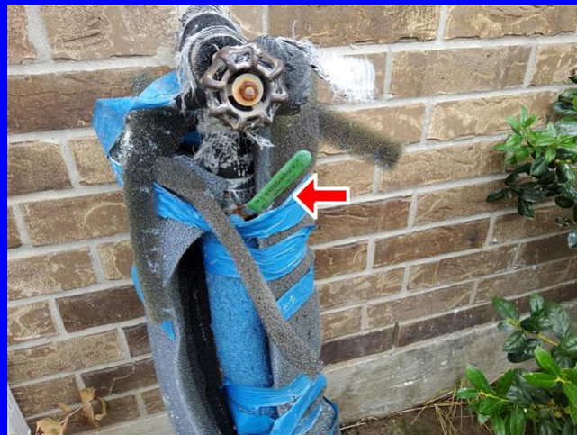
Main house water shut off - Right side
