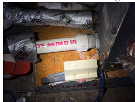
East AC drain pan is very rusted.
