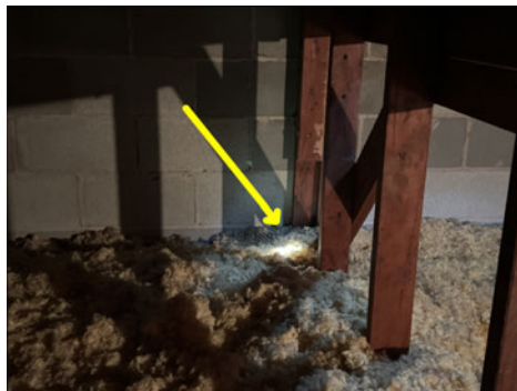
Daylight observed in the attic at multiple unintended locations.
