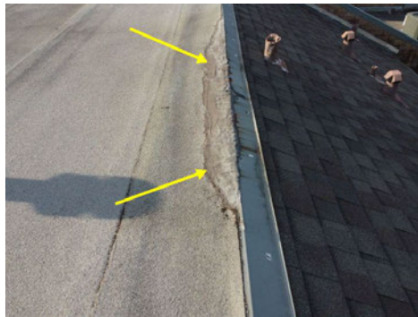
Flat roof damage/repair observed on the roof.
