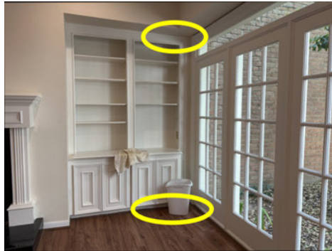
The master shower leaked through the ceiling onto the floor in the living room during operation.
