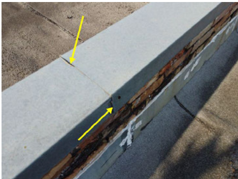
Roof flashing/cap flashing not sealed at seams and joints.
