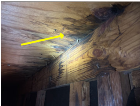
Observed multiple areas of water stains/wood rot in the attic.
