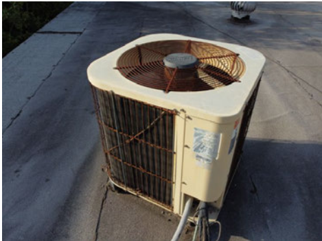
The west condenser unit data plate is damaged. Information no longer visible.
