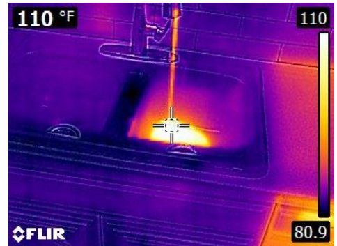
The water heater heated as intended at the time of inspection.
