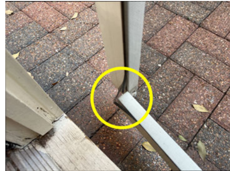
The courtyard screen door is damaged.
