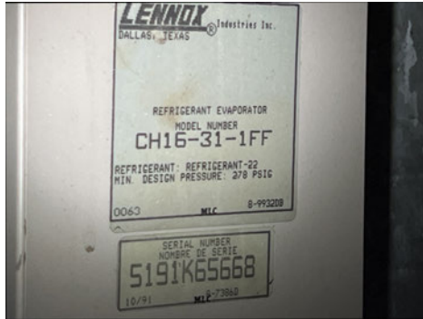
West evaporator: Lennox 2.5-ton 1991 R22
