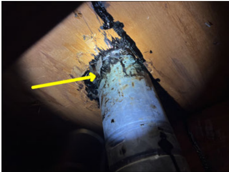
Improper tar repairs observed around hot vents.
