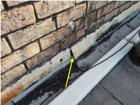
Counter flashing damaged at multiple locations on the roof.
