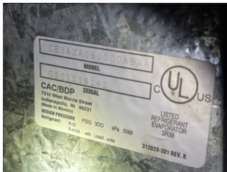
East evaporator: Carrier 5-ton 2003
