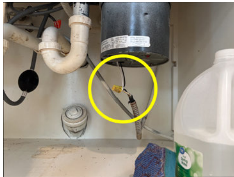
Wiring and electrical conduit not secured below the disposal.
