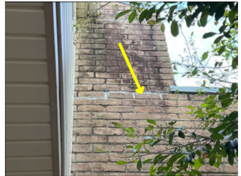
Brick cracks/repared cracks observed.
