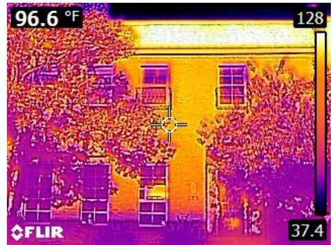
Infrared image of home during the inspection.
