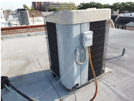
The east condenser unit data plate is missing.
