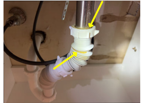
Small leak observed below the left master bath sink.
