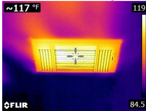
The east furnace heated as intended at the time of inspection.
