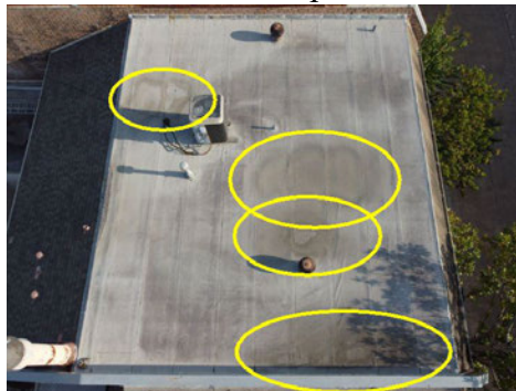
Observed multiple areas of water stains/evidence of ponding water on both flat roofs.
