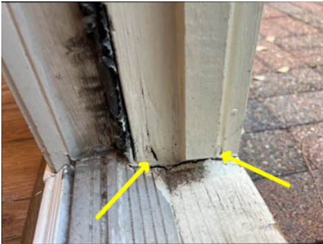
Wood rot observed at courtyard door/frame/trim.
