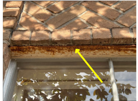
Lintels need paint.
