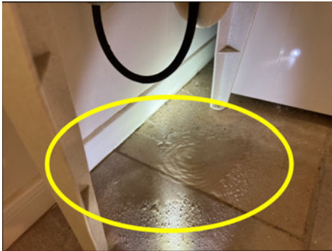
Water leak observed below the laundry room sink.
