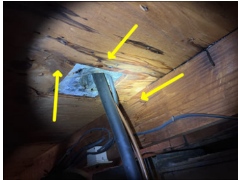
Multiple water stains observed on roof decking/attic framing. Dry at the time of inspection.
