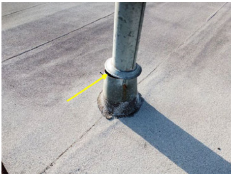
Misaligned storm collar observed on one or more hot vents.
