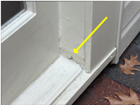
Exterior wood rot observed at multiple locations.
