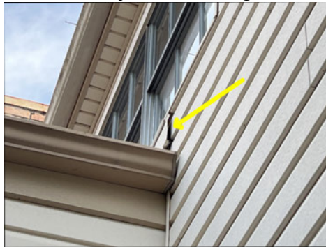
Damaged/loose siding observed.
