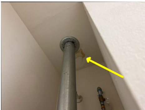
Water stain at ceiling above the water heater. Dry at the time of inspection.
