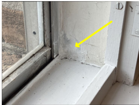
Water stain/damage at multiple window jambs. Dry.
