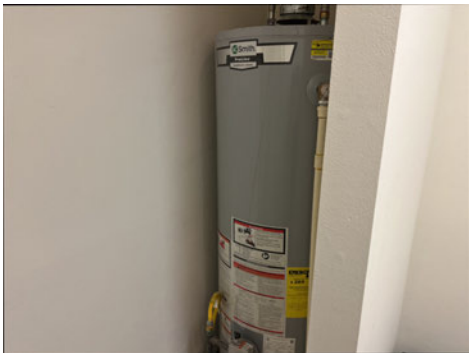
Water heater: A.O. Smith 2021
