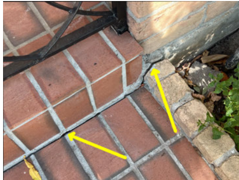
The front patio steps have settled/cracked.
