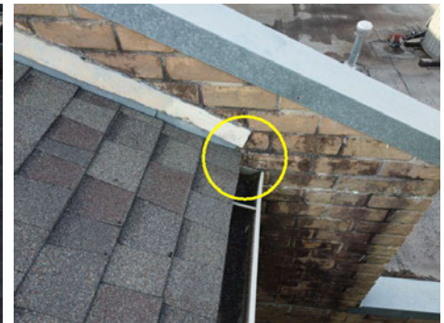
Kick-out flashing missing at multiple areas on the roof.
