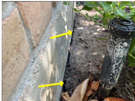
The soil has pulled away from the foundation wall at multiple locations.
