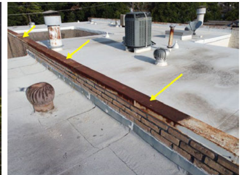
Multiple areas of rusted flashing observed on the roof surface.
