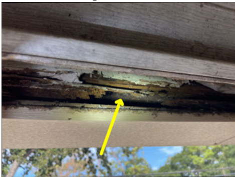
Observed wood rot above the garage door/garage door header.
