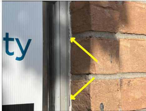
Seal all exterior windows/vertical trim/joints in siding.
