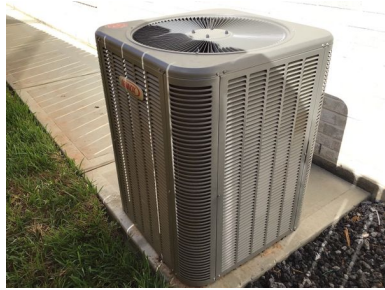
General Photos of HVAC Equipment:
