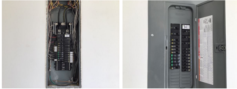
General Infrared Photos of Distribution Panel(s):
