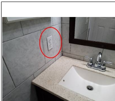
Outlet is near a wet location and needs to be under the protection of a GFCI
