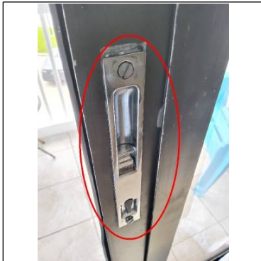
Hardware is loose
