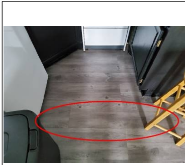
Unevenness at the kitchen threshold
