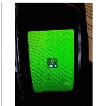
Return air temperature reading was 66°
