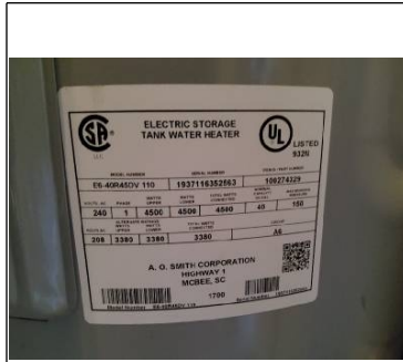
Water heater was manufactured in 2019 and is rated at 40 gallons
