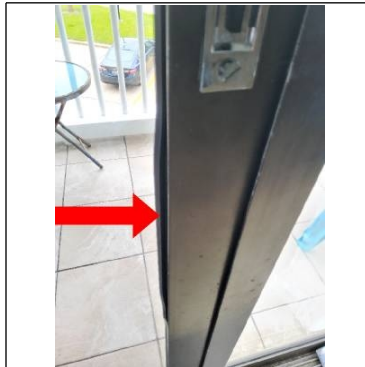
Rubber gaskets are coming loose
