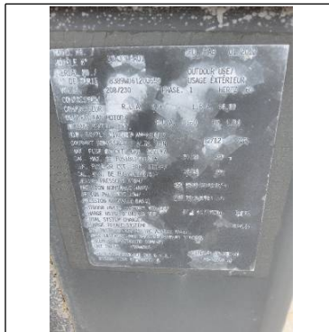
Exterior unit was manufactured in 2012, is rated at 1 1/2 tons and uses the newer refrigerant R410A
