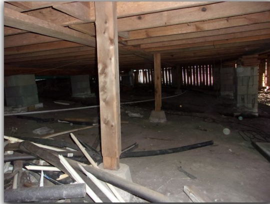
Signs of Structural Movement or Settling
