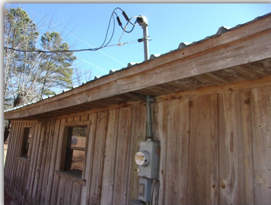
Unable to verify ground rod
