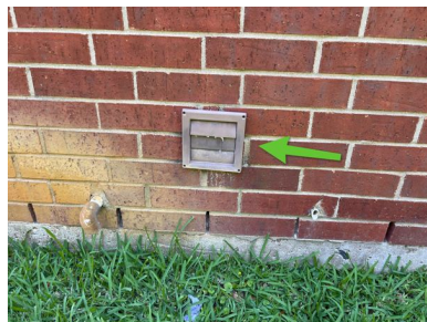
Dryer Vents: : Through Side Wall
