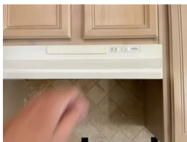
Photo - Exhaust Termination:
