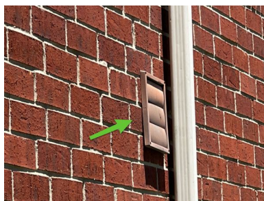
Range Exhaust: vents to the exterior
