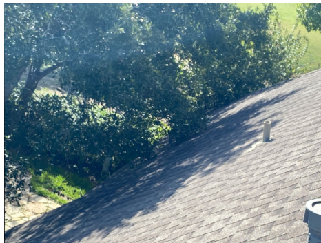
Tree limbs in contact with the roof can/ will damage the roof.
