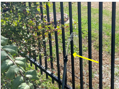
Damaged water line, water gusher in the yard; Station 3
