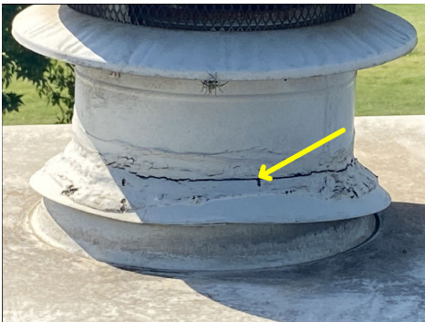
Storm collar needs caulking on the chimney.
