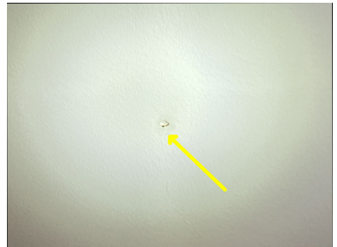
Impact damage observed at garage entry door
