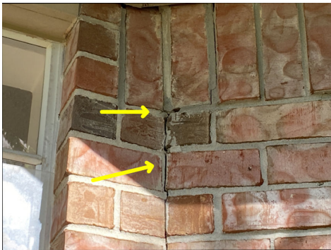
Brick cracks observed at South exterior wall
