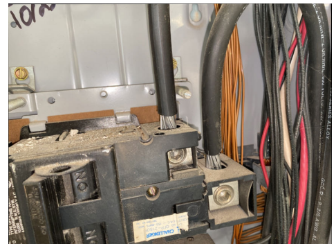
Aluminum feeder wires at main panel in garage
