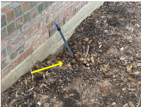
Depressions in soil near foundation are detrimental to good foundation maintenance, recommend filling in depressions.
