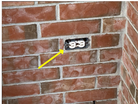
Front entry missing weatherproof covering
