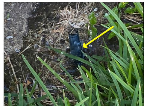
Damaged water line, water gusher in the yard; Station 4
