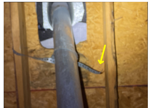
Vent pipe(s) not properly secured (strapped) in place.
