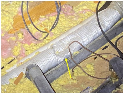
The exhaust duct is crimped/crushed in the attic.
