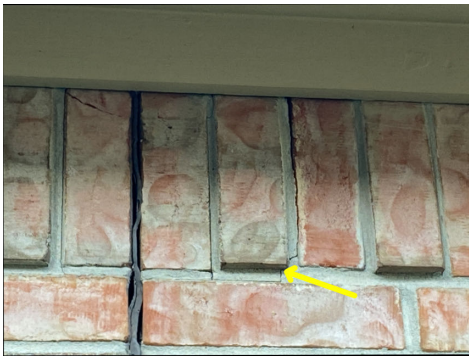
Typical cracks observed on East exterior wall
