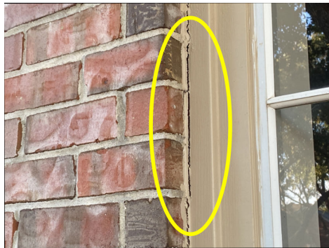
Missing/deteriorated sealant around windows observed in multiple locations
