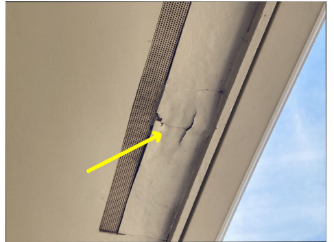
Wood rot observed at the southwest corner of home
