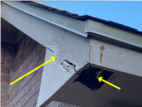
Wood rot observed on East exterior side of home
