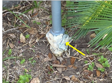
Gas shut off located at meter on South exterior wall
