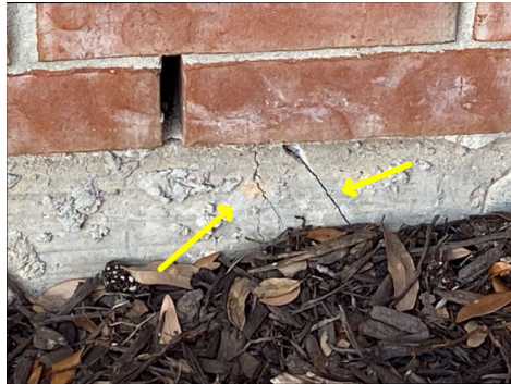
Foundation crack observed south of garage door
