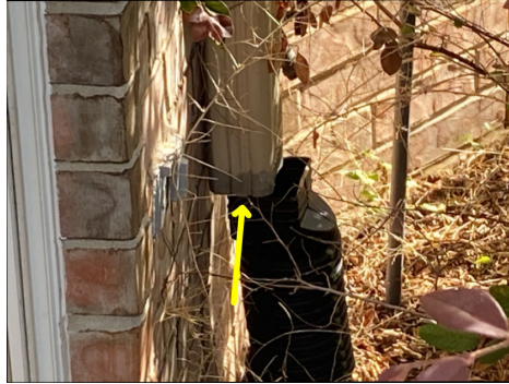
Downspout needs to be better connected to the drain system at one or more locations.
