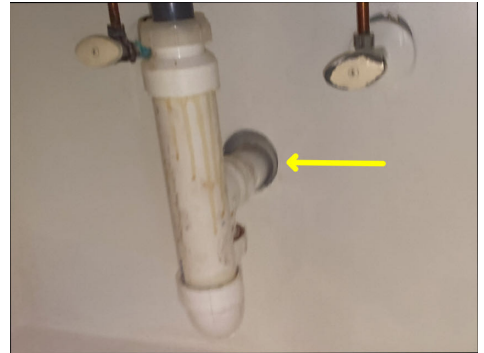
Recommend sealing all holes in cabinets to reduce air and water infiltration.
