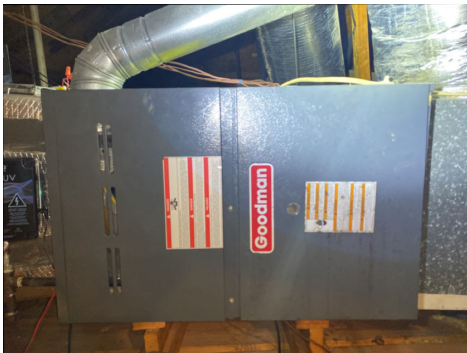
Furnace located in attic
