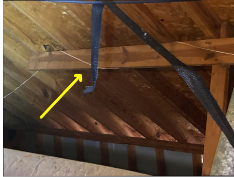
Observed insufficient purlin (roof bracing) struts (supports) in the attic.
