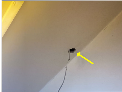
Recommend repairing holes/openings in garage walls/ceiling.
