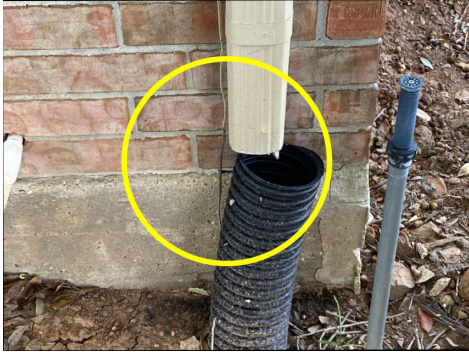
Downspout needs to be better connected to the drain system at north exterior wall.
