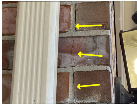
Cracks in brick/stone veneer and/or repairs, at northwest exterior wall of garage
