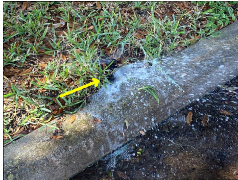
Damaged water line, water gusher in the yard; Station 1
