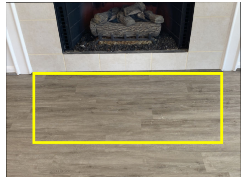
Inadequate sized non-combustible hearth extension at sides of the fireplace.
