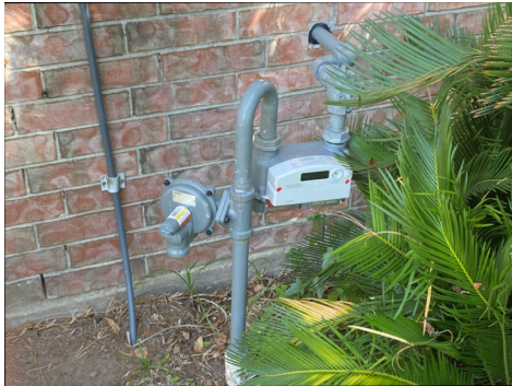
Gas meter located on South exterior wall
