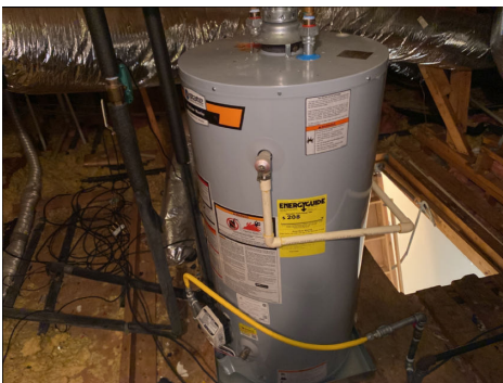
Water heater located in attic
