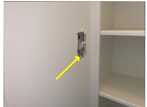
Pantry cover plates were either missing or damaged.
