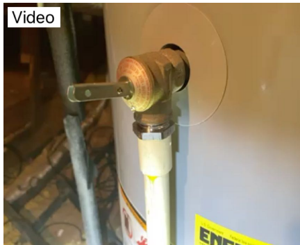
TPR valve leaks water when tested service/repair/replace as necessary.
