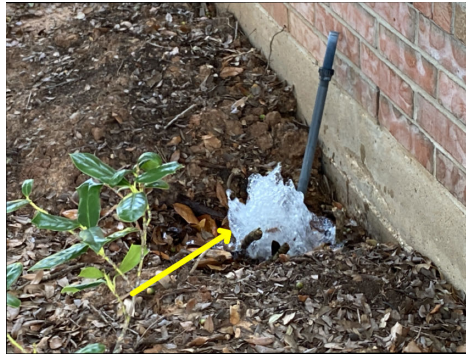
Damaged water line, water gusher in the yard; Station 2
