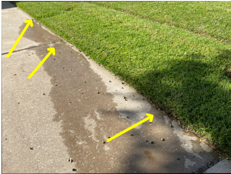
Zone 1 spray heads are clogged and / or grass has grown over head, blocking / preventing proper operation.
