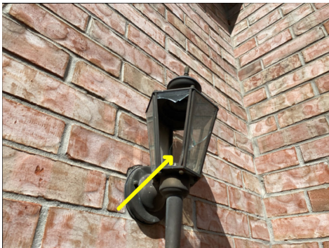
Is porch exterior light light fixture damaged.
