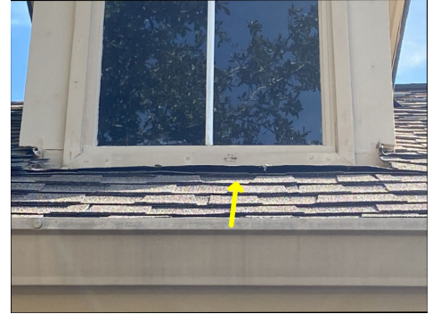
Lower edge of flashing not sealed.
