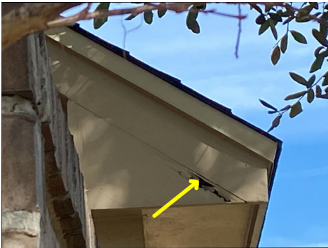
Wood rot observed on east exterior wall south of home
