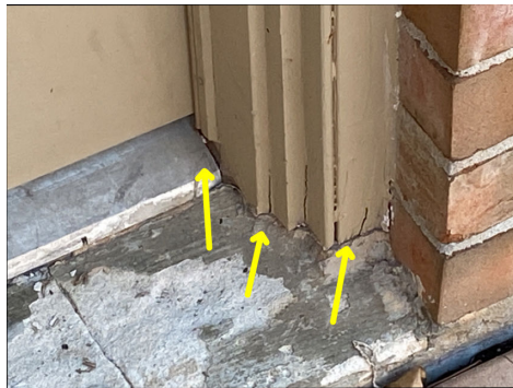
Missing/deteriorated sealant at door threshold observed at multiple locations
