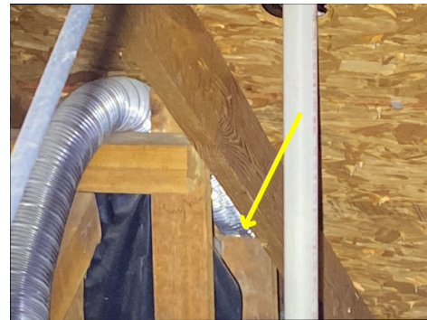
Exhaust fan improperly vents into the attic, should vent to the exterior.
