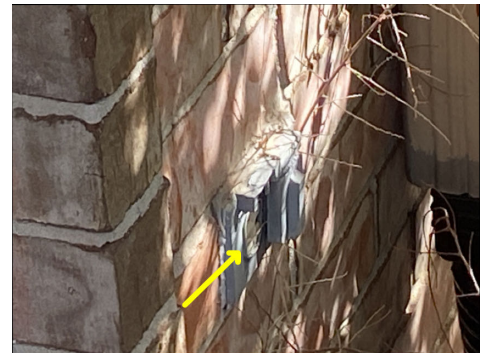
Damaged covering at South exterior outlet
