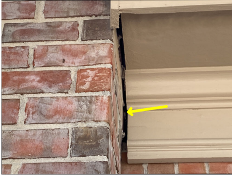
Missing/deteriorated sealant at frieze board and brick intersection on North exterior wall
