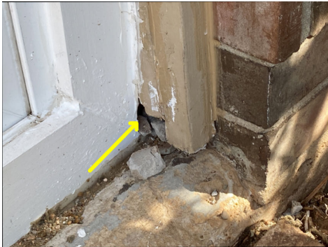
Gaps at joints in building components are potential pest / rodent entry points.
