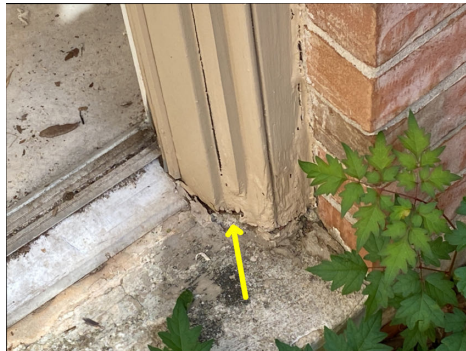
Wood rot of lower door and/or jamb; garage east door
