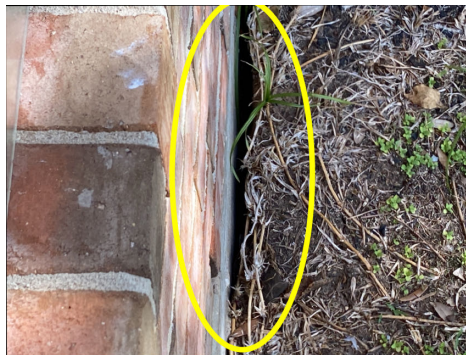
Soil pulled away from foundation at Southside of home
