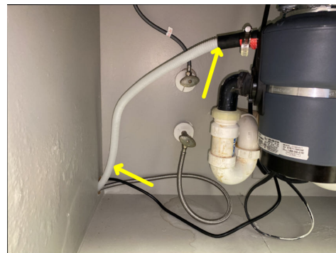
Drain line needs to be better elevated and secured above side inlet of disposal.
