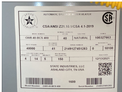
2021 State natural gas water heater
