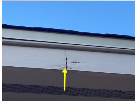
Wood rot observed on East side of home
