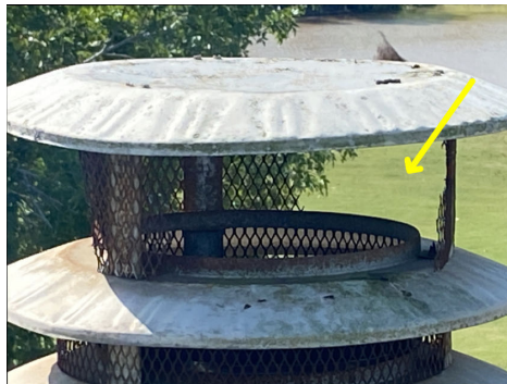
No spark arrestor on top of flue.
