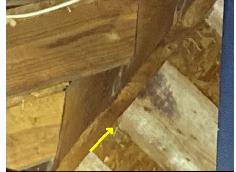
Ridge and/or valley board(s) not deep enough to support ends of rafters.
