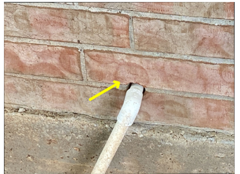
Missing/deteriorated sealant at North exterior wall
