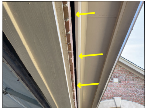
Frieze board separation at West exterior walls garage
