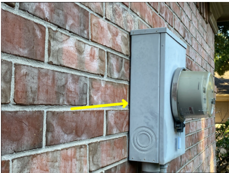
Missing/deteriorated sealant at meter box.
