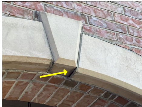
Cracks in the brick arch were observed. Loose bricks are hazardous.
