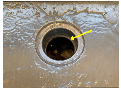
Rubber splash guard is missing.
