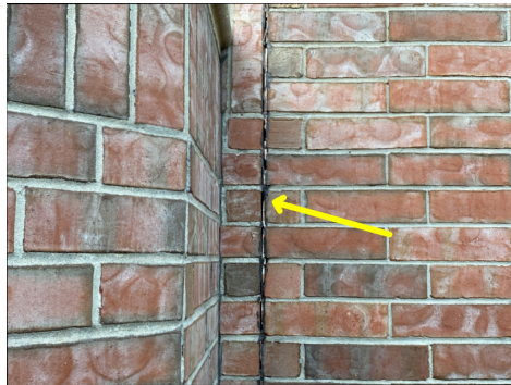
Expansion joint needs caulking.
