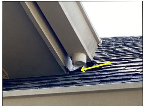
Gaps at joints in building components are potential pest / rodent entry points.
