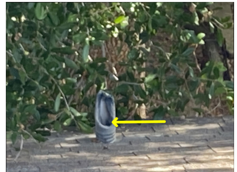
Not all lead flashing of drain waste vents are properly rolled down interior of plumbing vent pipes and/or are damaged by squirrels.
