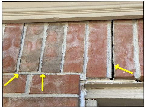
Brick crack observed at North corner of garage door
