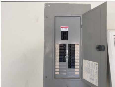
Exterior of main service, panel in garage
