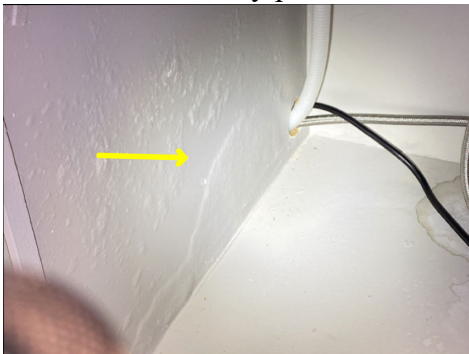
Water damage to the base of the cabinet below the kitchen sink.
