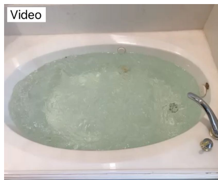
Spa tub was operational at time of inspection
