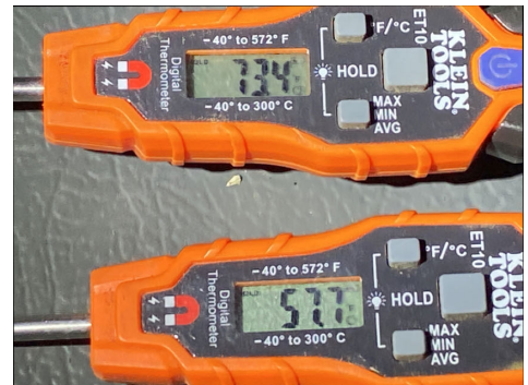
A/C was operational at time of inspection with a 15.7°F differential.
