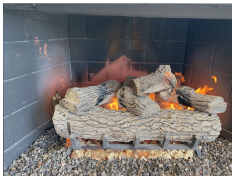
Fireplace with operational at time of inspection
