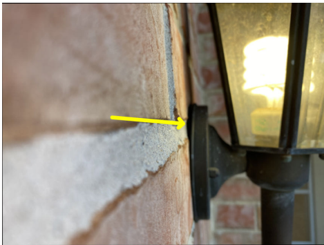
Missing/deteriorated sealants at exterior lights observed in multiple locations
