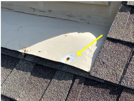
Exposed staples/nail-heads/fasteners observed on the roof are not properly sealed.
