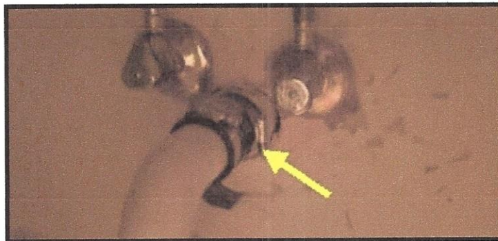
Flexible drainage connections were observed
