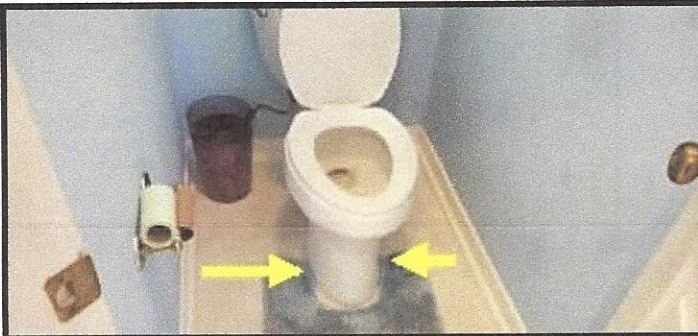
The commode is loose
