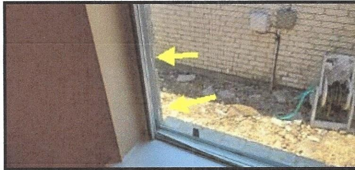
Missing or damaged windows screens
