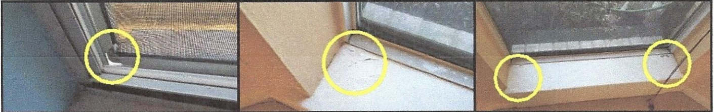
Missing or damaged windows screens
