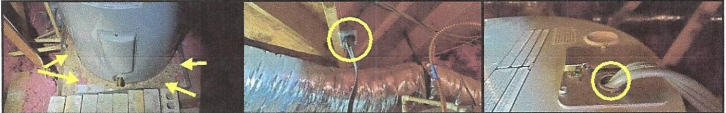
Debris/insulation was observed in drip pan
