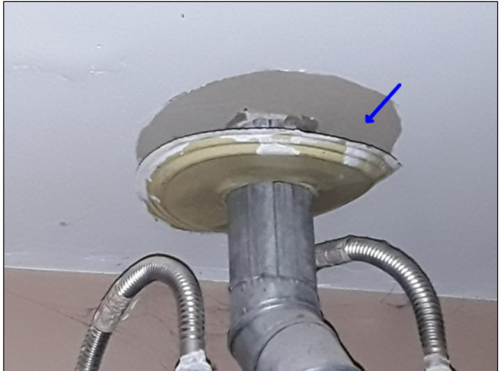
Flue collar not flush at ceiling.
