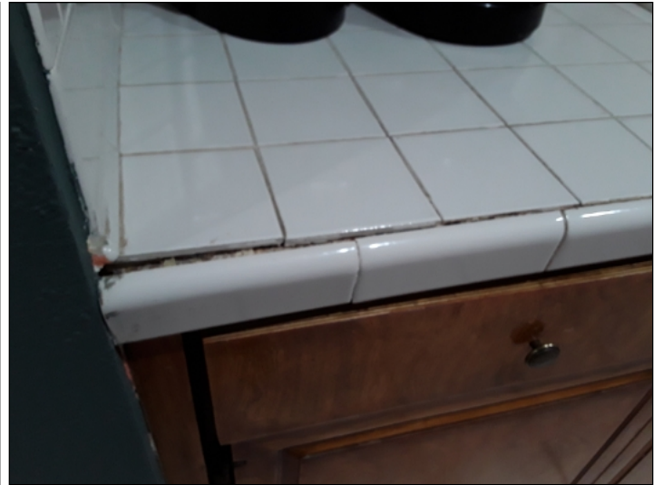
Countertop damaged. Mainly at - kitchen
