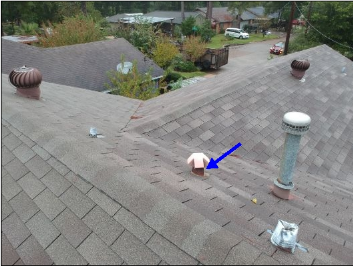
-There are signs of rusted flashing/vents on the rooftop. We recommend painting or replacing all rusted or deteriorated flashing/vents as needed.
