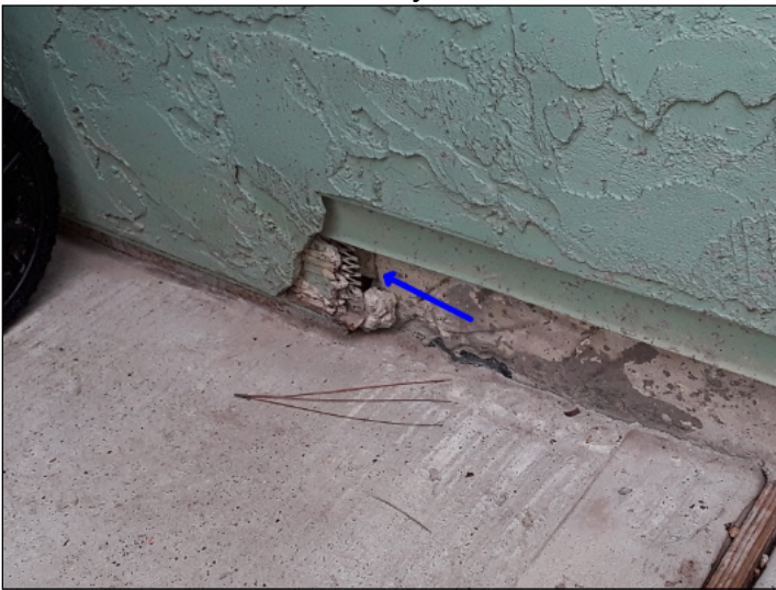
-Recommend sealing gaps & holes in stucco to help prevent water penetration. Mainly at - rear
