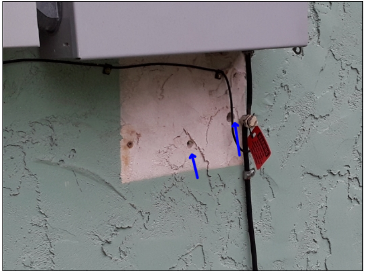
-Recommend sealing gaps & holes in stucco to help prevent water penetration. Mainly at - rear
