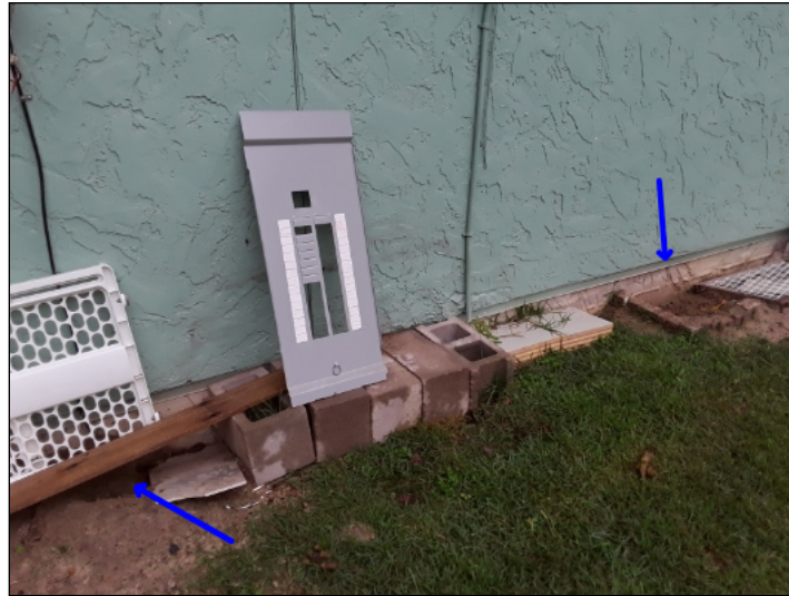
Holes noted at foundation. Mainly at - rear
