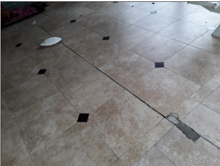
-Cracks were noted in the tile. Mainly at - patio
