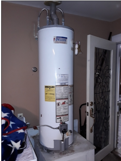
Overview of water heater(s)
