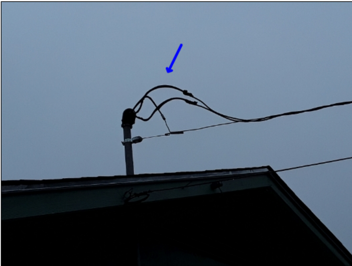
Improper drip loop. Recommend drip loops be formed on individual conductors to prevent the entrance of moisture into weather head.
