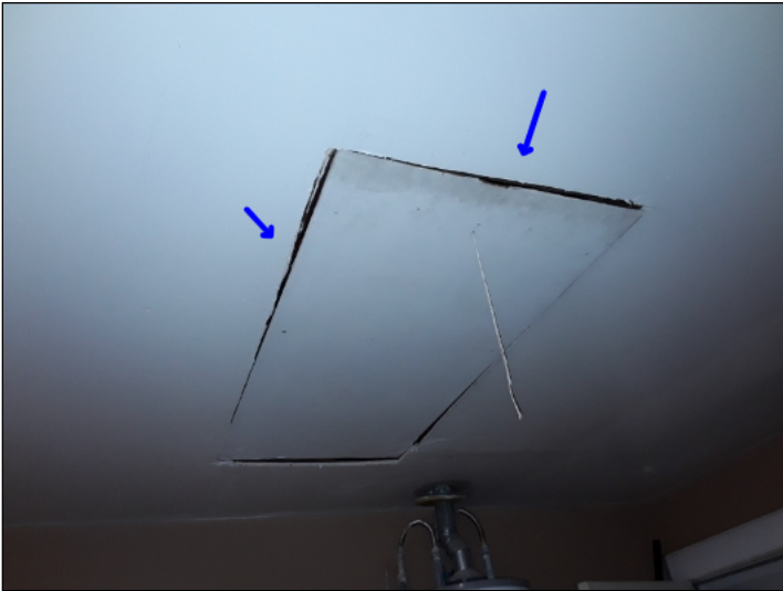
-There is no moulding around the attic stairway in the garage. Recommend adding trim to help maintain the proper fire break. The attic stairways are also not the proper fire rating by today's standards.
