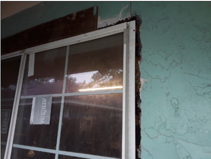
-Stucco is damaged, recommend repairs to help prevent water penetration. Mainly at - left (at garage window)
