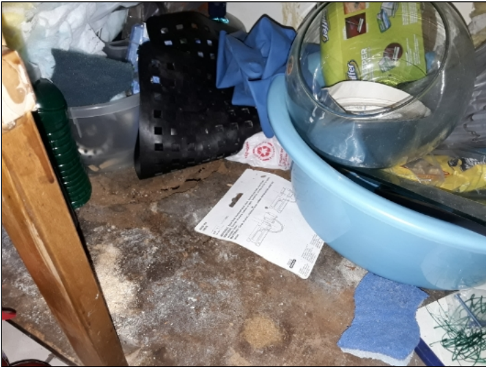
-The are signs of water damage in the cabinet under sink. Mainly at - kitchen
