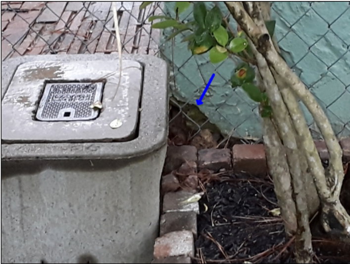
-Stucco is damaged, recommend repairs to help prevent water penetration. Mainly at - right
