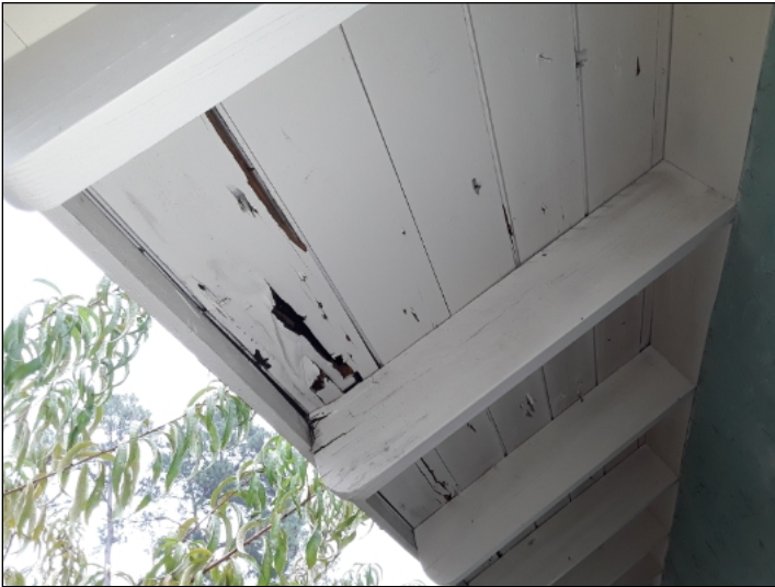
-Deterioration was noted at the soffit, recommend replacing all deteriorated soffit. Unable to determine the condition of the underlying materials. Mainly at - left rear
