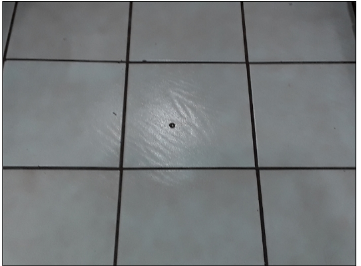
-Chips were noted in the tile. Mainly at - kitchen
