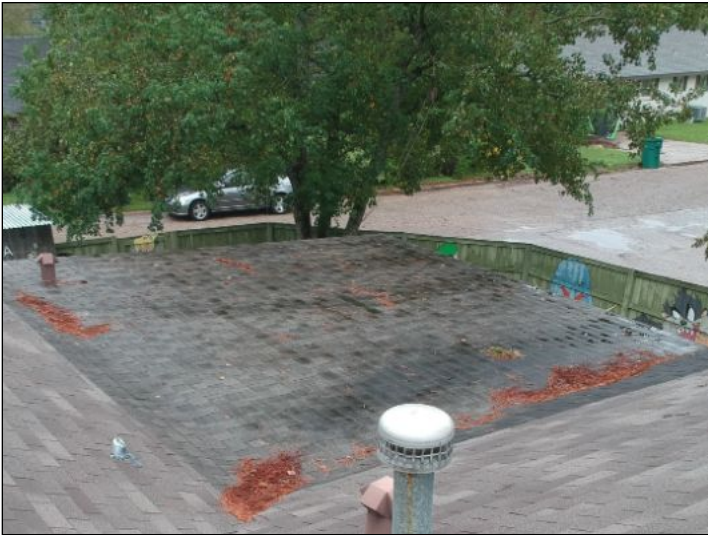
-Parts of the roof is ponding. This may cause leaks or damage to roof over time.
