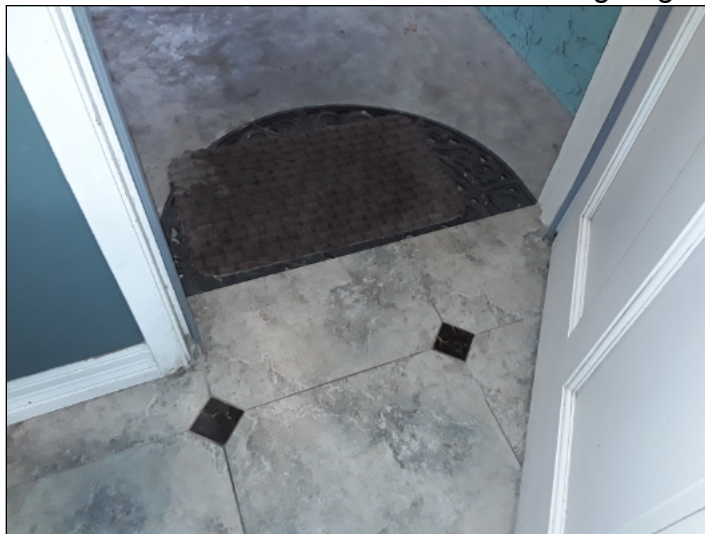
-The threshold is missing. Mainly at - front door
