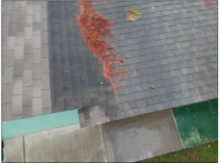
-Debris were noted on the roof which can cause water to back up on the roof and allow water to penetrate through the roofing materials, recommend removing debris from roof. Unable to fully inspect roof covering as debris limit the visibility of the roof surface.
