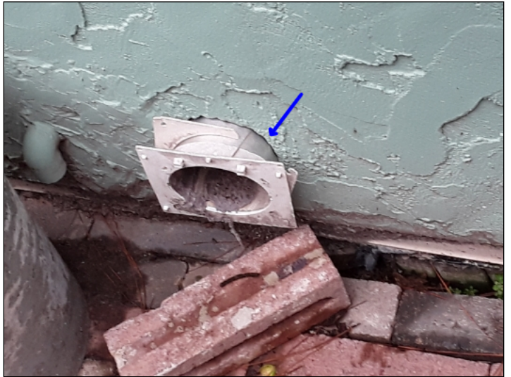
-A vent cover is damaged, recommend repairs to help prevent water penetration, rodent or bird intrusion. Mainly at - left
