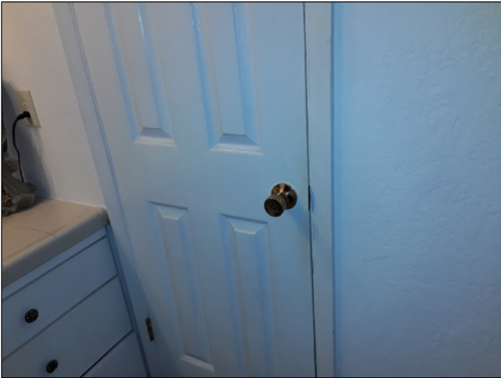
No access to closet at master bedroom. Locked.
