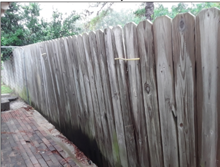
-Although fences are not inspected it was noted that the fence is showing some signs of damage or deterioration.
