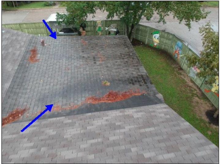
-The shingle roof covering had been applied over a surface with a pitch (slope) less than the industry standard, and is subject to leakage if proper underlayment was not used. Unable to determine if proper underlayment methods were used at time of inspection.
