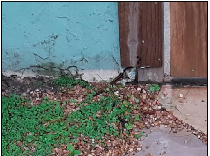
-Stucco is damaged, recommend repairs to help prevent water penetration. Mainly at - right
