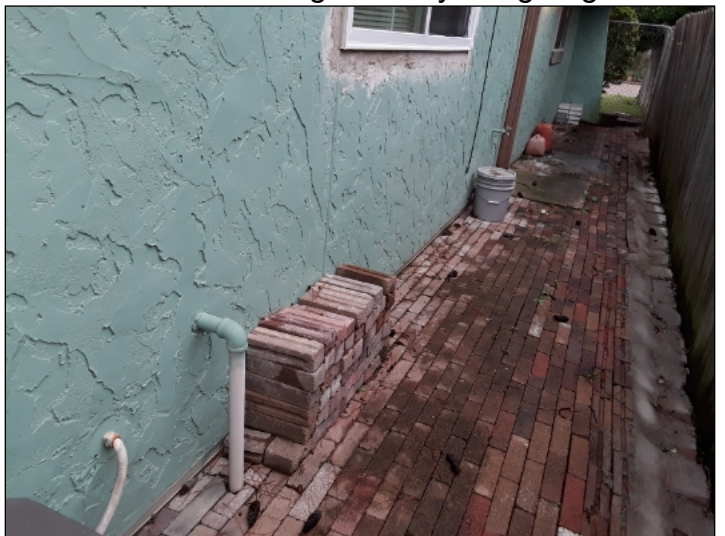
-Wood or other debris is stacked against the house. Recommend all wood or other materials be separated from the structure to help prevent conducive conditions for wood destroying insects.
