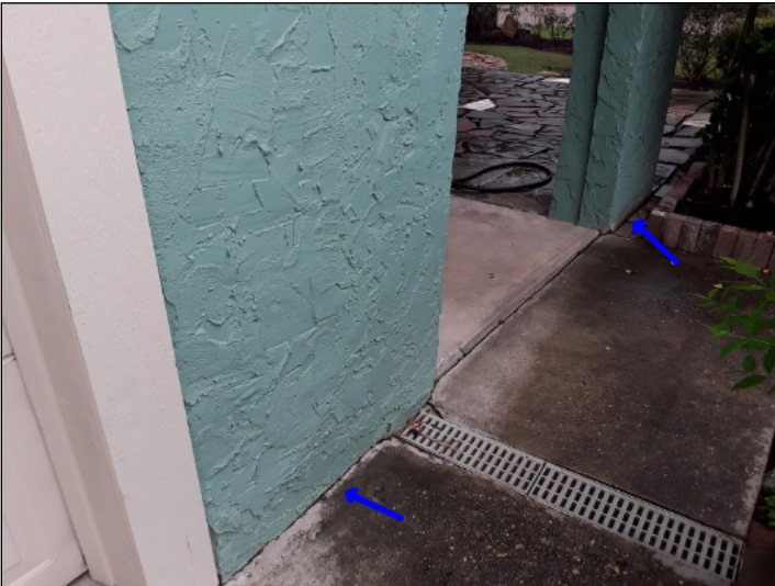
-The soil is too high or footing is too low which does not allow proper exposure of the slab. This can cause conducive conditions to Wood Destroying Insects or water penetration usually if there is improper slope. Mainly at - front
