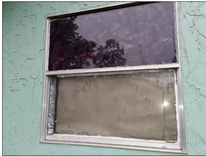
Damaged or incomplete window. Mainly at - rear
