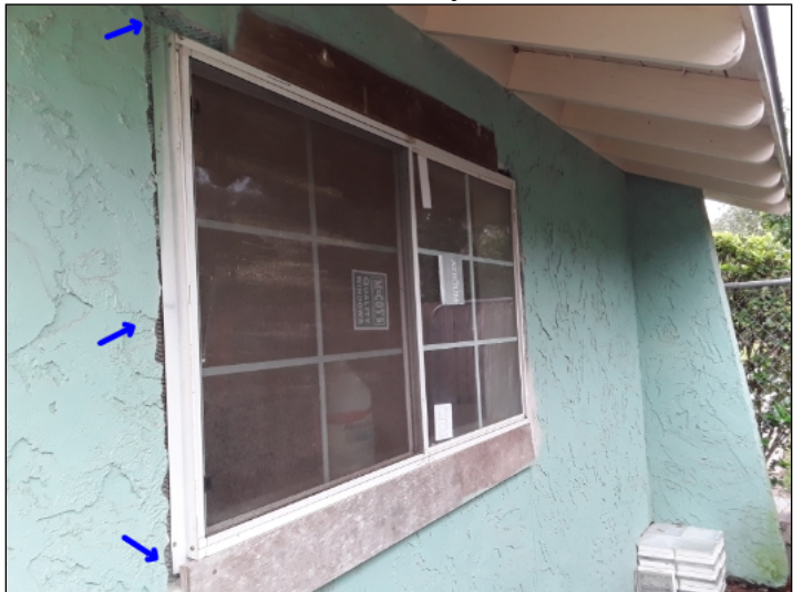
-Stucco is damaged, recommend repairs to help prevent water penetration. Mainly at - left (at garage window)
