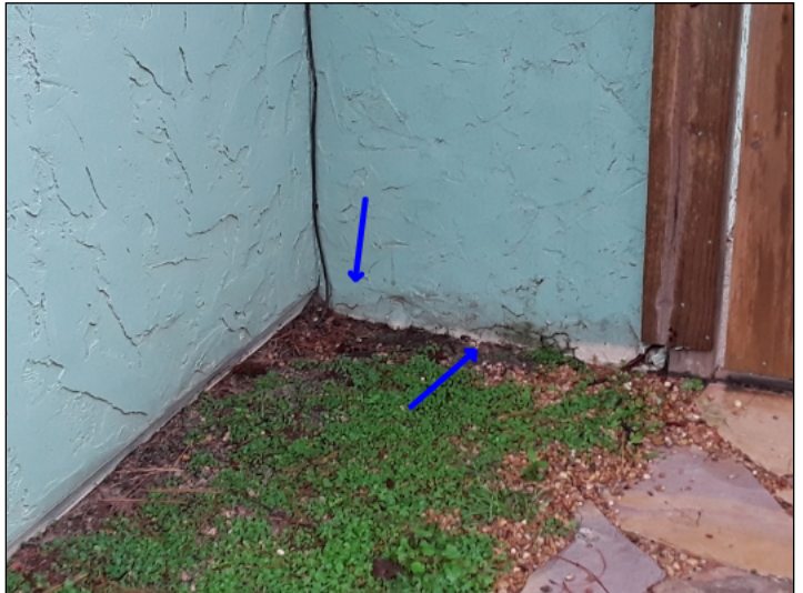
-The soil is too high or footing is too low which does not allow proper exposure of the slab. This can cause conducive conditions to Wood Destroying Insects or water penetration usually if there is improper slope. Mainly at - front
