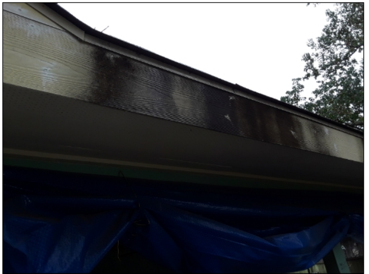
Stains noted at trim.
