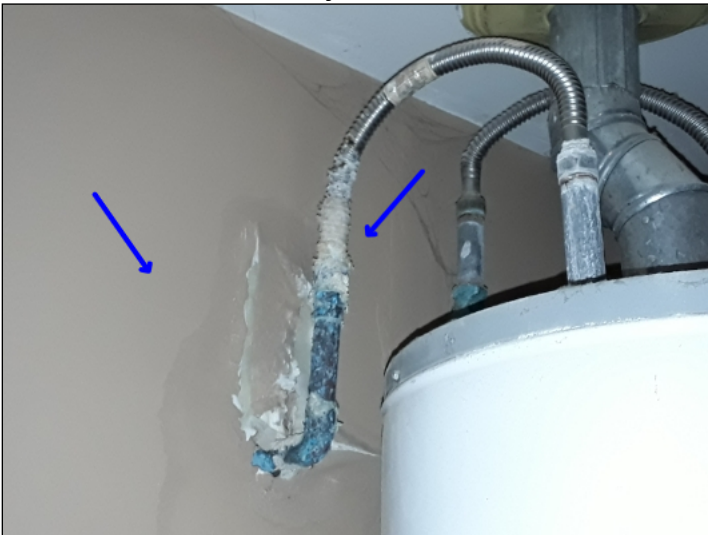
-There are indications of a possible water leak at the water heater connections due to rust/corrosion or deterioration at wall penetration. Recommend a licensed plumber be consulted for further evaluation and/or repairs.
