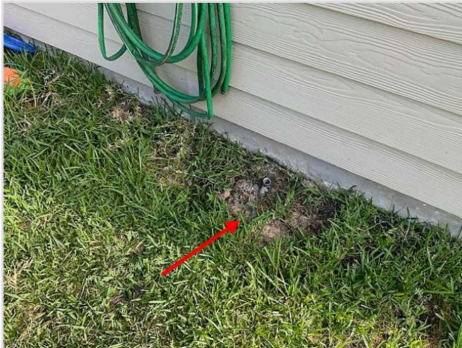
Soil erosion (rear)
