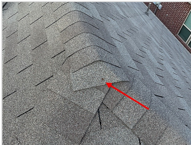
Nail in need of caulk maintenance (front)
