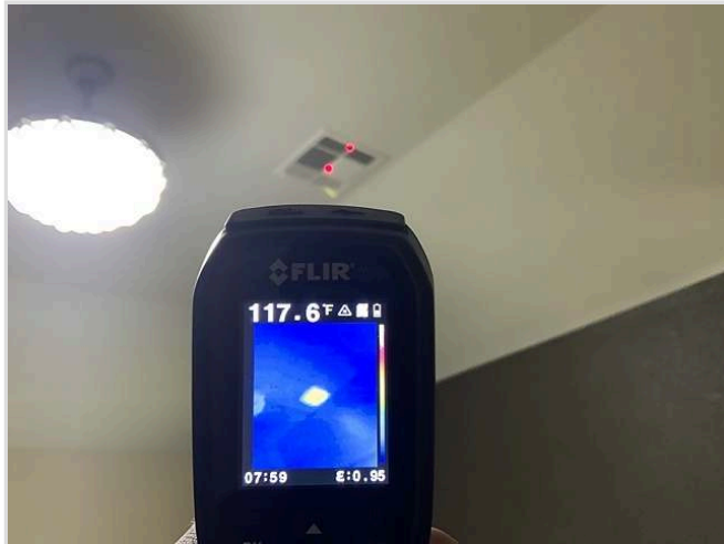
Thermal showing +100 degrees at supply register (master bedroom)
