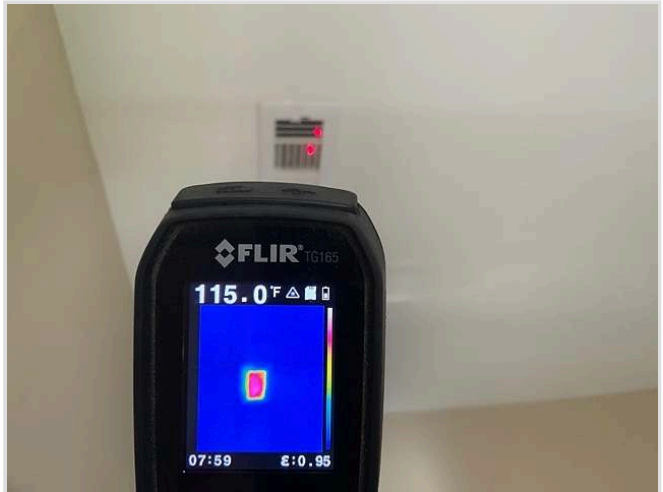
Thermal showing +100 degrees at supply register (master bathroom)
