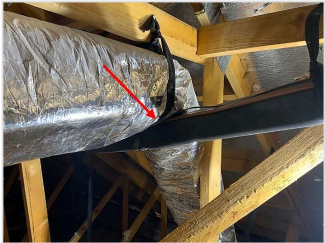
Duct in contact with refrigerant line
