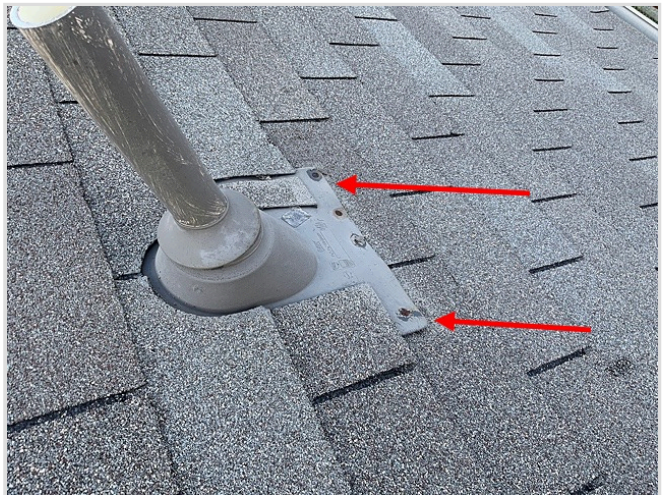
Nails in need of caulk maintenance (right)
