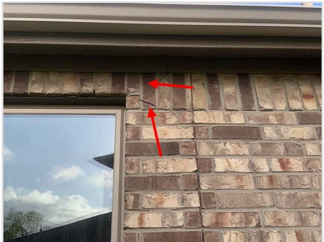
Crack above and adjacent to window opening (left)
