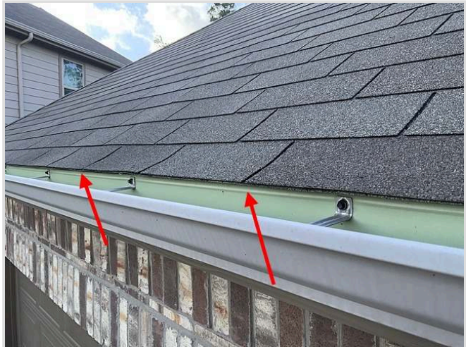
Gutters improperly installed in front of drip edge (front)
