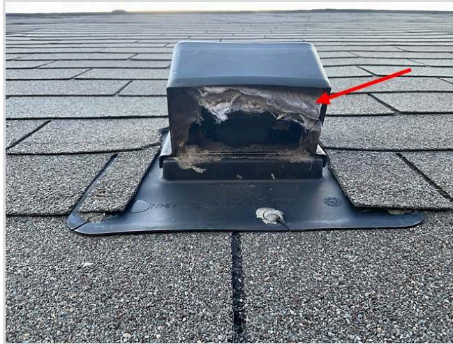
Excessive lint build up (right)
