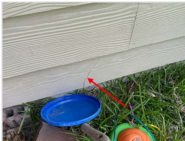
Damaged wall covering (rear)
