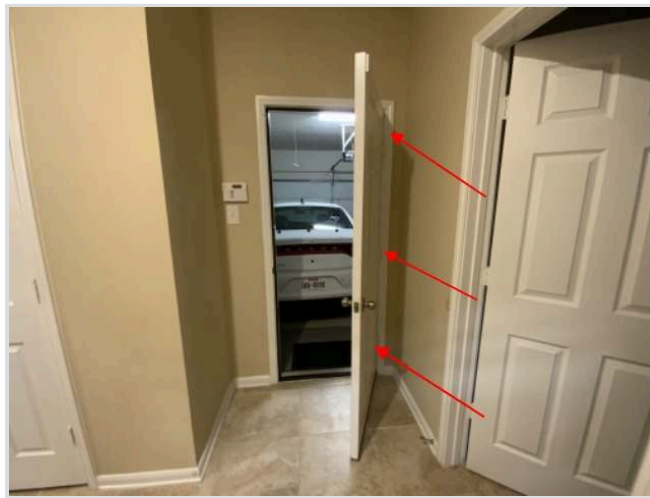
Self closing hinges not installed (garage entry door)
