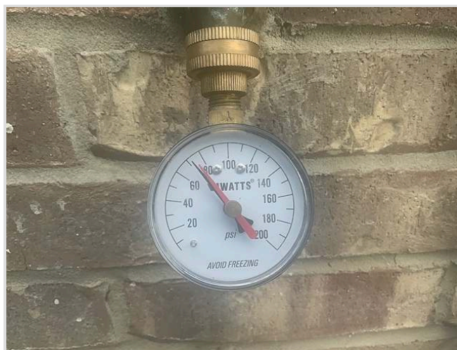
Static water pressure (70-80 psi)
