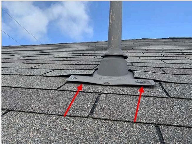
Raised flashing (left)
