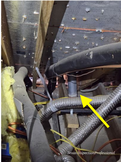
Exhaust vent strap broken for water heater in attic area
