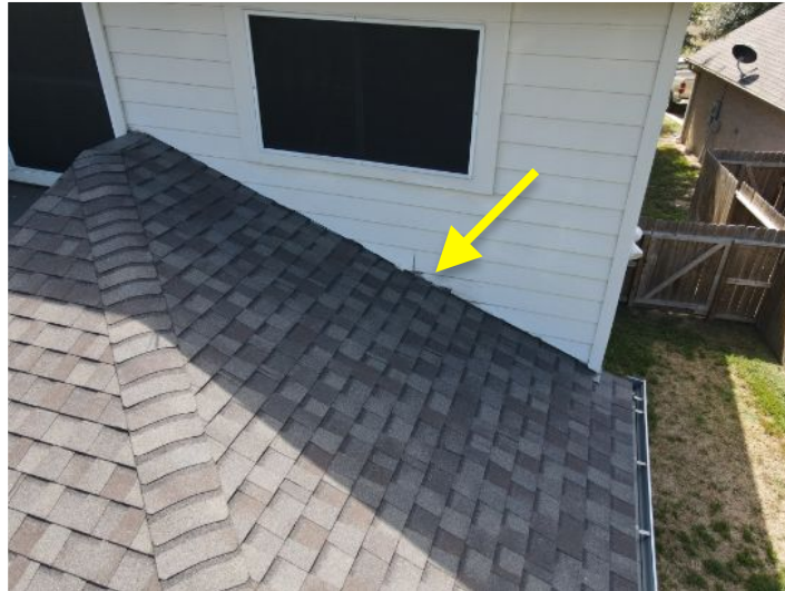
Hardy plank chipped - Rear
