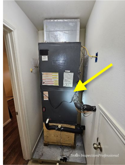
Furnace installed as per standards - upper level office unit - Not operational in heating mode
