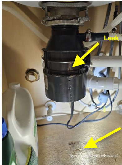
Disposer leaking - Water dripping under the sink
