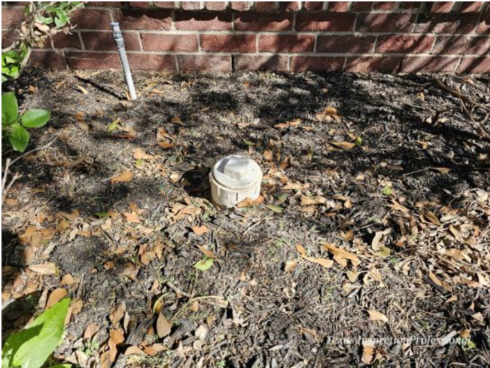
Plumbing main cleanout
