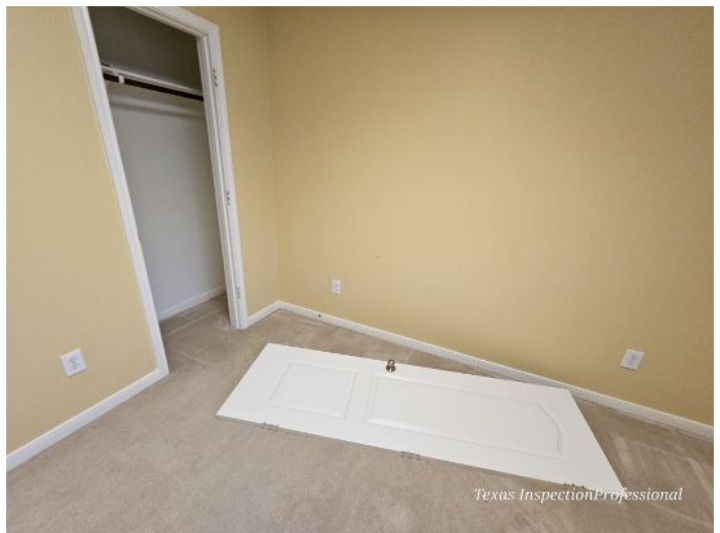
Closet door not installed - Upper level bedroom
