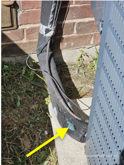
Insulation needs to be replaced
