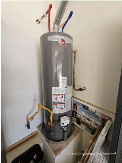
Water heater installed as per standards
