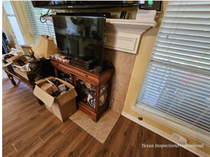
Fireplace blocked - Unable to check
