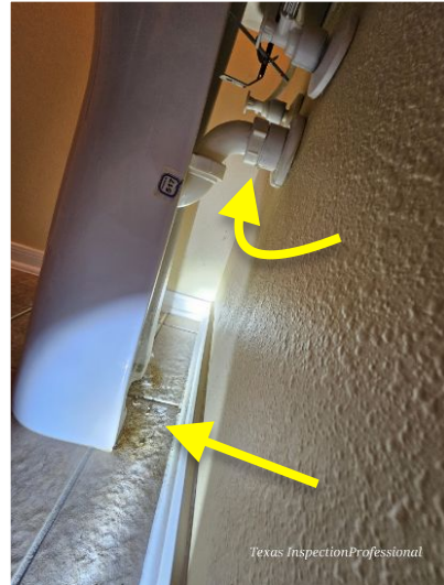
Water leaks under sink - Lower level common bathroom
