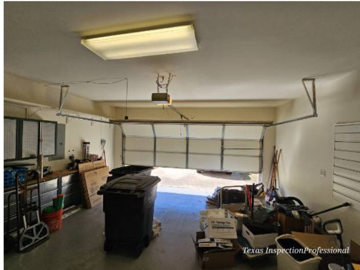
Garage door operator operational
