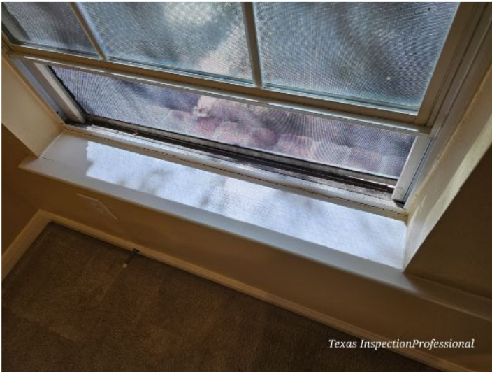
Window frame needs caulking and sealing - Upper level bedroom
