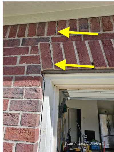
Gap needs to be filled with mortar in between bricks - Front
