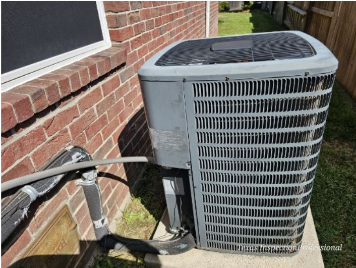
AC compressor -upper AC installed as per standards
