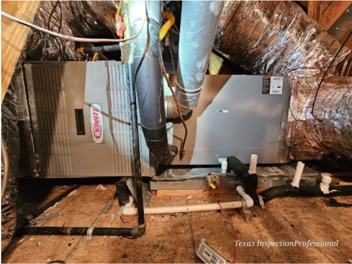
Furnace installed as per standards
