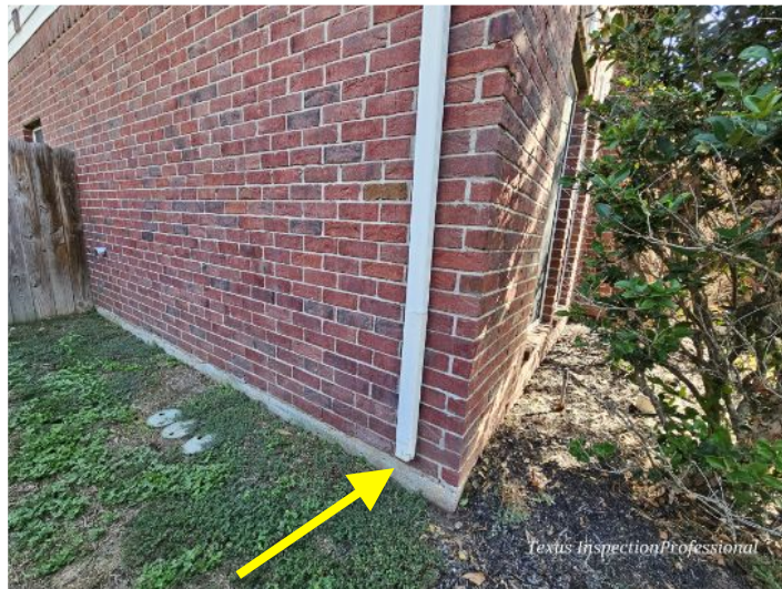
Splash guard not installed -Left side of the house - rain water will splash close to foundation slab
