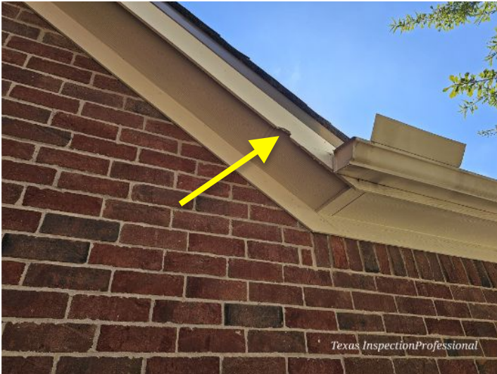
Fascia chipped - Front
