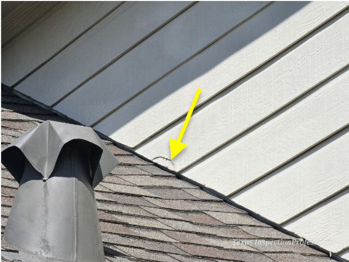
Hardy plank chipped - Front right
