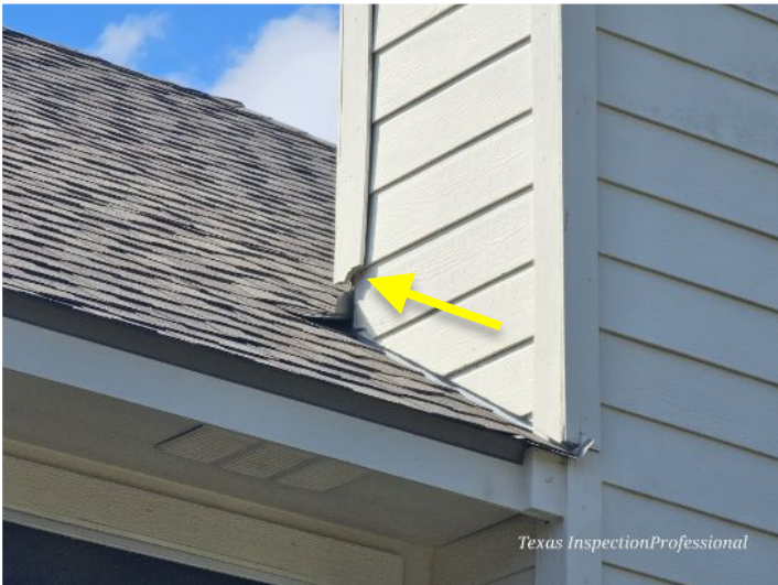
Hardy plank chipped - Rear of the house around chimney
