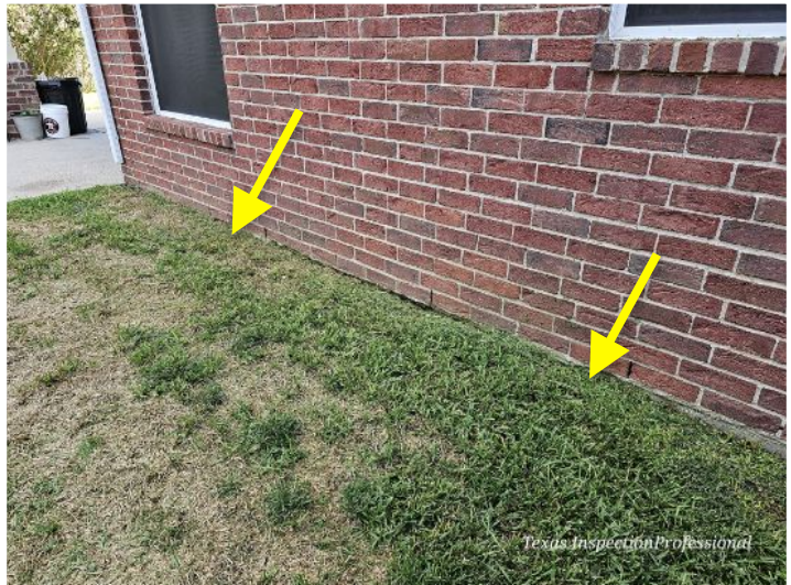
High soil level observed - Left side of the house- Foundation not visible
