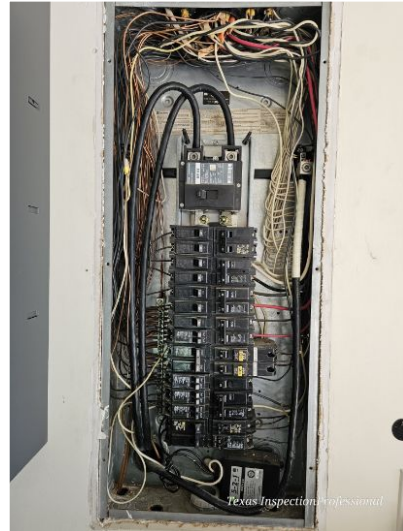
Branch circuit - Copper wiring observed
