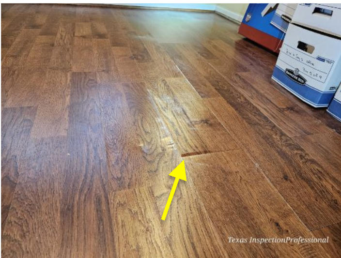
Vinyl floor peeling off/ damaged - Upper level office room
