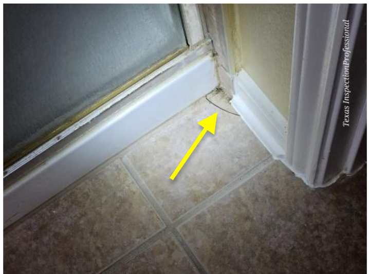
Broken / cracked tile - Master bathroom
