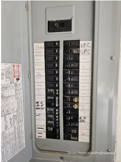
Electrical panel - Main power shutoff
