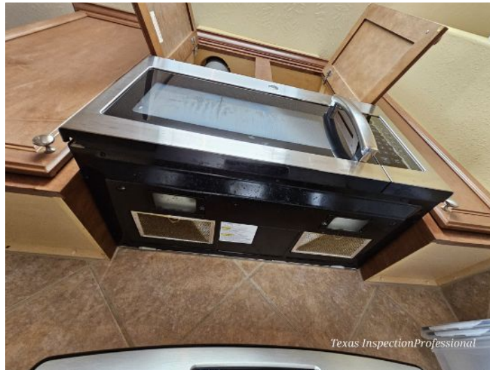
Light does not turn on
