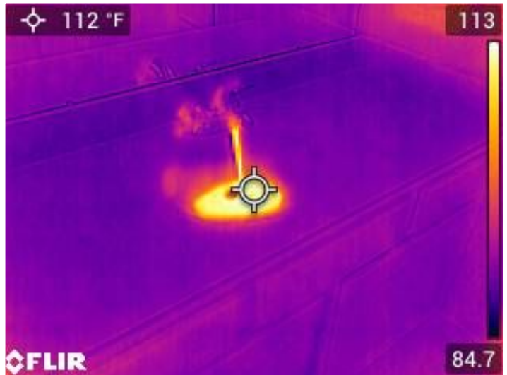
Hot water temperature - optimum - Upper bathroom
