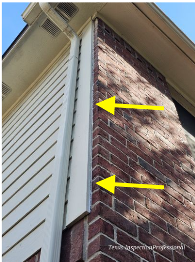
Hardy plank gap needs to be filled - front
