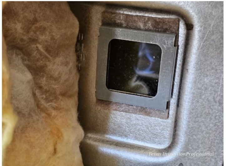
Water heater operational
