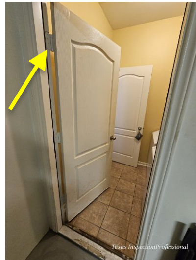
No self-closing hinges found on garage to home door
