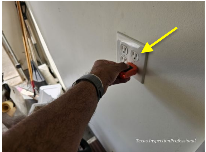
No GFCI (Ground fault circuit interpreter) installed - garage
