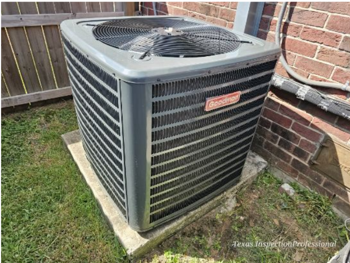
AC compressor installed as per standards
