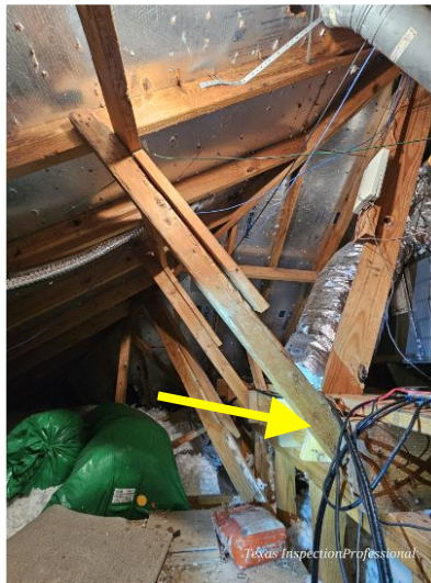
Roof support stud not screwed from bottom
