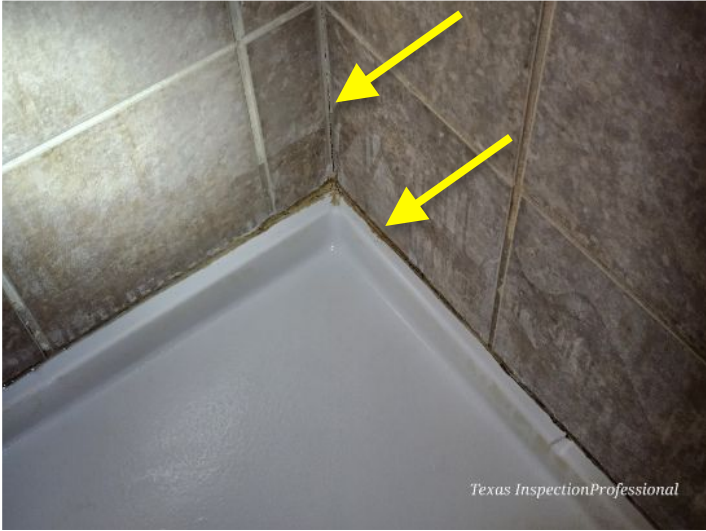
Shower surround needs caulking / sealing
