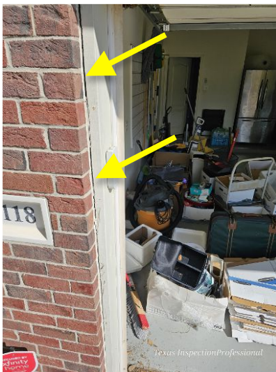
Garage door frame needs re-caulking /sealing
