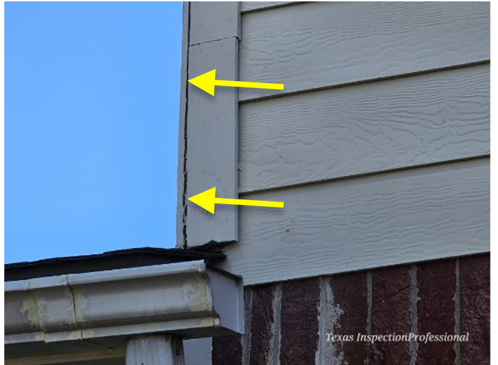
Hardy plank gap needs to be filled
