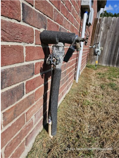
Water main shutoff for the house
