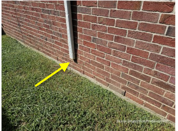
Splash guard not installed -Right side of the house - rain water will splash close to foundation slab
