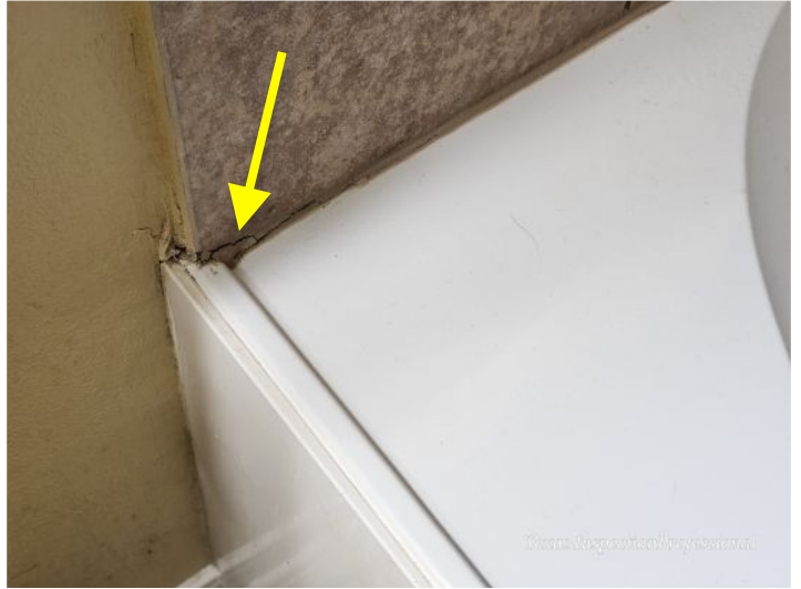
Tub surround needs caulking / sealing
