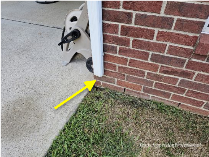
Splash guard not installed -Rear - rain water will splash close to foundation slab
