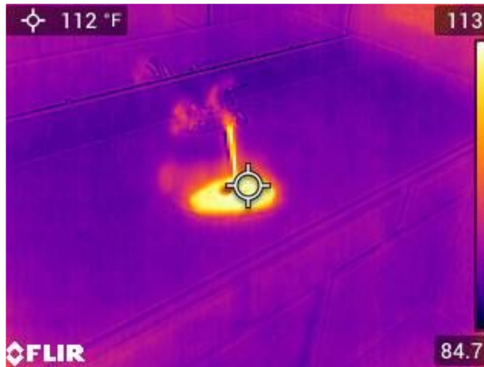
Hot water temperature - optimum - Upper bathroom
