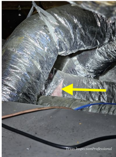
Insulation missing / chewed/ cracked - Hot / cold air leaks
