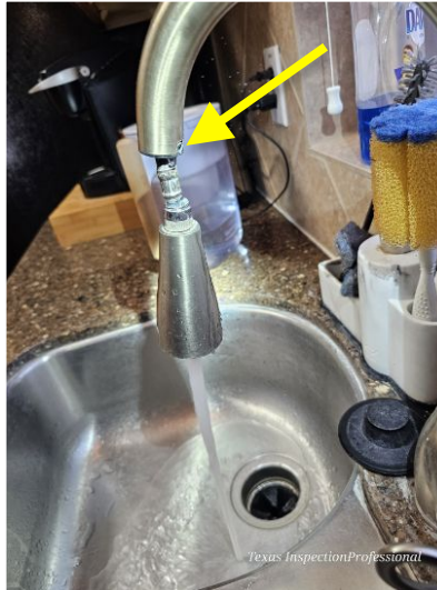
Faucet leaks Kitchen
