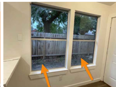
Breakfast area windows stuck shut
