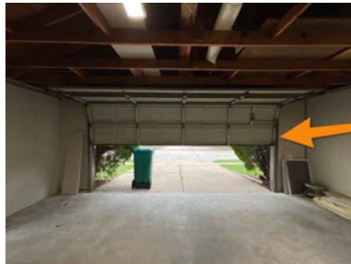
Unable to completely open garage
