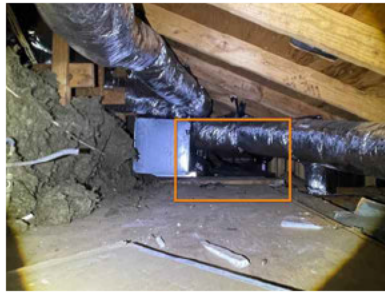
No access, minimum head room requirement not met
