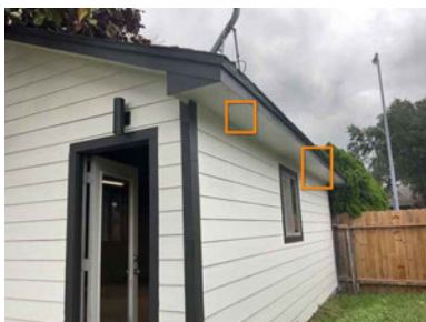
No soffit venting at garage add on
