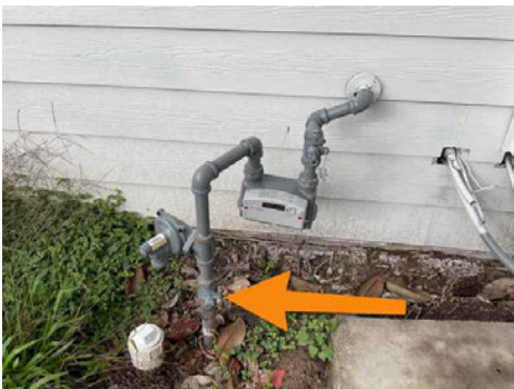
Gas service off
