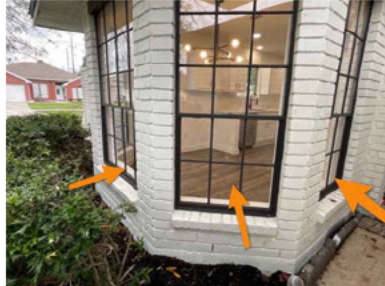
Front windows missing screens
