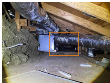
Inadequate head room
