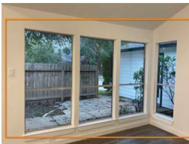
Living Room windows stuck shut
