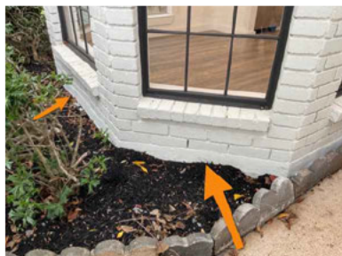
Slab painted multiple locations
