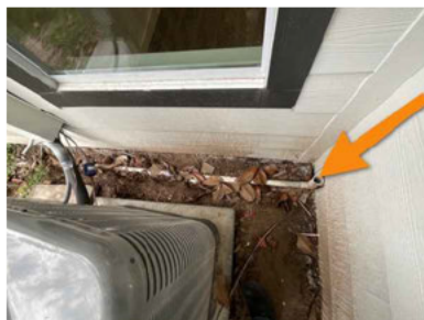
Laundry stand pipe drain at garage
