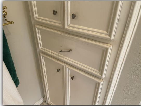
Hairline cracks were found on the interior of the property as evident of settlement.
