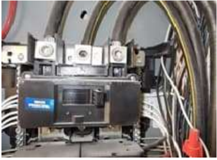
Missing Anti-Oxidant Gel
