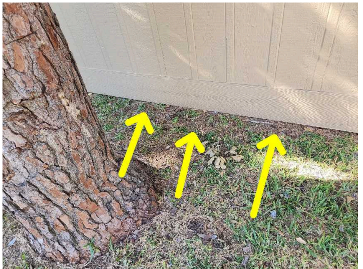
Dirt too high
