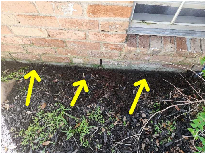
Dirt too high
