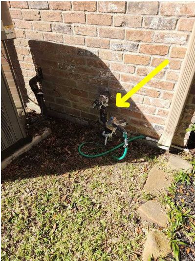
Main water supply valve
