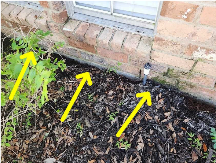
Dirt too high
