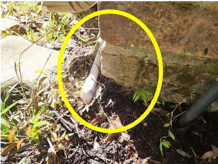
Cracks at corners
