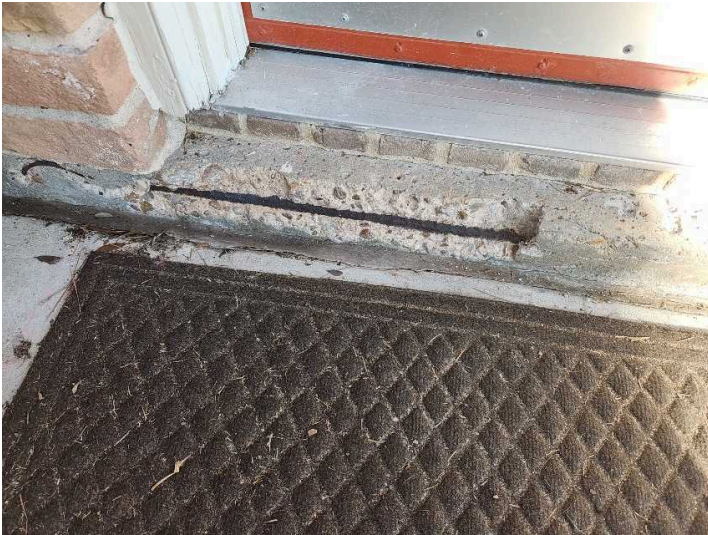
Reinforcement bar exposed
