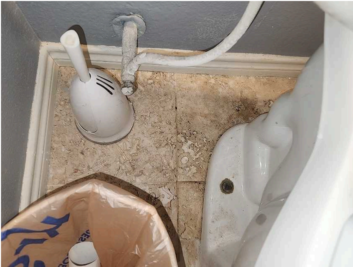
Water leak from tank
