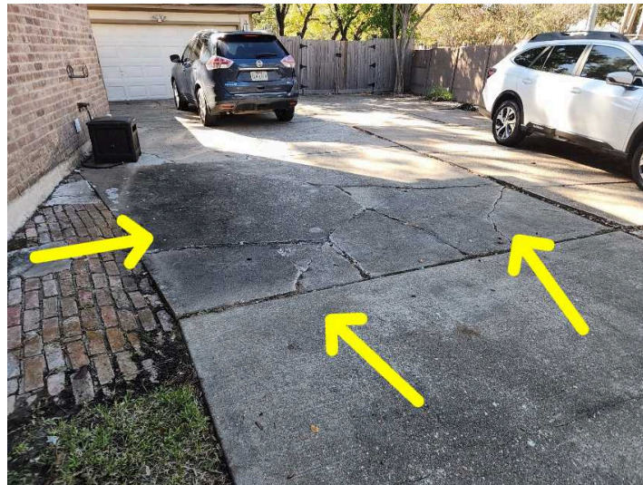
Driveway concrete is cracking and uneven
