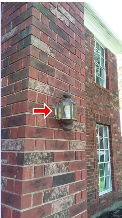
B. Item 15(Picture) entry lights
