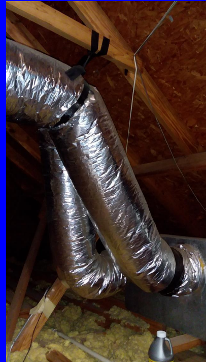
insulated ducts attic
