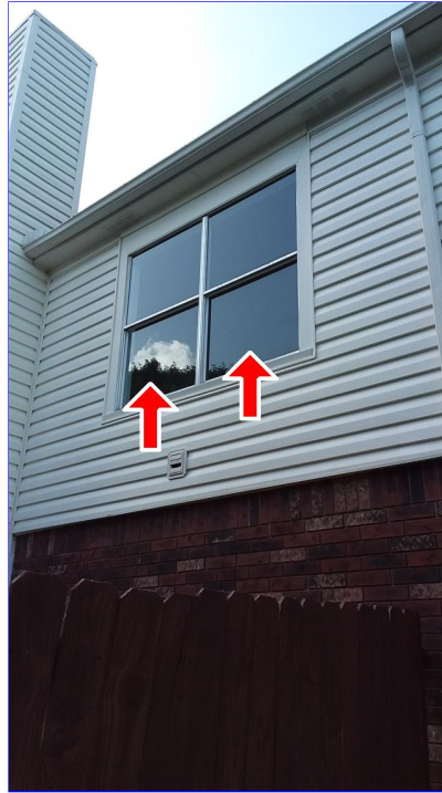
H. Item 7(Picture) multiple windows
