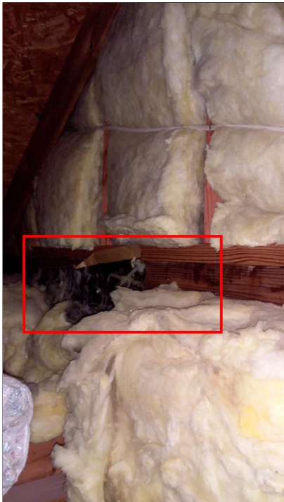
D. Item 5(Picture) garage attic
