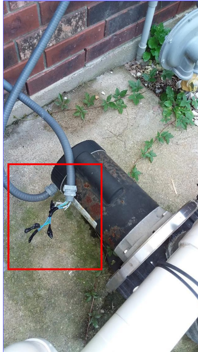
B. Item 7(Picture) not grounded properly
