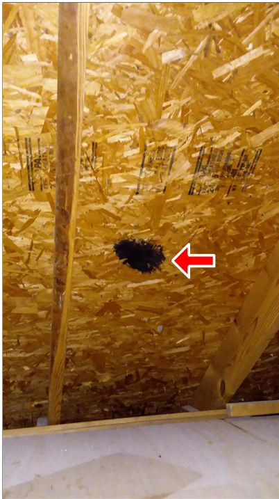
D. Item 8(Picture) garage attic
