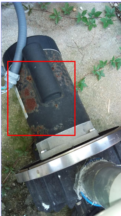
B. Item 8(Picture) equipment rusting
