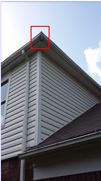
B. Item 10(Picture) multiple areas
