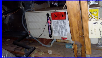
gas furnace attic
