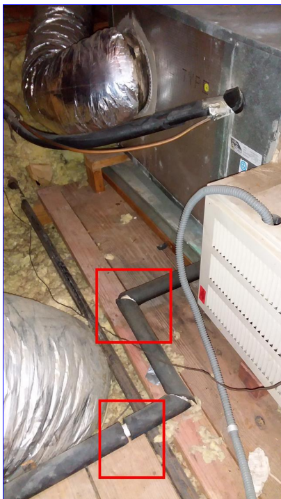
B. Item 8(Picture) rear unit
