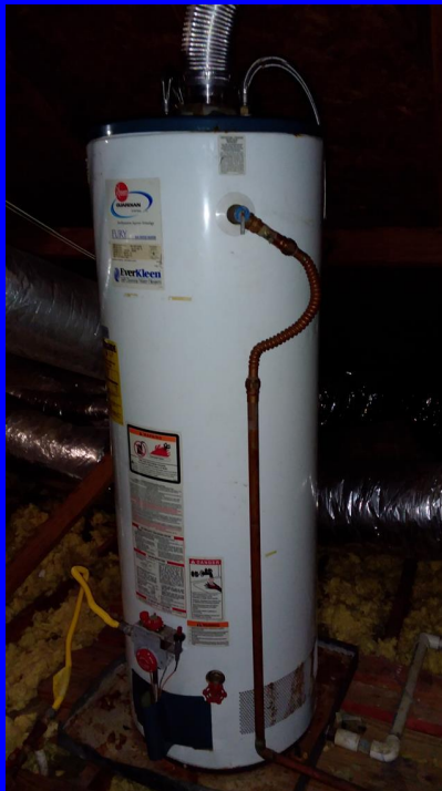
50 gallon water heater attic
