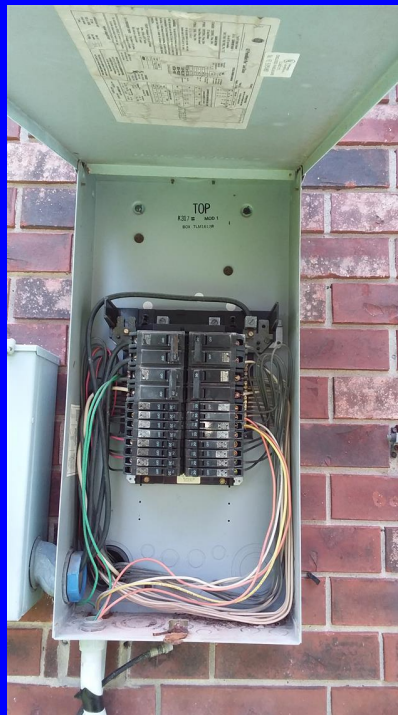
service panel exterior left 100 amp
