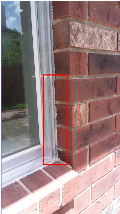
H. Item 9(Picture) multiple windows
