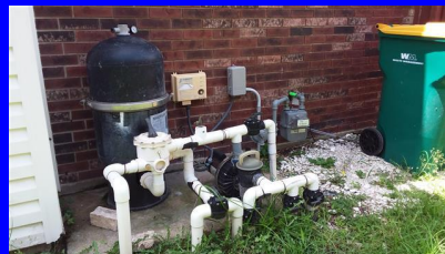
pool pumps rear left
