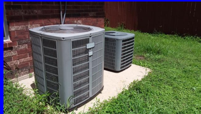
ac units exterior rear
