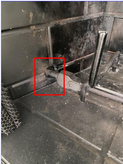
J. Item 3(Picture) seal gap at gas line
