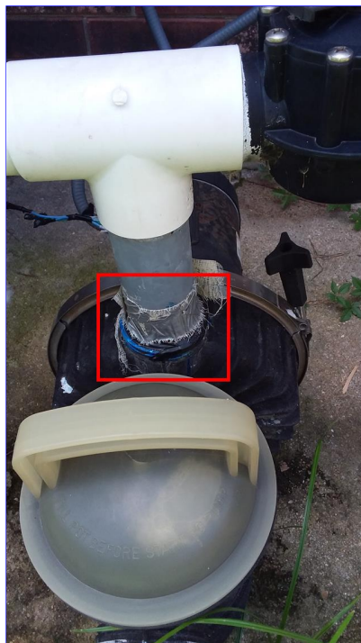
B. Item 9(Picture) pipes repaired inproperly
