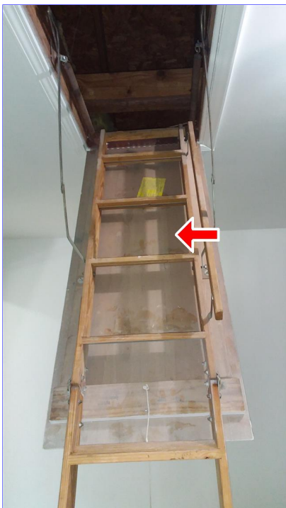
D. Item 2(Picture) garage
