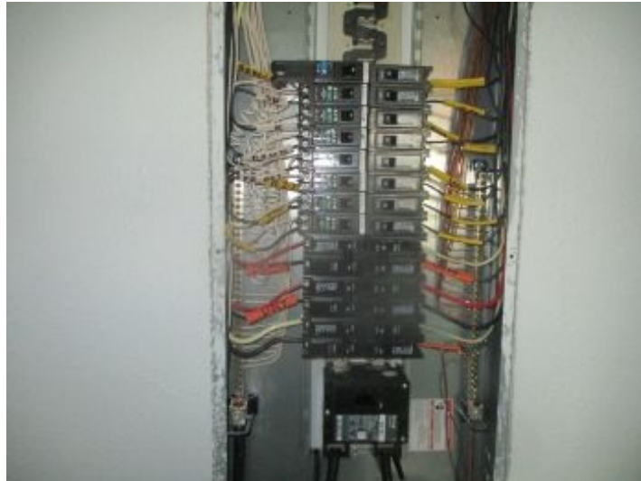
A view of wiring to breakers at interior panel
