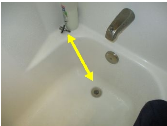
Disconnected drain stop at tun in hallway bathroom.
