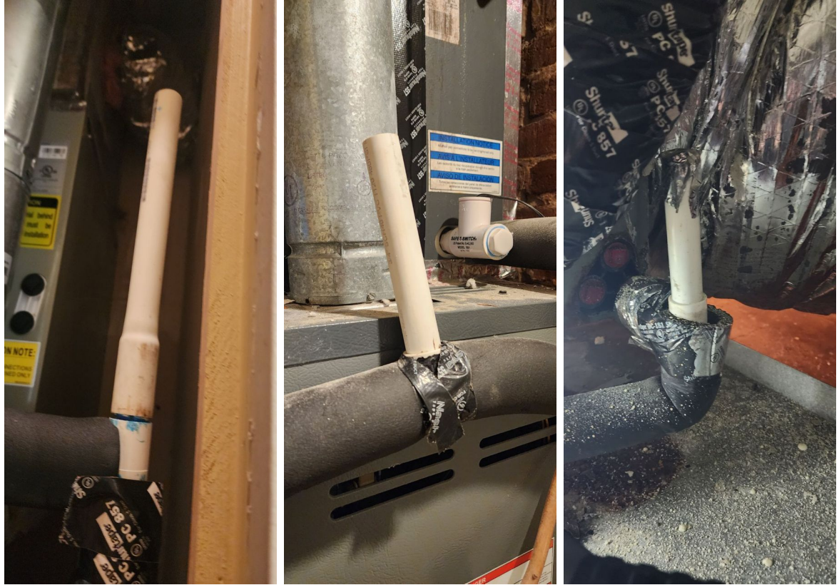
Type of System(s): Central Air Conditioner Brand Exterior for upstairs : Amana
