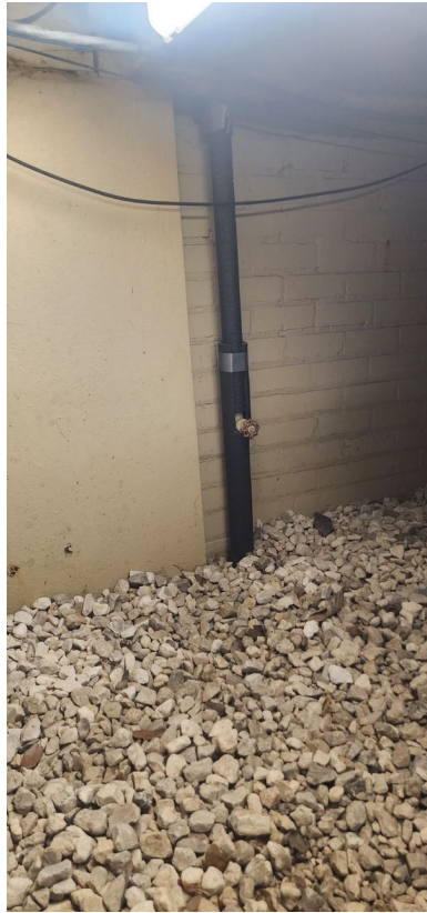
Static Water Pressure Reading: 55 to 60 psi
