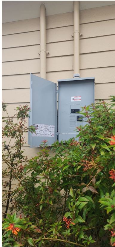
Main Service Panel Amperage: 200 Amp
