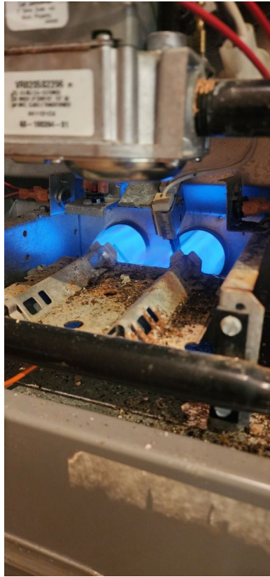
Energy Source for downstairs master bedroom: Natural Gas Brand of furnace downstairs master bedroom: Weather King
