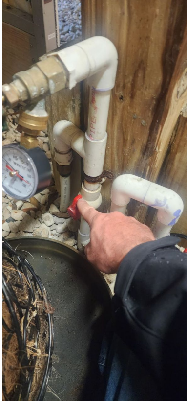
Static Water Pressure Reading: 50 to 55 psi
