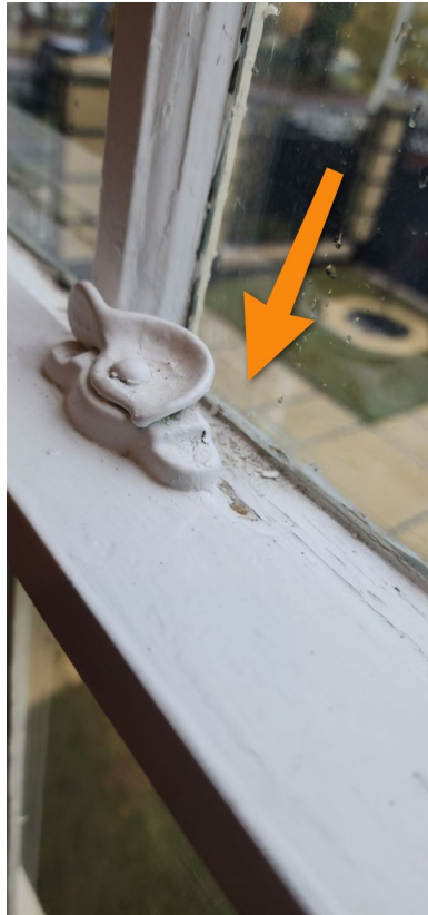
Missing lock at living room Southeast corner
