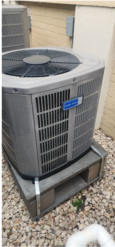
Downstairs master bedroom exterior unit tonnage: 2tons
