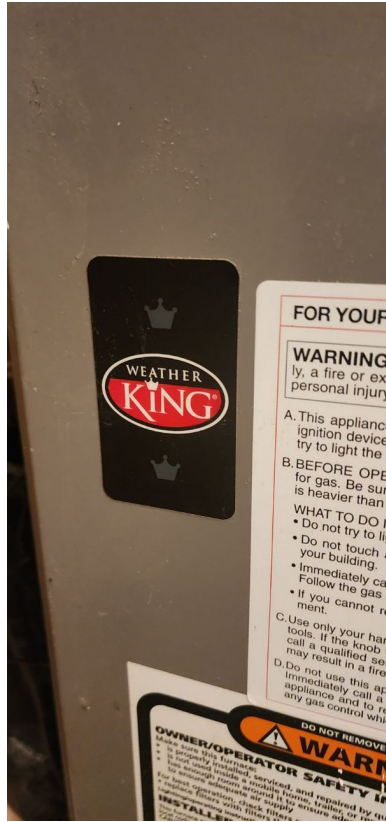
Downstairs master bedroom furnace year of manufacture: 2006
