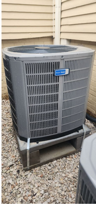
Downstairs exterior unit tonnage: 5 Tons
