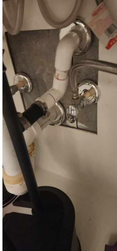
AC drain line under bathroom sink
