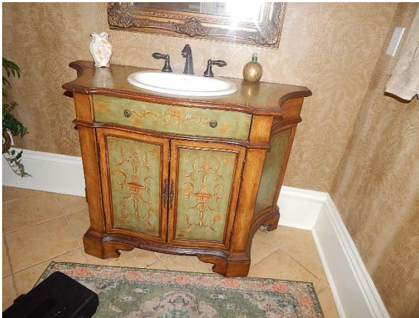
Surface mold growth was observed inside the hall bathroom sink cabinet. A high elevation of airborne Aspergillus/ Penicillium was detected in an air sample taken inside this cabinet.
