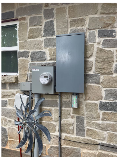
Main electrical disconnect and surge protection.
