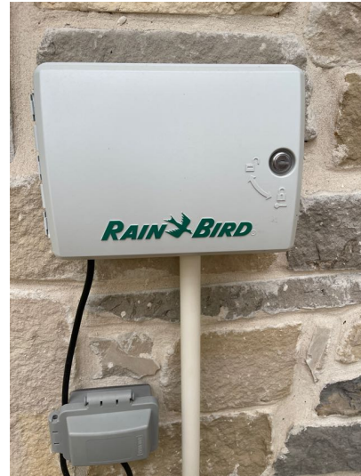
Optional Systems Landscape Irrigation (Sprinkler) Systems
