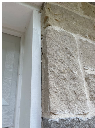
Gaps were noted at some door/windows frame junctions with brick. All exterior wall penetrations, changes of materials and direction should be properly sealed to prevent water and pest intrusion.
