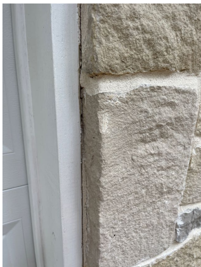
Gaps were noted at some door/windows frame junctions with brick. All exterior wall penetrations, changes of materials and direction should be properly sealed to prevent water and pest intrusion.
