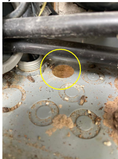
There were missing knockouts in the bottom of the exterior panel and could allow pests to enter.
