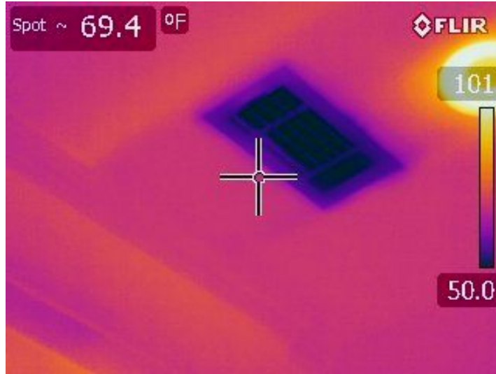
AC was cooling properly. Temperature differential measured 70-50=20 degrees between air supply and registers. Typical range should be 14 to 21 degrees.
