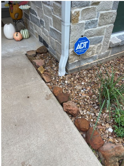
Drainage system was observed with drain grates in the yard and terminations at the curb. Gutter system was installed on the home with gutters down spouts terminating into the drainage system.
