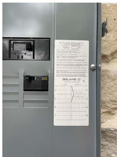
Electrical Systems Service Entrance and Panels
