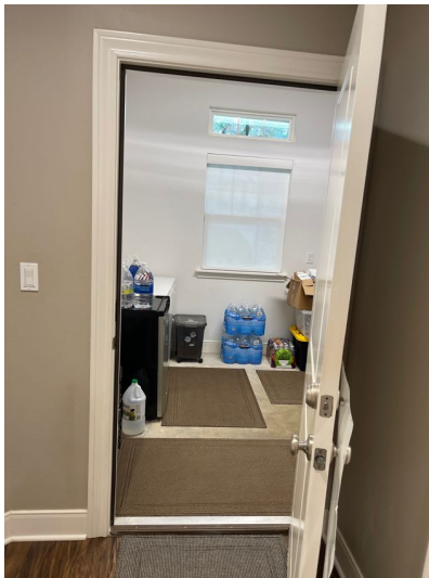
Self closing hardware was missing or ineffective at the garage pedestrian door.
