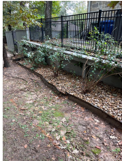
The retaining wall at the back and side of the home had some soft or rotted areas.
