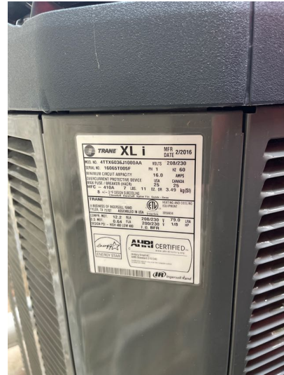
The Condensing unit manufactured by Trane. Unit appeared to be 3 ton, 14 SEER, using 410a refrigerant. Per the manufacturer's label, max amps on breaker should be 25. Per the labeling on the electrical panel, AC was connected to a 25 amp breaker.
