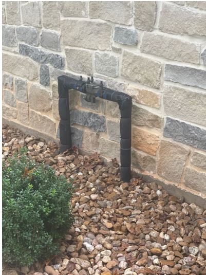
Pressure check valve was observed on the right side of the home and maintains separation of the irrigation system and the potable water supply.
