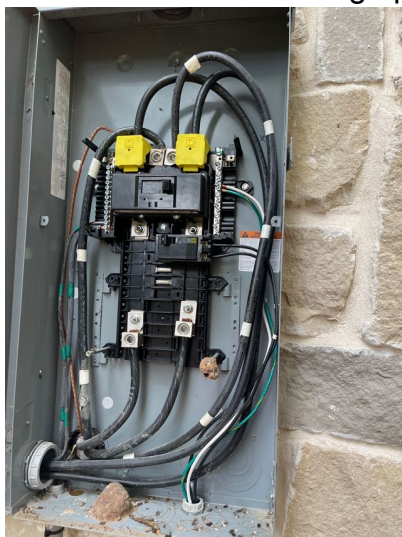
Electrical Systems Service Entrance and Panels
