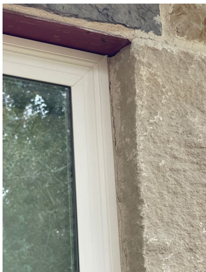
Gaps were noted at some door/windows frame junctions with brick. All exterior wall penetrations, changes of materials and direction should be properly sealed to prevent water and pest intrusion.
