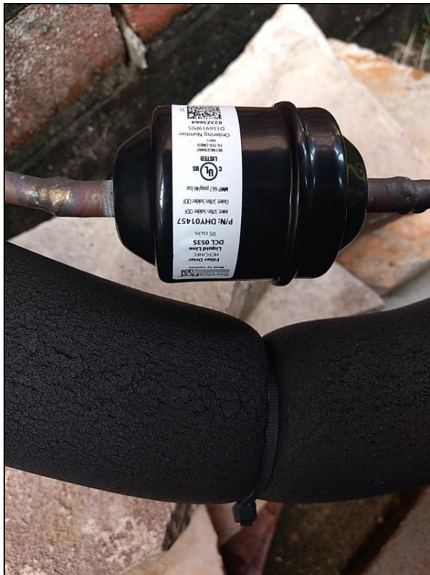
Liquid line dryer
