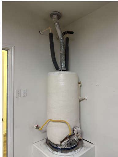
Photo(s) of 2nd water heater: None
