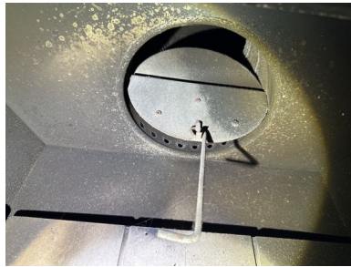
Photo(s) of gas valve:
