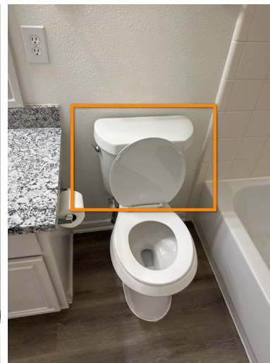
2nd Floor Bathroom tank
