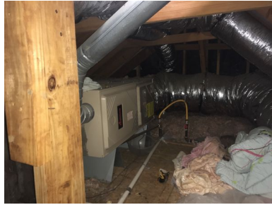
General Photos of HVAC Equipment:
