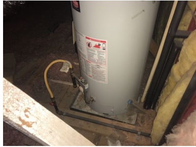
General Photos of Water Heating Equipment:
