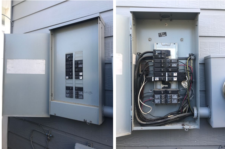
General Infrared Photos of Distribution Panel(s):
