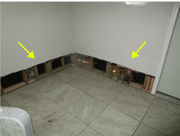
utility room partially gutted
