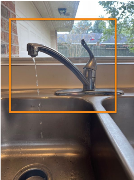
Kitchen sink (no pressure fittings are in open position)
