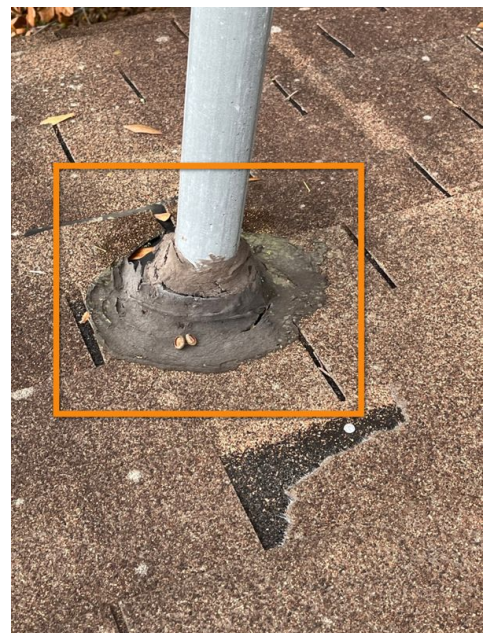
Mast pole at roof
