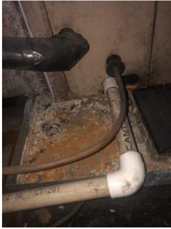
Insulate primary drain line per code. Install secondary drain pan and Inline safety float switches to prevent the coil pan from overflowing if both AC drains are clogged. A float switch detects water backup and turns off the unit before the pan can overflow and spill out onto your attic floor and through the ceiling. Clear AC drain line.
