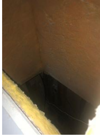
Dust present in the return plenum.
