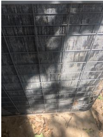
Smashed condenser coil fins. This will prevent the AC from working efficiently.
