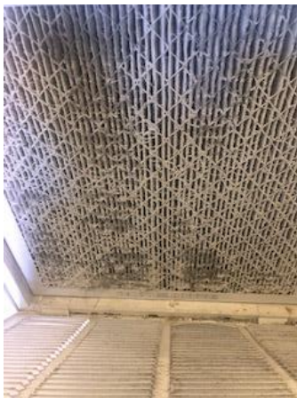
Replace dirty filter.
