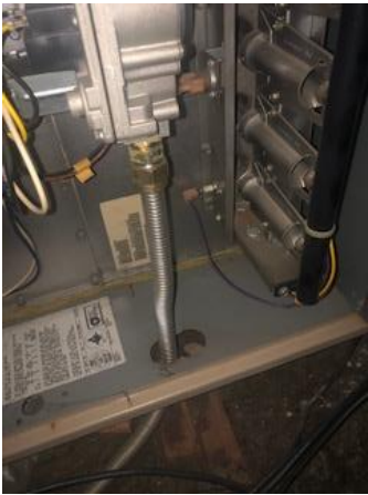
Upgrade furnace gas line to rigid pipe per code,
