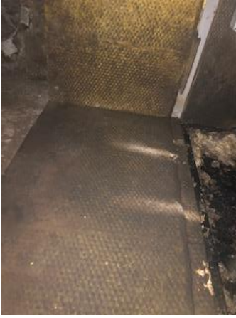
Black growth present in the supply plenum.
