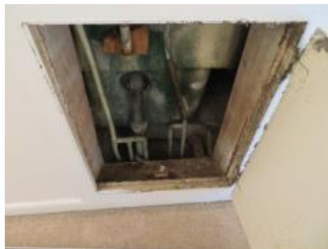
PS=Previous Subterranean Termites
