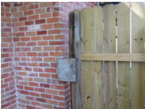
R=Wooden Fence in Contact w/Structure
