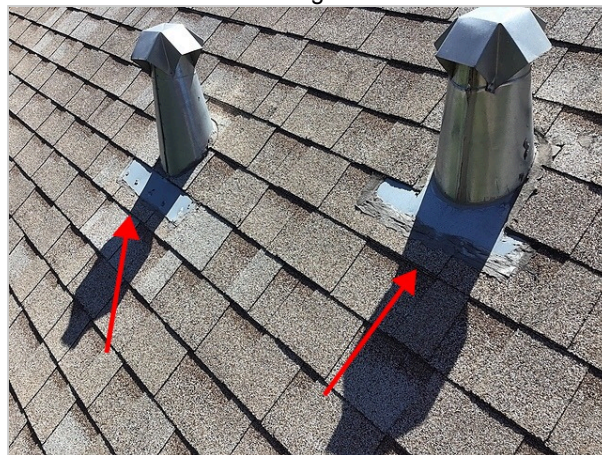
Caulked at the apron
