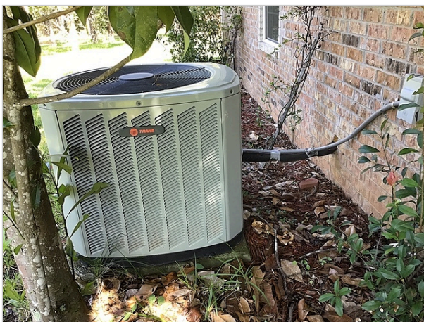
Outside AC unit
