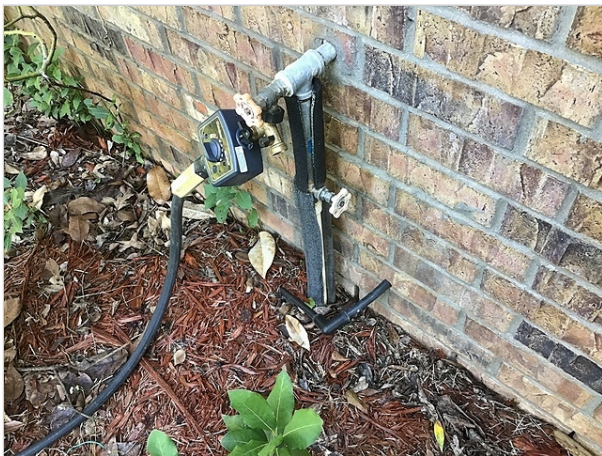
Main water supply valve
