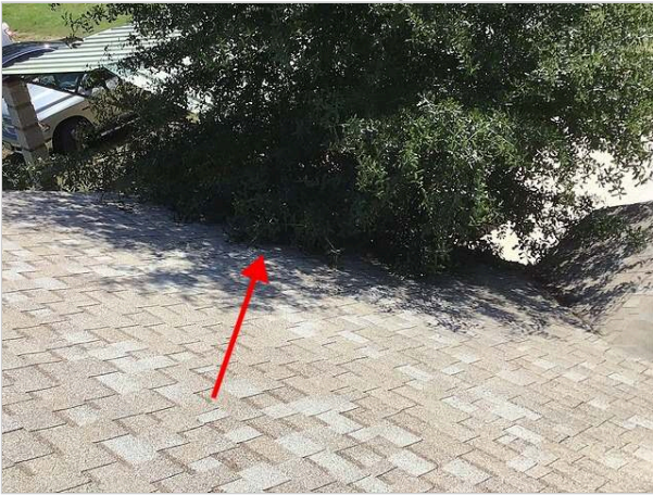
Tree in contact with the roof
