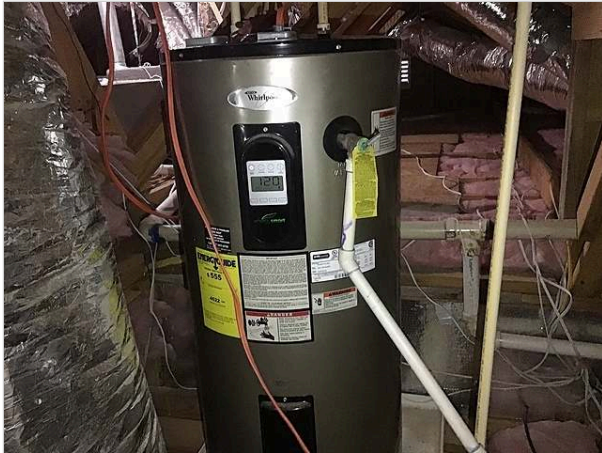
Unit in attic
