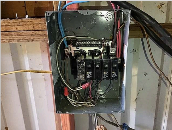
2. Sub-panel cover removed for inspection
