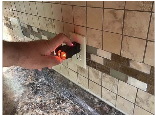
Tester showing not GFCI protected (kitchen)
