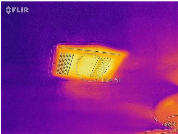
Thermal showing 100+ degrees of temperature output (downstairs guest bedroom)
