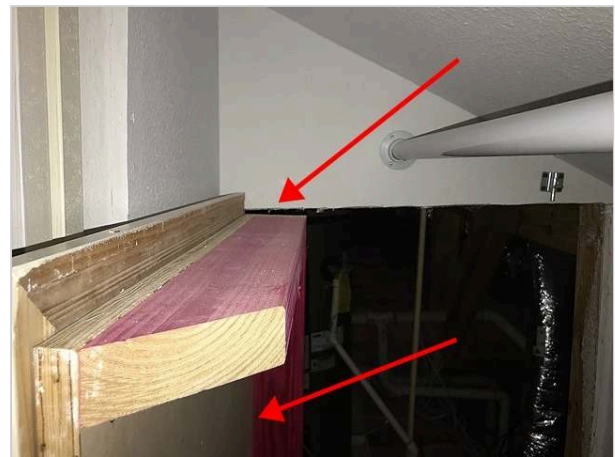
Not insulated/no weather stripping (attic water heater access)
