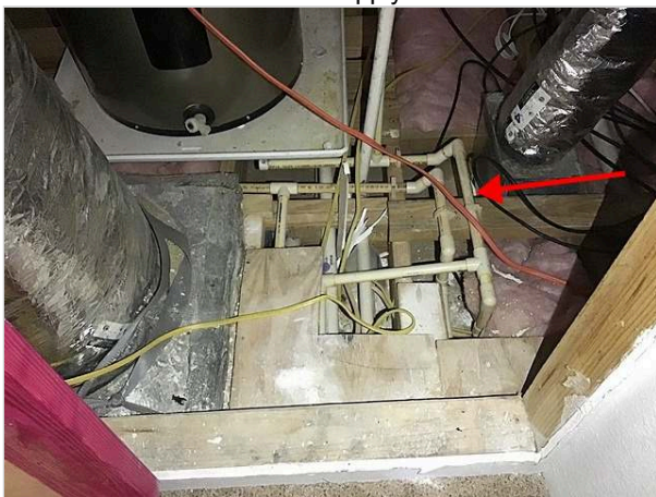
Not properly insulated
