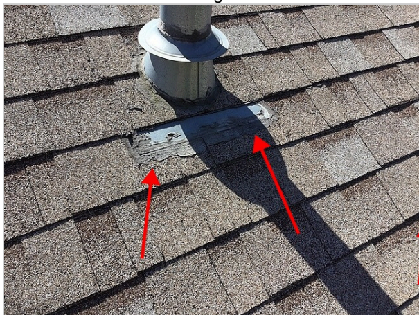
Caulked at the apron
