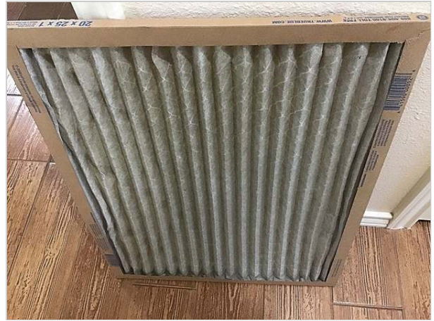
Needed to be replaced
