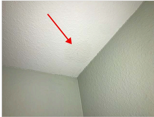
Staining (master bedroom)
