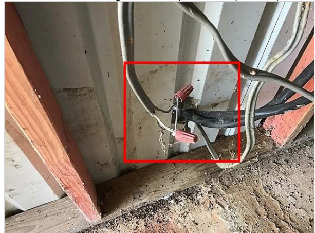
Not in a junction box (well house)
