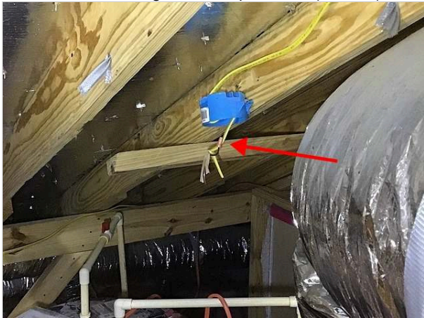
Not in junction box (attic)
