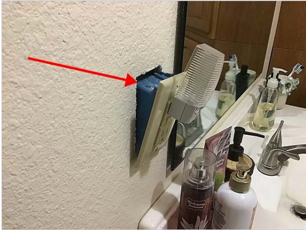
Loose (hall bathroom)
