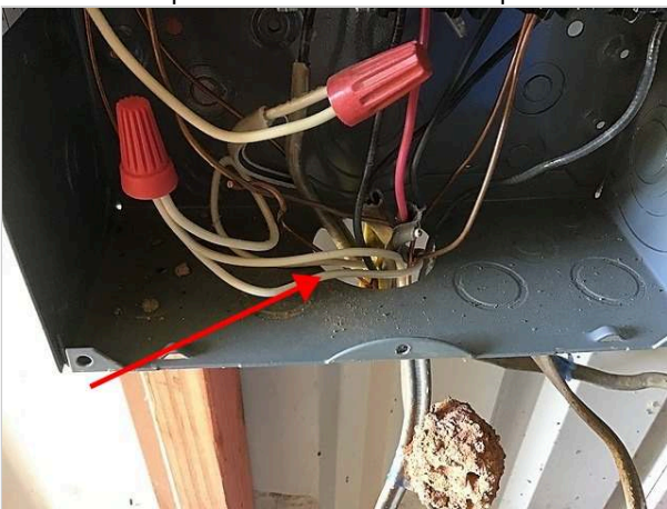
Not protected from abrasion (no grommet/bushing)
