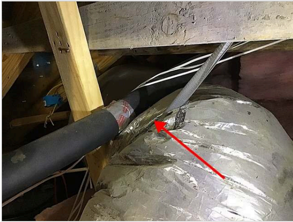
In contact with the refrigerant line
