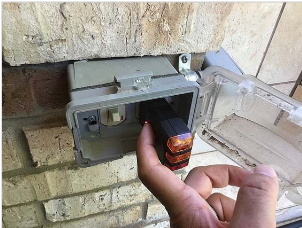
Tester showing not GFCI protected (exterior)
