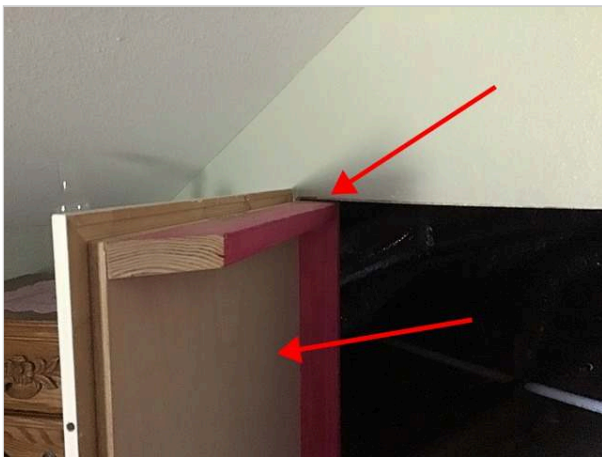
Not insulated/no weather stripping (attic HVAC access)
