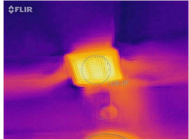
Thermal showing 100+ degrees of temperature output (kitchen)
