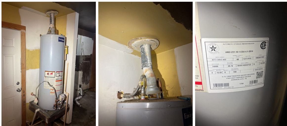
Photo(s) of 1st water heater: Natural Gas
