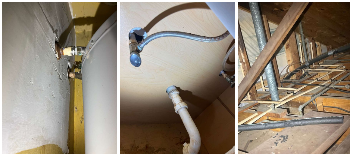
Water shut off location: Left of Structure
