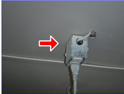
B. Item 2 (Picture) Missing plug cover storage room
