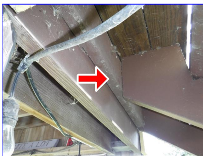
I. Item 2 (Picture) Missing pressure blocking / hangers
