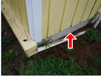
E. Item 2 (Picture) Wood deterioration along bottom rear
