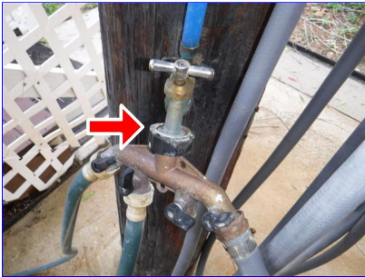
A. Item 3 (Picture) Missing anti siphon devices on outside hose bibs
