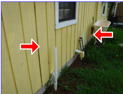
B. Item 2 (Picture) 2 vent pipes rear terminate within 3 feet of operational window
