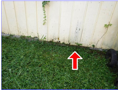
E. Item 4 (Picture) Wood deterioration along bottom rear
