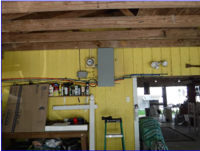
A. Item 3 (Picture) Mounted too high
