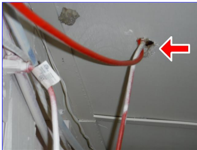
B. Item 3 (Picture) Extension cord run through ceiling storage room
