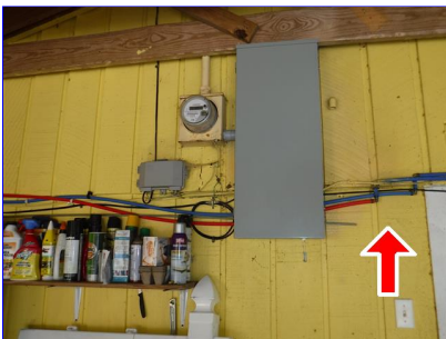
A. Item 7 (Picture) Un-insulated water lines left side
