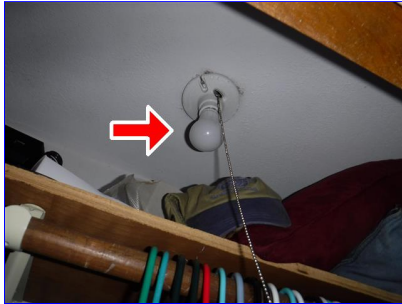
B. Item 1 (Picture) Un-covered light fixtures in bedroom closet
