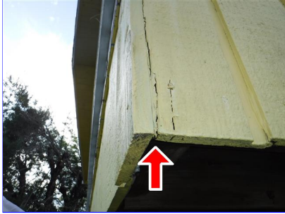
E. Item 1 (Picture) Wood deterioration right front corner
