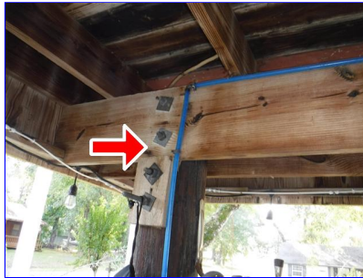
A. Item 4 (Picture) Un-insulated water lines in crawlspace
