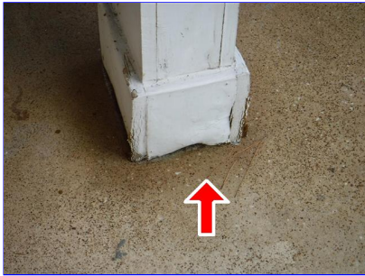
E. Item 3 (Picture) Wood deterioration post trim
