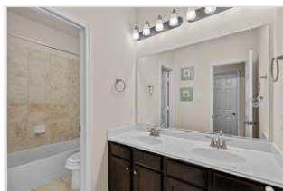
Bath #2 is located upstairs in the hall next door to the media room. It provides dual sinks, a large wall mirror, and private toilet area. The cabinets have some damage to the stain.
