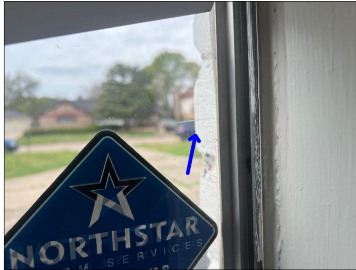
Cracked windowpane(s) were noted. Mainly at - front middle bedroom
