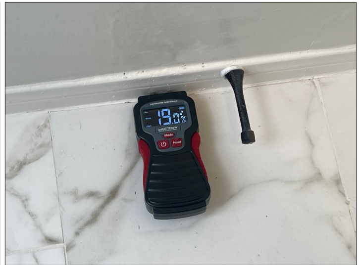
Checked water stain with a moisture meter and found it to be at a high moisture level. Unable to determine condition of the underlying materials. Mainly at - behind leaking primary tub spout
