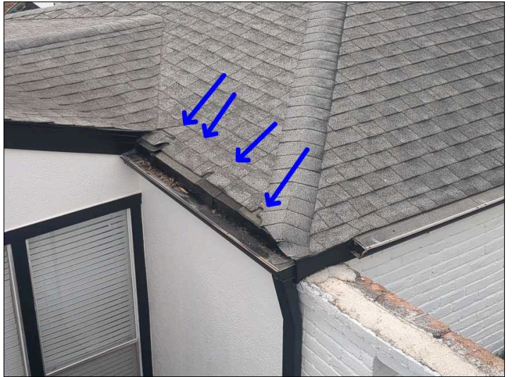
There are damaged or missing shingles on the roof, recommend repairs or replacement of damaged shingles.
