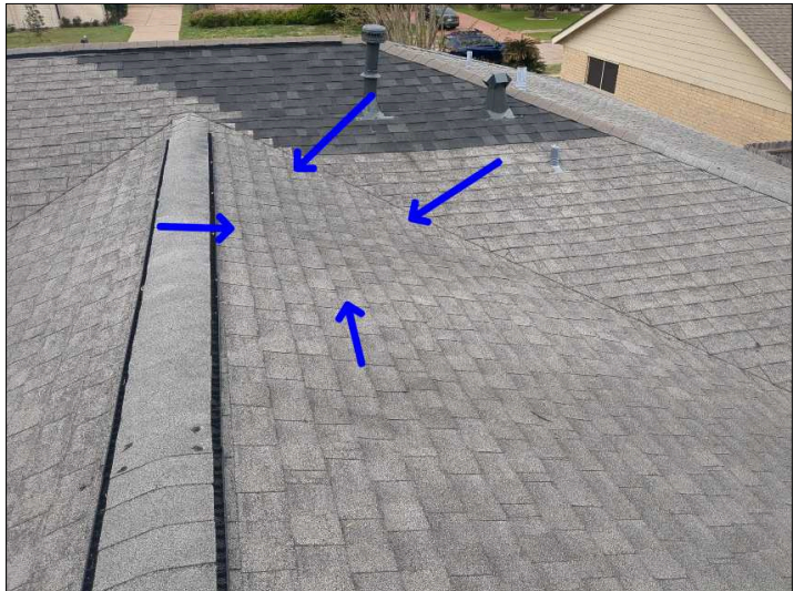
There are indications that there is deteriorated decking under the roof covering due to a soft spot under the shingles, recommend contacting a roof specialist to evaluate and repair as needed and check entire roof for other issues that may be of concern.
