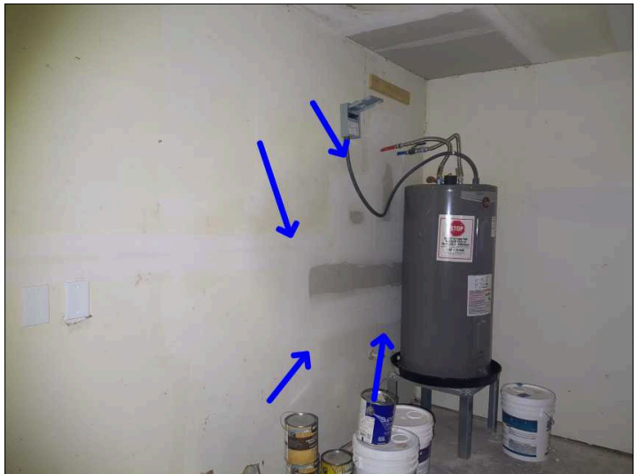
There is evidence of previous patch work and or painting on the interior finishes. Recommend contacting homeowner for more information. Mainly at - garage
