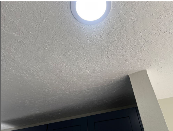
There is evidence of previous patch work and or painting on the interior finishes. This condition may limit the inspector's visual observations and ability to render accurate opinions as to the performance of the structure. Recommend contacting homeowner for more information. Mainly at - kitchen
