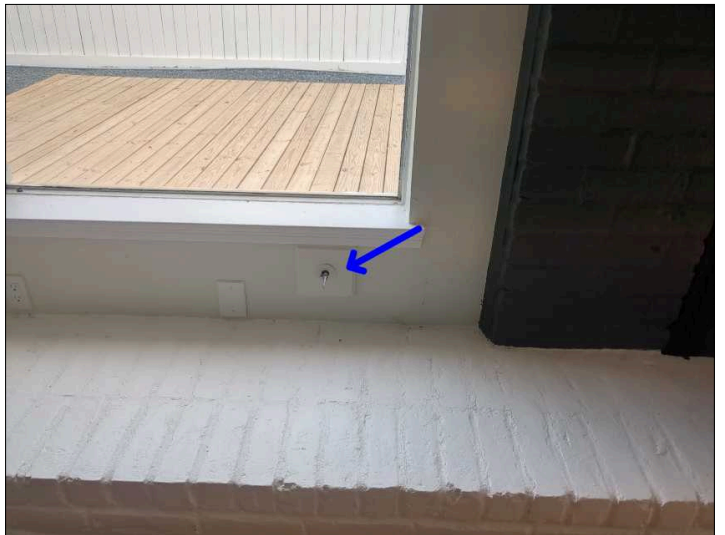
Overview of fireplace gas shut off valve.
