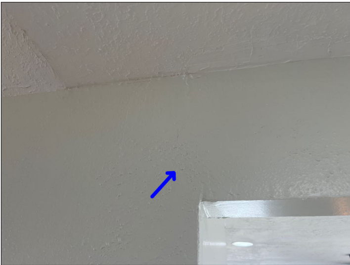
Settlement cracks were noted in the drywall. Mainly at - front entry
