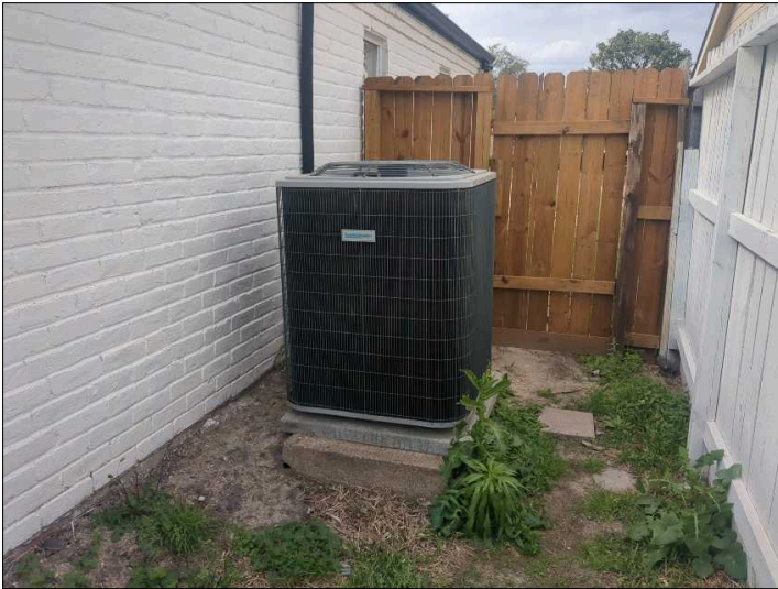
Overview of A/C Condenser
