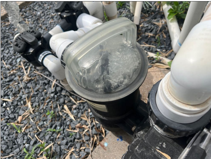
The pool equipment is sucking air, recommend sealing by applying grease to o-ring seals on the filter and strainers.
