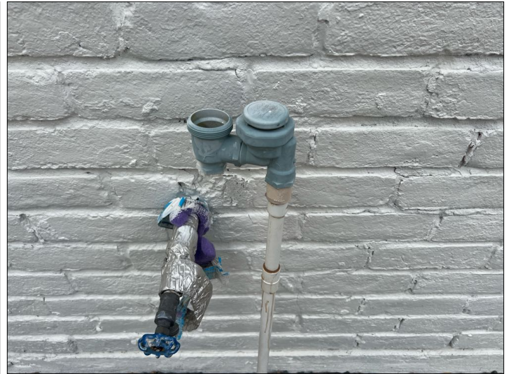
The swimming pool fill valve is disconnected and not properly equipped with a vacuum breaker.
