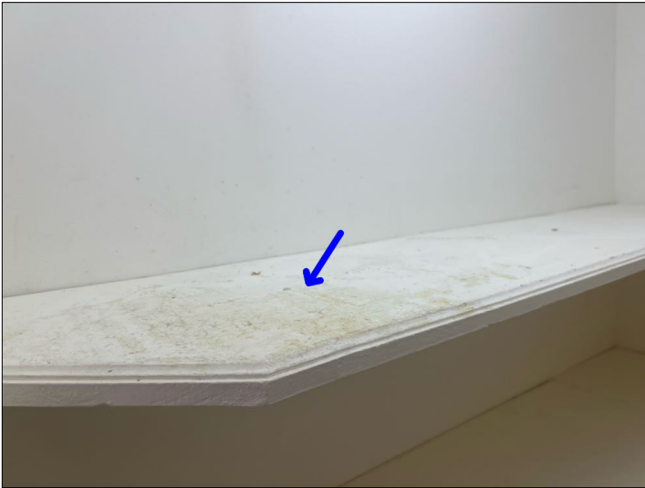
Mold like stains are present. Recommend contacting our office to schedule an evaluation and mold testing to determine the type of mold and identify the source of contamination. Mainly at - pantry
