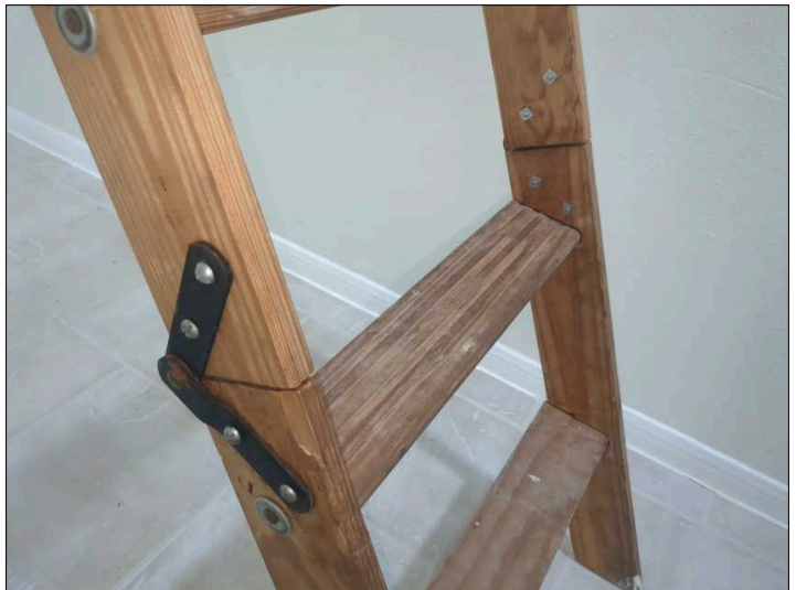
Attic stairway not cut properly to the floor, recommend cutting ladder so the ladder is a straight line when in the down position, otherwise it will put undue stress at the hinge and can cause ladder to fail.
