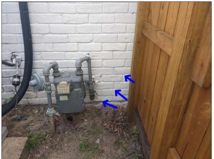
Settlement cracks were noted in the brickwork. Mainly at - left side rear
