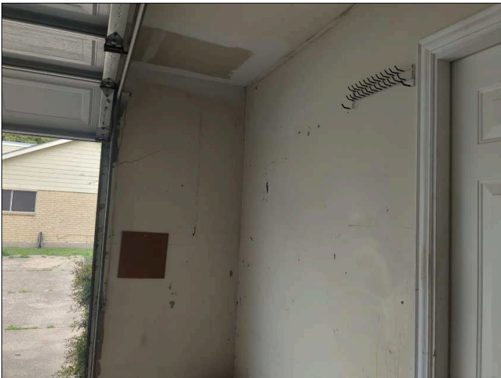
Paint is peeling in the garage walls. This is often a common occurrence due to high moisture of unconditioned garage space, recommend repainting to help prevent further deterioration.
