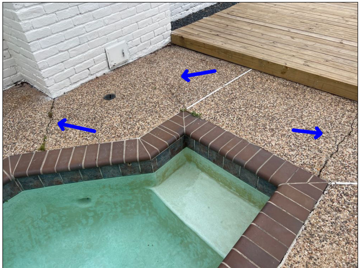
There are settlement cracks in the pool decking and coping.
