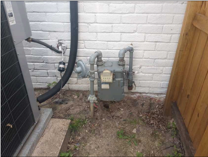
Overview of Gas meter
