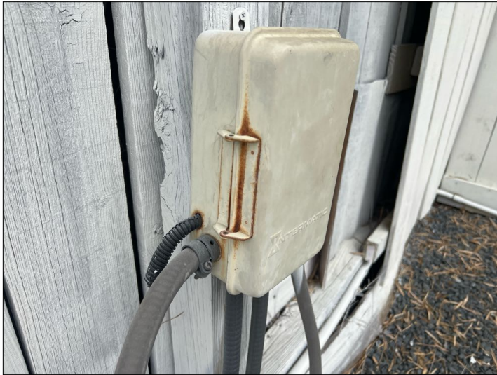
Pool timer is rusted.
