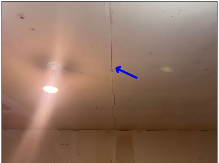
Settlement cracks were noted at the tape joint in the drywall. Mainly at - garage
