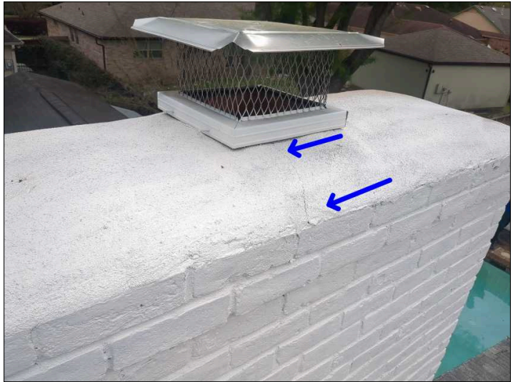
Seal all cracks in mortar cap to help prevent further deterioration.
