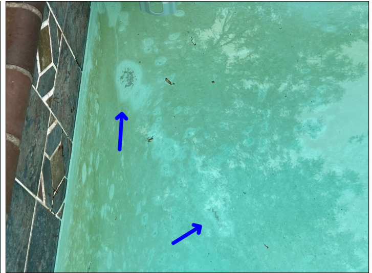
The surface of the pool is damaged. Unable to determine the condition of underlying materials. Mainly at - right
