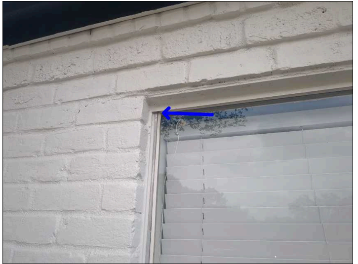
Glazing bead is loose, damaged or deteriorated. Recommend replacing or sealing damaged glazing bead to help prevent moisture penetration.
