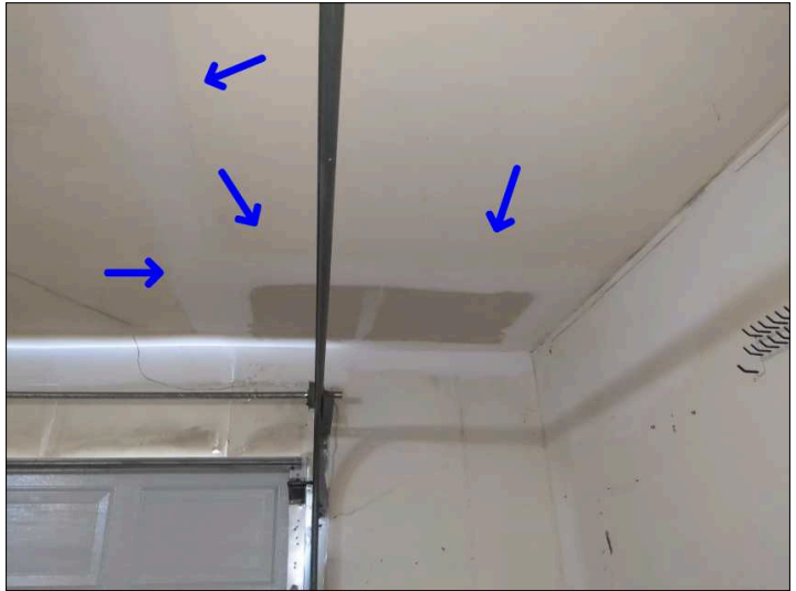
There is evidence of previous patch work and or painting on the interior finishes. Recommend contacting homeowner for more information. Mainly at - garage
