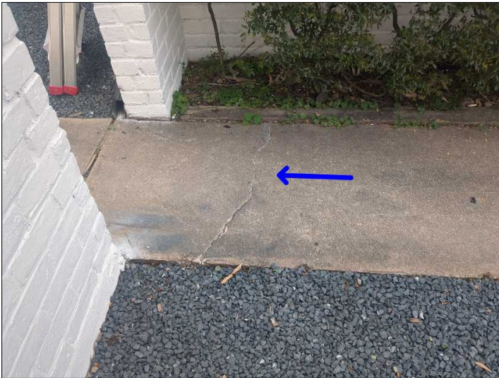
Cracks were noted in the pavement. These are cosmetic in nature at this time. Recommend sealing to help prevent further deterioration. Mainly at - front sidewalk
