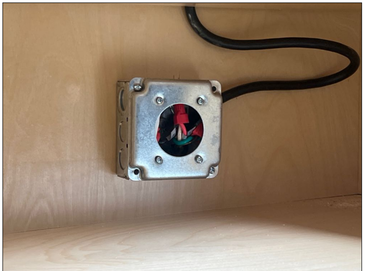
There are visible unprotected wiring splices. Recommend the wiring be properly enclosed. Mainly at - under cooktop
