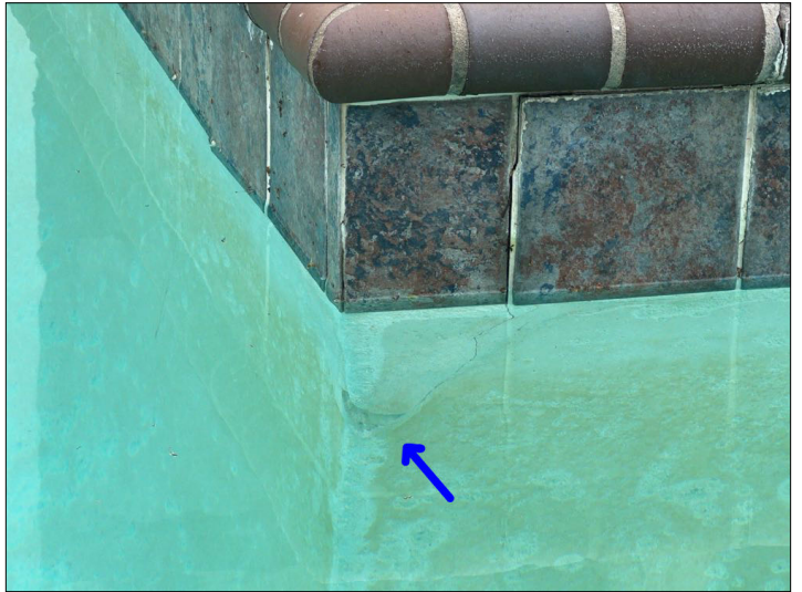
There are indications of a crack(s) in the pool surface. Unable to determine the condition of the underlying materials. Mainly at - left
