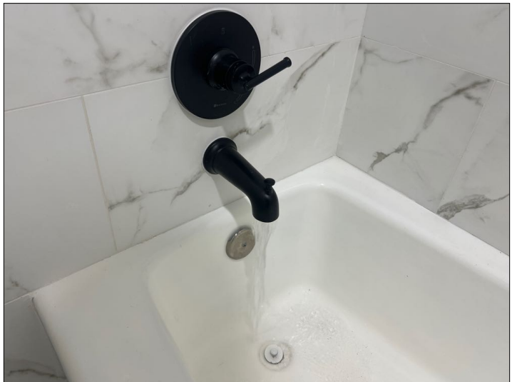
Overview of Plumbing Fixture(s) in Operation.
