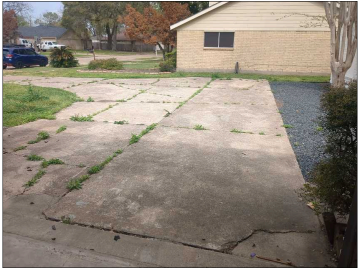
Uneven pavement was noted, recommend repairs to help prevent tripping. Mainly at - driveway
