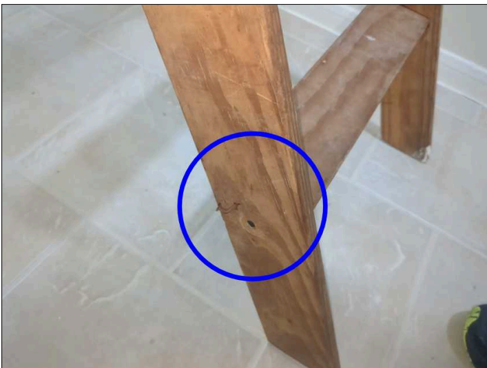
There is at least one nut loose or missing on the attic stairway, recommend checking all nuts and bolts to make sure they are all present and tightened.
