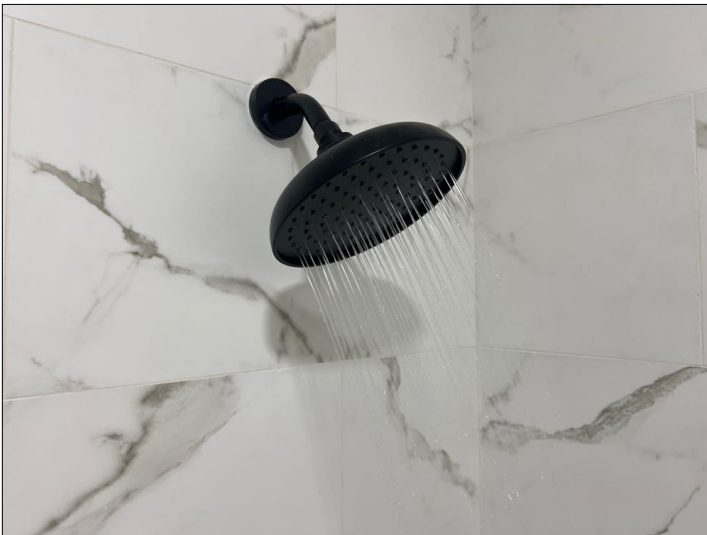
Overview of Plumbing Fixture(s) in Operation.
