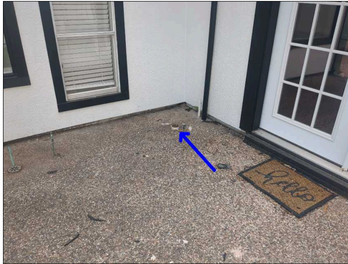
Overview of Service Point of Entry.
