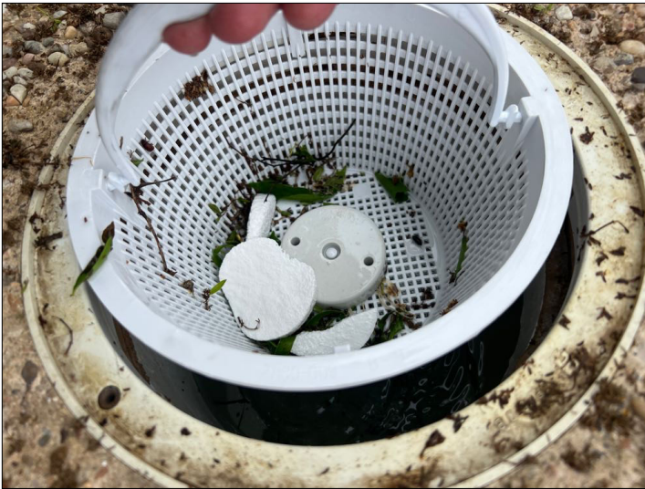
There are sanitizer tablets located in the skimmer basket. It is not recommended since this causes a strong concentration of chlorine to enter into the pump system damaging components.
