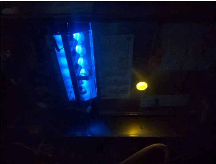
Overview of Furnace burner compartment in operation
