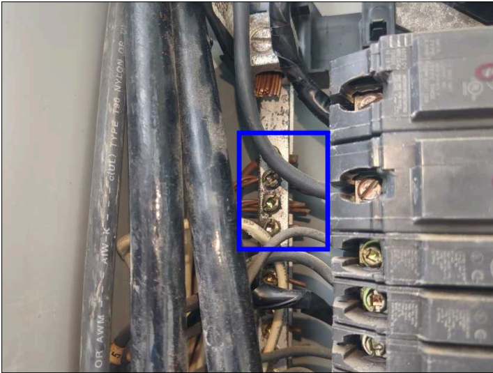
There are more than two ground wires located under the same screw on the ground bar. Ground wires should have no more than two wires under an individual screw.
