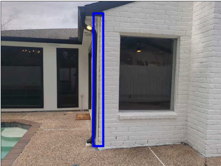
Recommend sealing between the trim and brickwork to help prevent water penetration. Mainly at - rear
