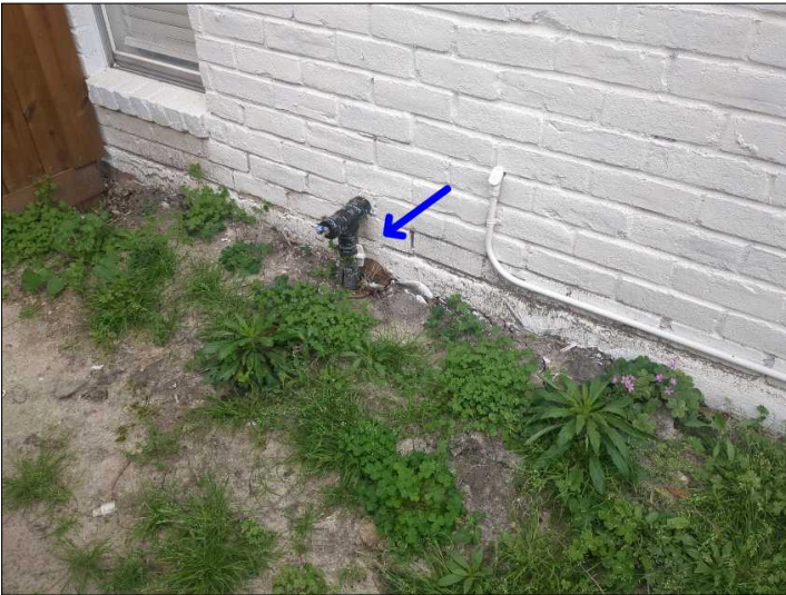
Overview of Water shut off valve
