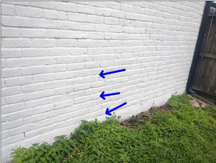
Settlement cracks were noted in the brickwork. Mainly at - right side front
