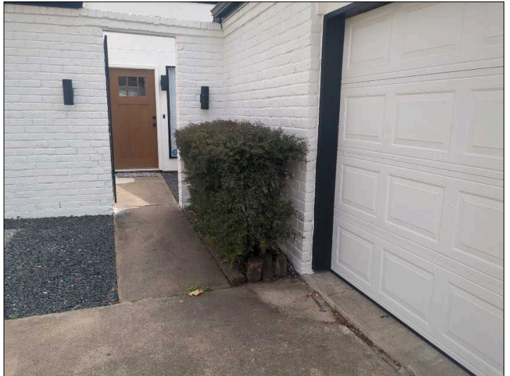
Recommend trimming vegetation so that it is not in contact with the house. Vegetation in contact with the structure can hold moisture against the structure and promote damage to building materials and conducive conditions for wood destroying insects.
