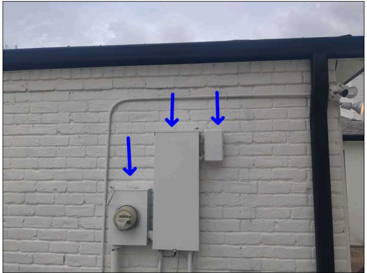
It is recommended that Electric Panels, Meter Boxes and Disconnects be sealed between the box and the Exterior cladding to help prevent water penetration.
