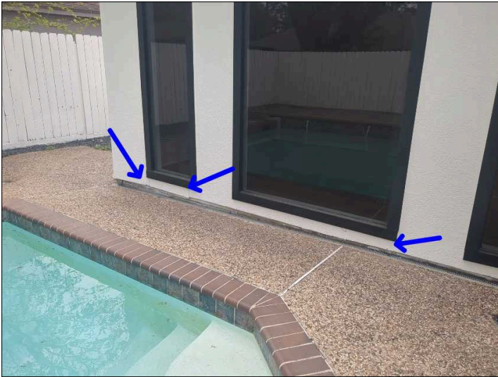
There is some damage to the exterior siding, recommend repair or replacement to help prevent water penetration. Unable to determine the condition of the underlying materials. Mainly at - rear right
