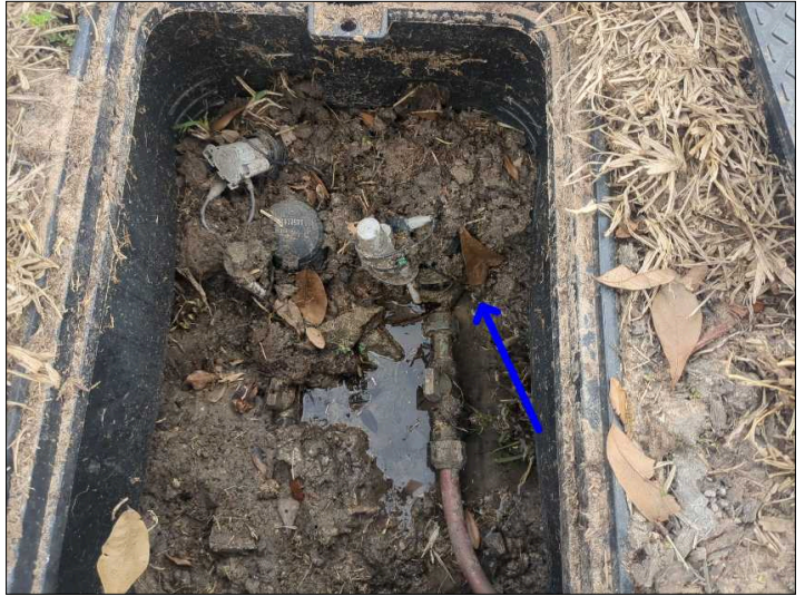
Leak/water movement noted in the meter box at the water meter.
