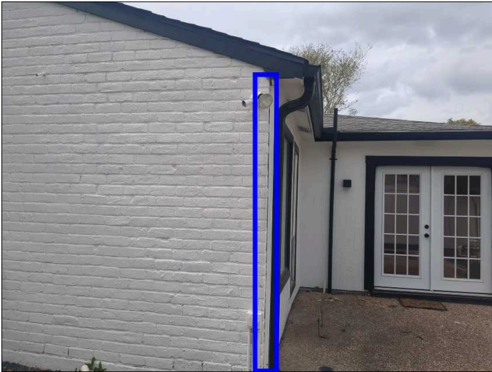
Recommend sealing between the trim and brickwork to help prevent water penetration. Mainly at - rear
