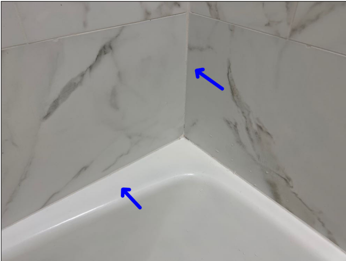
Grout was used in the corners of the tub/shower. It is recommended that a flexible sealant be used in the corners to allow for movement to help prevent future cracking in the corners of shower stalls and tub surrounds due to settlement.
