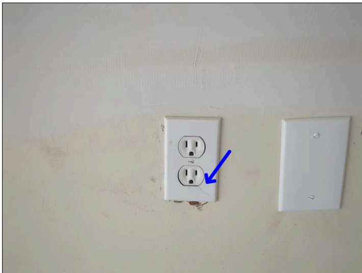
Receptacle plate is broken or missing, recommend replacing covers to help prevent electrical shock. Mainly at - garage
