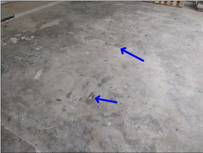
Cracks were noted in the pavement. These are cosmetic in nature at this time. Recommend sealing to help prevent further deterioration. Mainly at - garage
