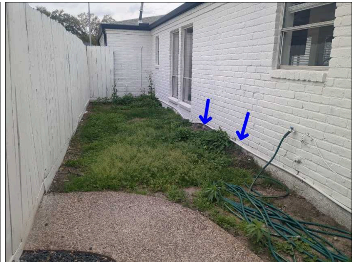
The soil or concrete is too high or footing is too low which does not allow proper exposure of the slab. This can cause conducive conditions for Wood Destroying Insects or water penetration usually if there is improper slope. Mainly at - right side rear
