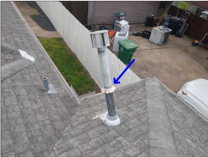
There are signs of rusted vents or flashing on the rooftop. We recommend painting or replacing all rusted or deteriorated vents or flashing as needed.
