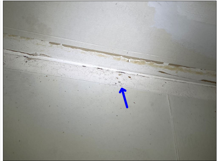
Mold like stains are present. Recommend contacting our office to schedule an evaluation and mold testing to determine the type of mold and identify the source of contamination. Mainly at - garage
