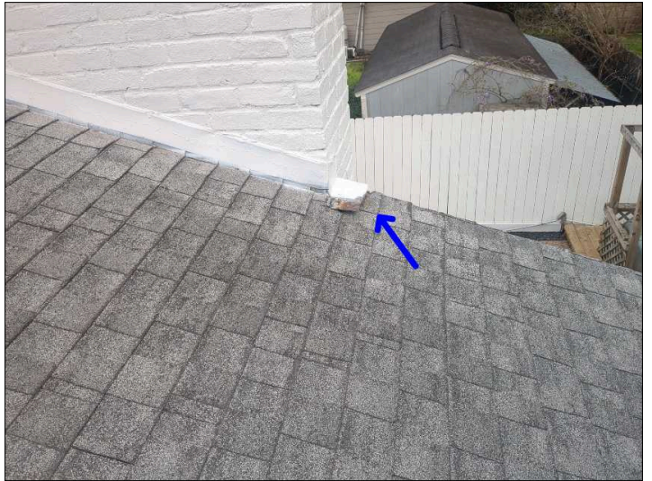
The roof flashing is lifted. Recommend securing all loose or lifted flashing and sealing nails to help prevent water penetration.
