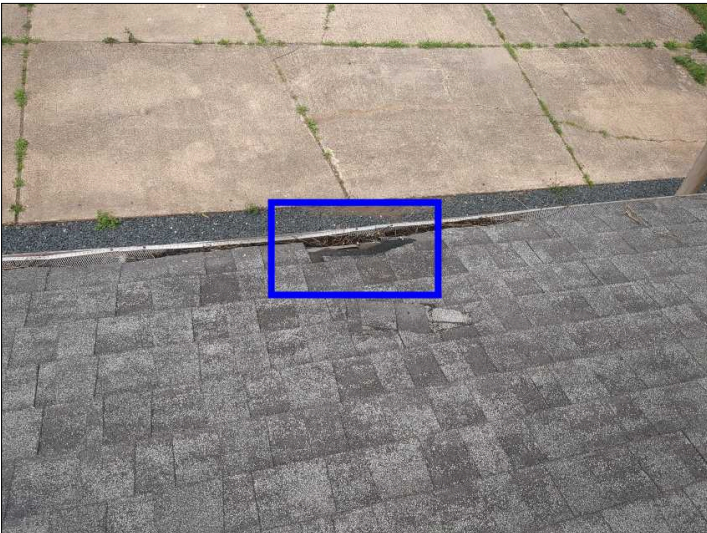
There are damaged or missing shingles on the roof, recommend repairs or replacement of damaged shingles.
