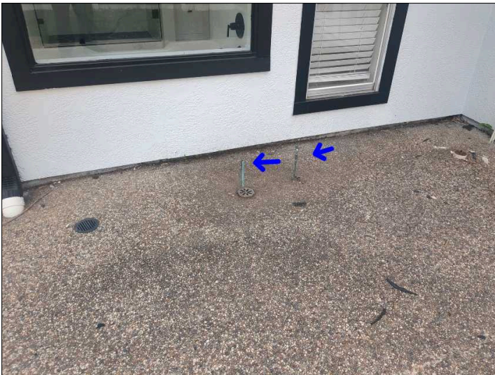
Copper tubing is noted to be coming through the spa deck in the left rear. Recommend removing to help prevent trip/fall hazard.
