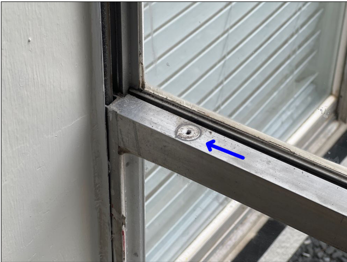
The window lock/latch is missing. Mainly at - front entry
