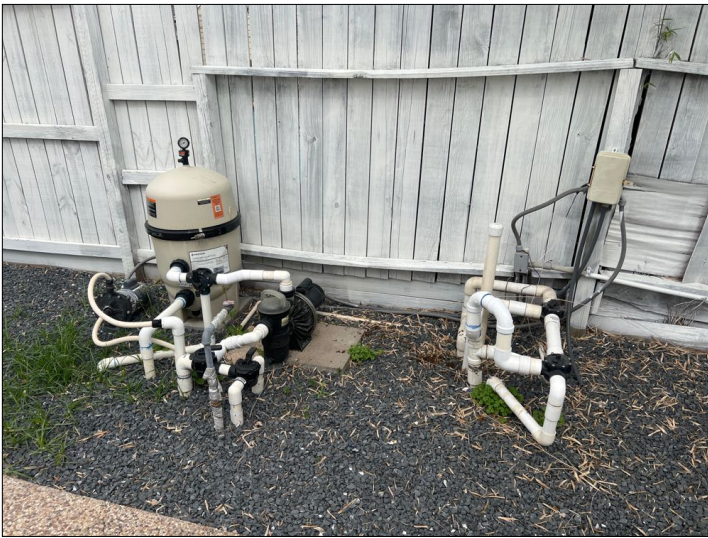
Overview of pool equipment
