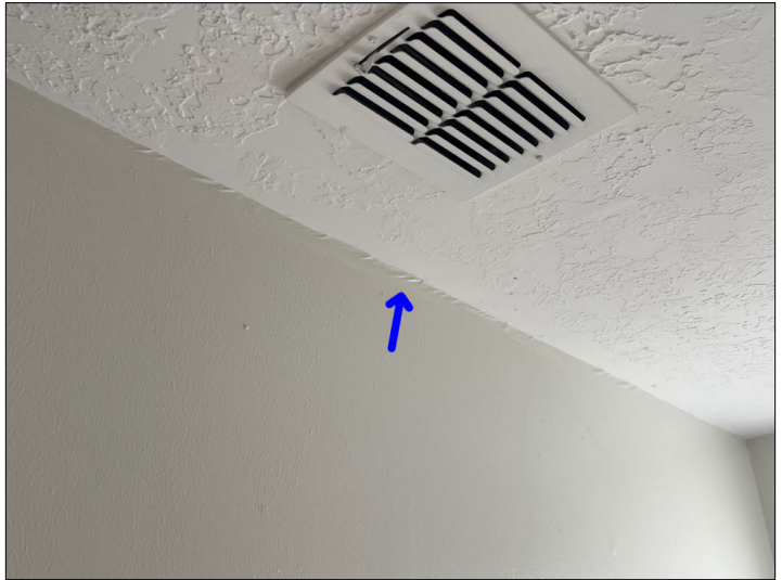
Tape is twisting due to movement in the corners of the drywall, this is normally a sign of foundation movement or structural settlement, other movement noted may give signs of the cause. Mainly at - laundry
