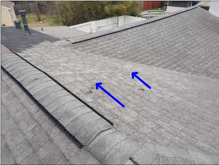
The decking is buckling on the roof, this is often caused by an improper gap for expansion of the decking materials, recommend consulting a roofing contractor for evaluation and repairs as needed.
