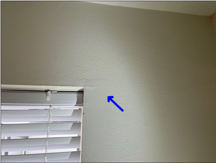
There is evidence of previous patch work and or painting on the interior finishes. Recommend contacting homeowner for more information. Mainly at - front entry
