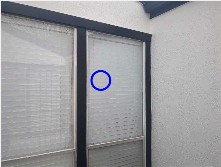
A hole was noted in a window pane. Mainly at - front
