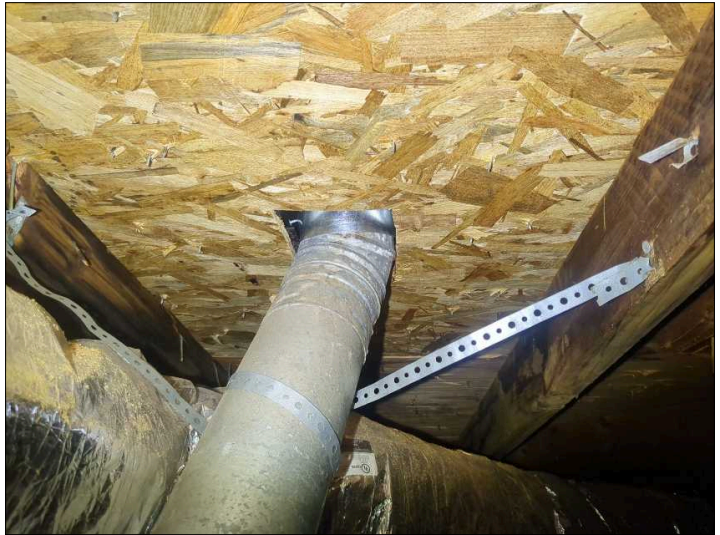
There is improper clearance around the flue pipe, the furnace vent should have at least 1" clearance to combustibles.
