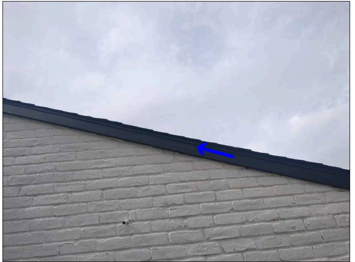
Recommend sealing trim to help prevent water penetration. Mainly at - rear
