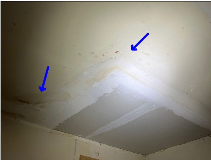
There are indications of water penetration to the ceiling evident mainly by staining. Unable to determine condition of the underlying materials. Mainly at - garage
