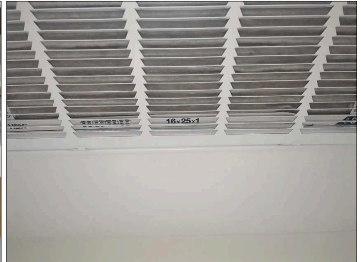
Overview of disposable filter
