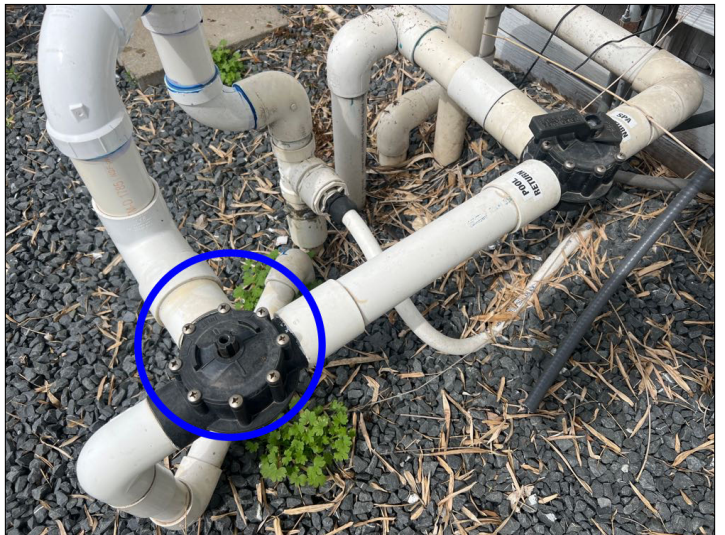
The valve handle is missing.
