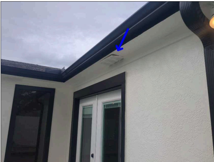
The attic vent screen is loose, damaged or missing, recommend repairs to help prevent unwanted entry.
