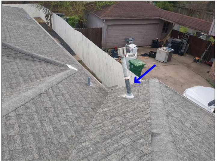
One or more of the vents and or flashing is unpainted, recommend painting all unpainted vents and flashing to help prevent damage due to UV rays or rust.
