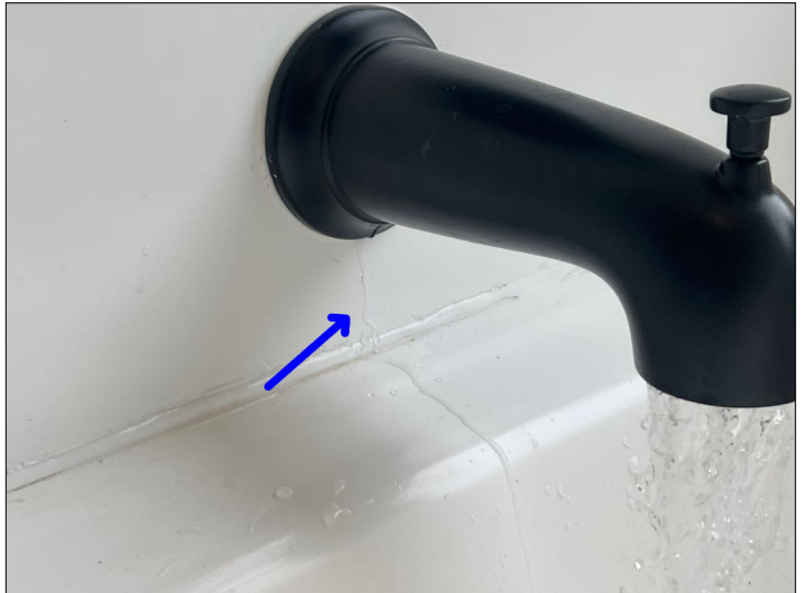
There is a water leak at the base of the faucet, recommend repair or replacement. Unable to determine condition of underlying materials. Mainly at - primary bath
