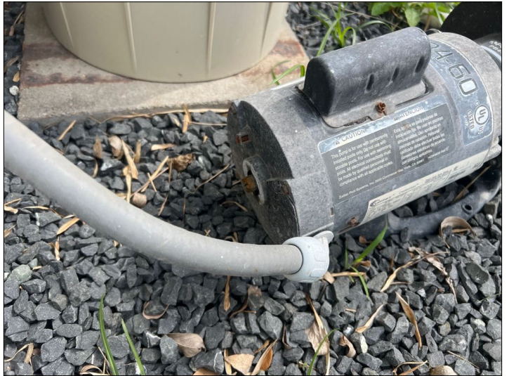
There is no evidence of electrical bonding between the pool and the pool equipment.
