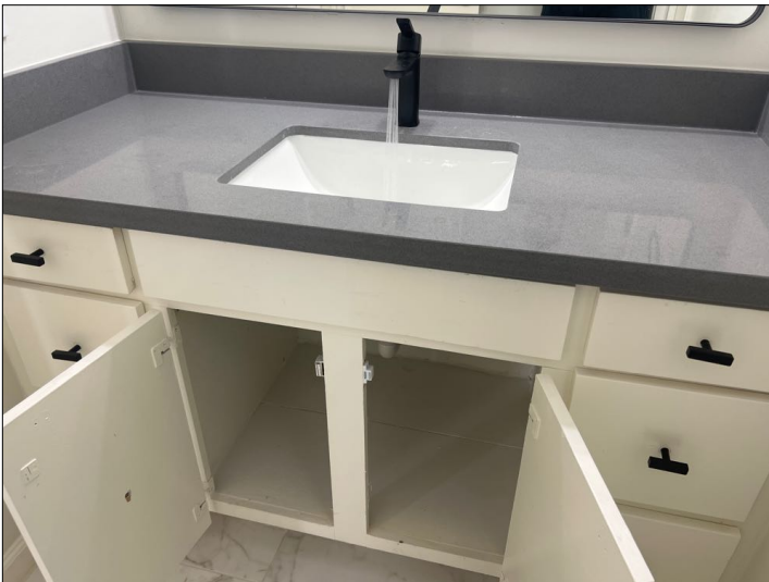
Overview of Plumbing Fixture(s) in Operation.
