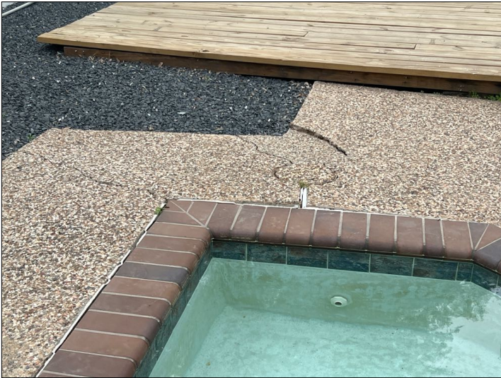
There is uneven pavement noted around the pool or spa.
