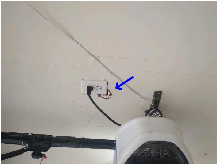
There is at least one hole in the ceiling in the garage. All holes in the garage ceilings or wall against living areas should be patched to help keep the recommended fire barrier between the home and garage.
