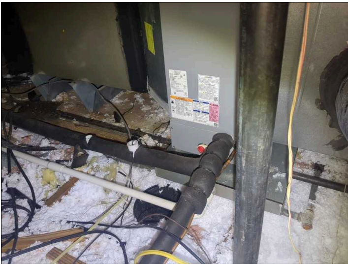
Overview of A/C Evaporator
