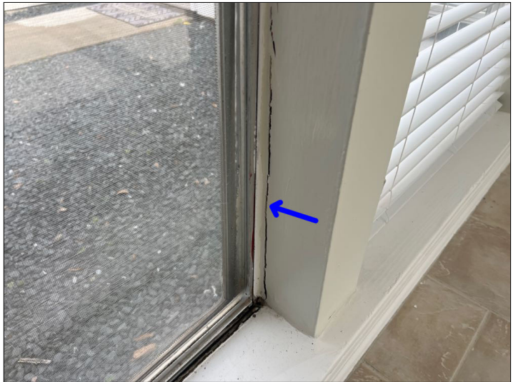
Sealant is needed around the interior of the windows between the window framing and the drywall to help prevent water penetration.
