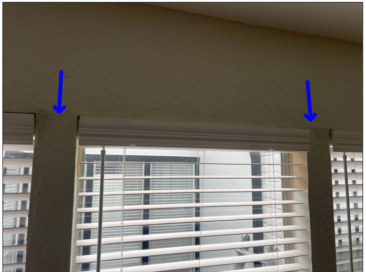
Settlement cracks were noted in the drywall. Mainly at - front right bedroom
