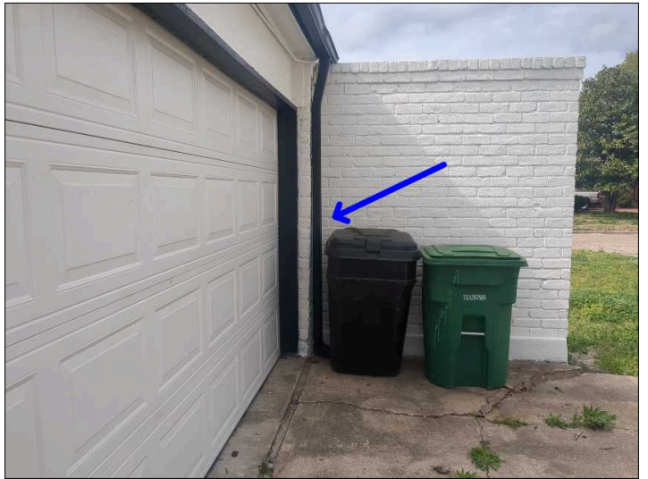
The gutters are sagging and/or loose. Attention to the gutters is required to keep them functioning as designed. Mainly at - front
