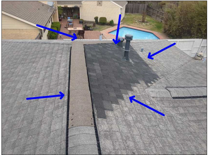
Signs of previous repairs were noted on the roof. Indications are that they are working as intended at time of inspection.
