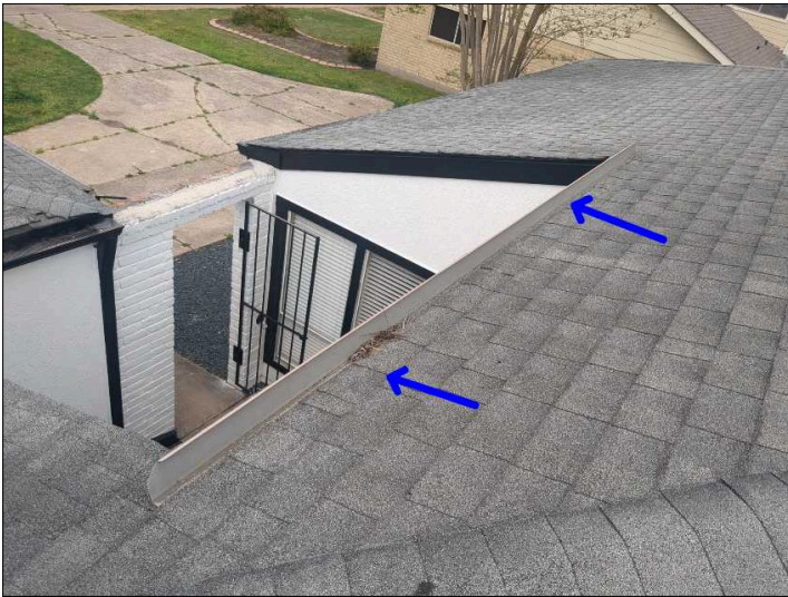
One or more of the vents and or flashing is unpainted, recommend painting all unpainted vents and flashing to help prevent damage due to UV rays or rust.
