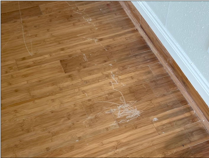
There are scratches noted in the wood flooring. Mainly at - living room
