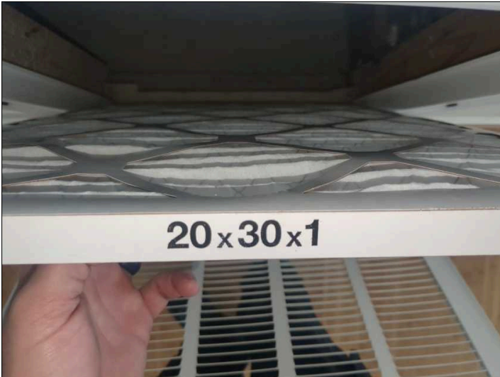
Overview of disposable filter
