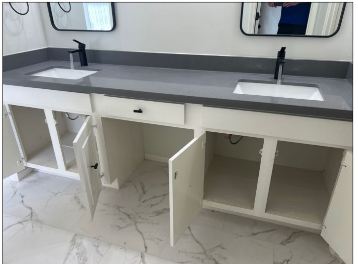
Overview of Plumbing Fixture(s) in Operation.
