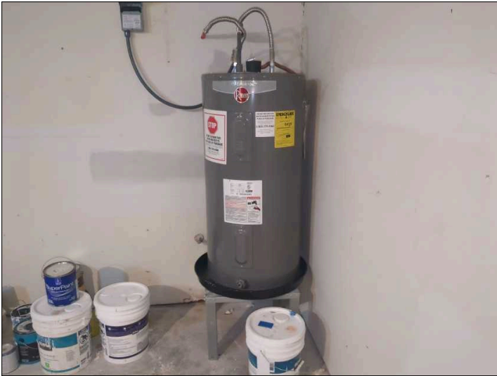
Overview of Water heater
