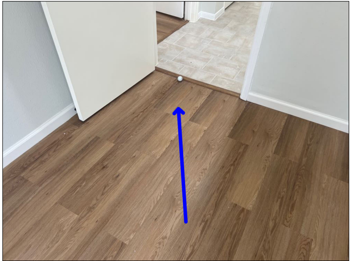
Uneven or sloping floors were noted. Some times in older homes minor slopes may be due to construction methods at that time, however if floors are sloping more than normal it is recommended that some follow up investigation be made. Sloping floors can be caused by foundation movement or from structural issues usually on upper floors. Floors were noted to be sloped. Mainly at - front middle bedroom
