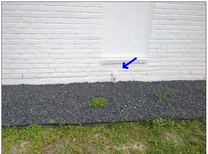
Electrical receptacle(s) are registering an open ground. Mainly at - front right exterior
