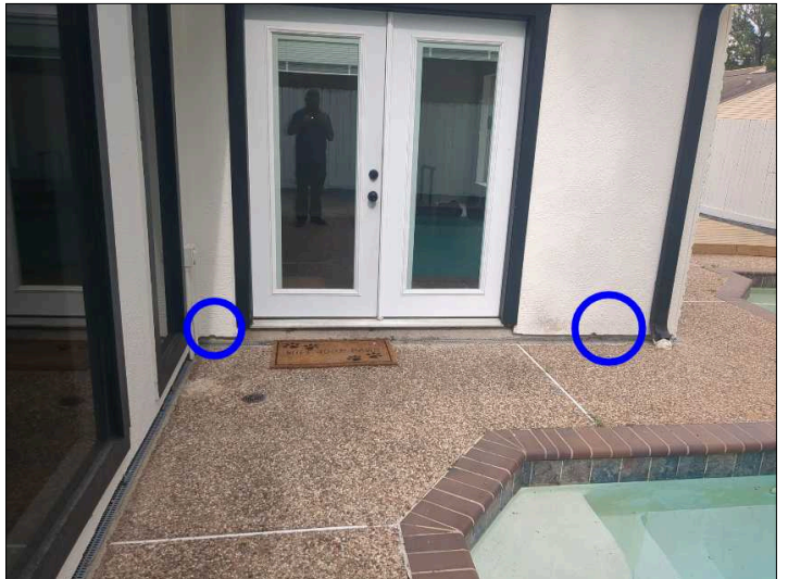
There is some damage to the exterior siding, recommend repair or replacement to help prevent water penetration. Unable to determine the condition of the underlying materials. Mainly at - rear right
