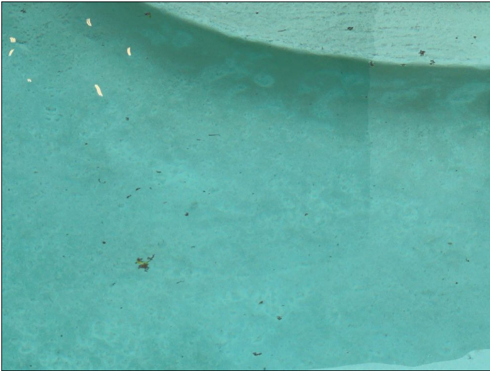
The surface of the pool is worn. Unable to determine the condition of underlying materials.
