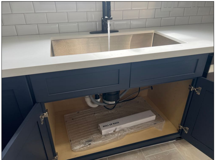
Overview of Plumbing Fixture(s) in Operation.
