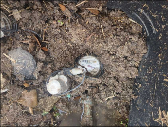
Overview of Water meter
