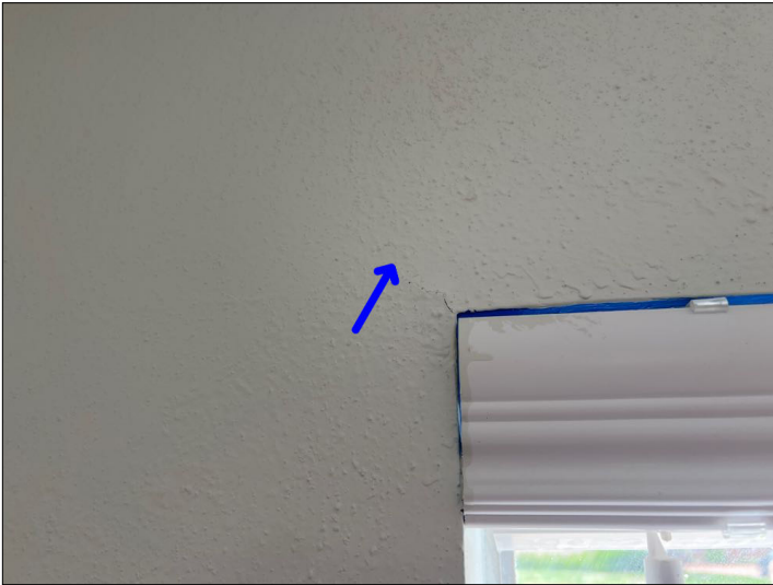
Settlement cracks were noted in the drywall. Mainly at - front middle bedroom
