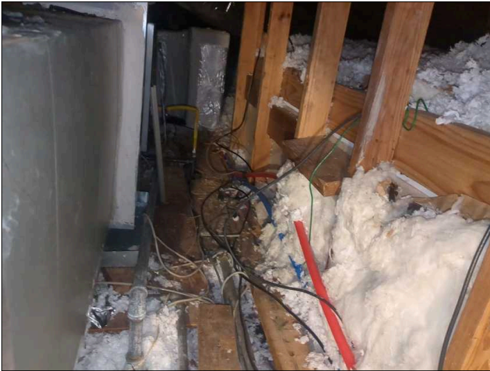
There is not an adequate workspace and/or pathway to the furnace, located in the attic as recommended.
