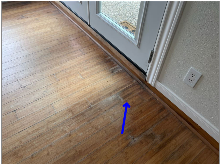
There are signs of discoloration or moisture damage on the floor. Mainly at - living room
