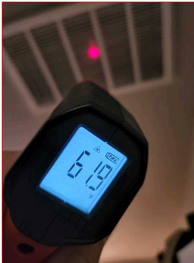
Return temp 61.9 degrees. Master bedroom area.
