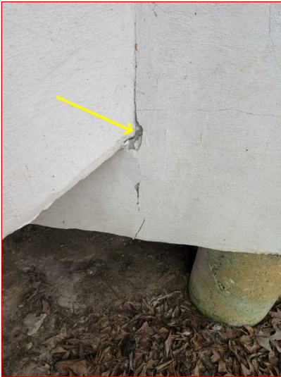
Cracks were noted.
