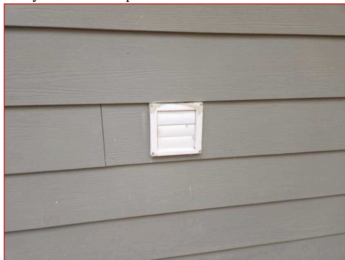
Recommend dryer duct to be cleaned periodically to keep it clear of lint.
