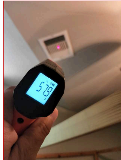
Supply temp 57.9 degrees. North side.
