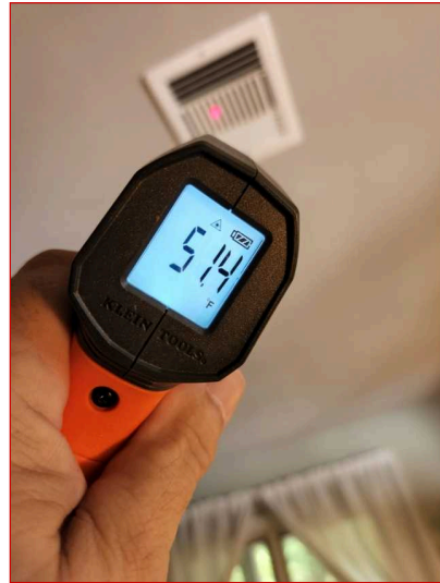
Supply temp 51.4 degrees. Master bedroom area.
