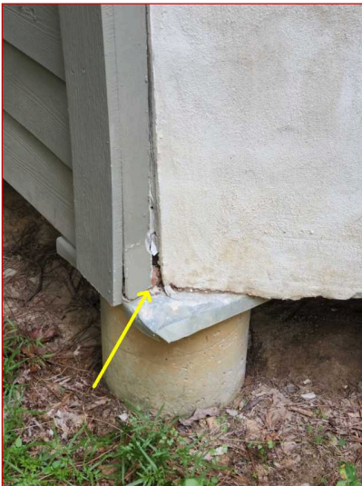
Repairs needed at one or more areas around the home.
