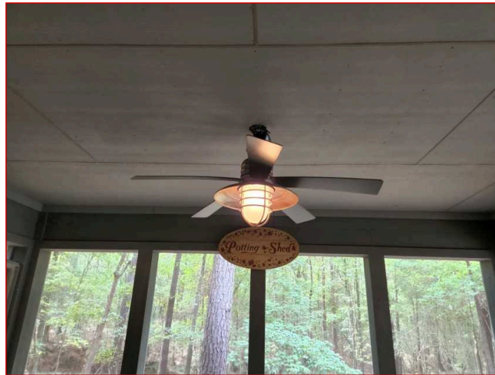
Ceiling fan not working.
