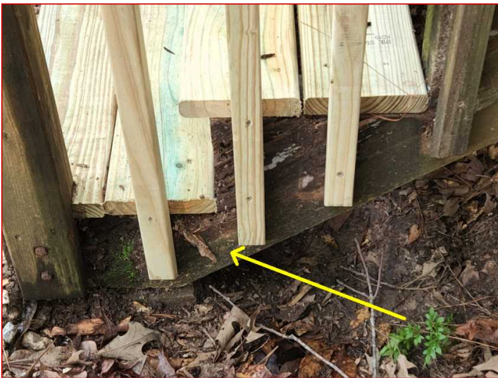
Stringer needs replaced at front steps.
