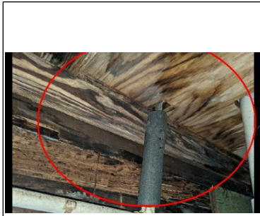
Moisture damage under bathroom viewed from the crawlspace
