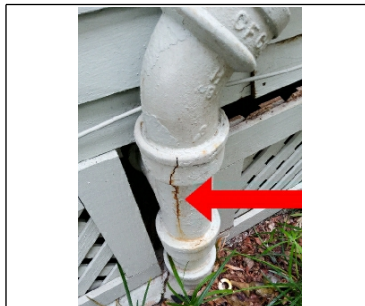
Crack in old cast iron or steel drain waste line
