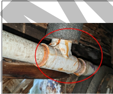
There was a leak in the distribution lines for the bathtub
