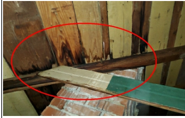
Moisture stains observed from inside the attic
