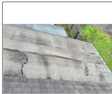
Flat roof has excessive granule loss
