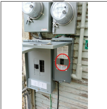
70amp main breaker for front home is located at the rear garage apt in the northwest corner
