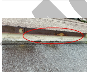
Fascia board over the north side of the flat roof is deteriorating
