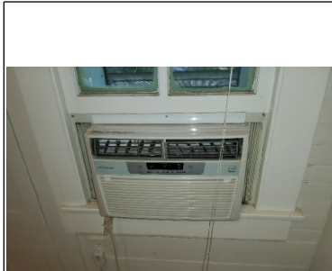
Kitchen window unit functioned properly
