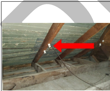
Old knob and tube wiring in the attic was still in use
