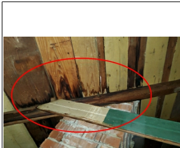
Moisture stains at the penetration of the roof from the chimney
