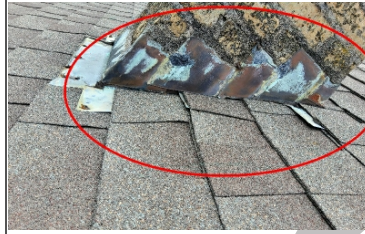
Flashing at the roof likely needs resealed
