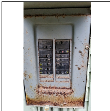
Breaker box is rusted
