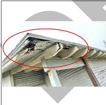
Southeast corner has deterioration of the roof structure
