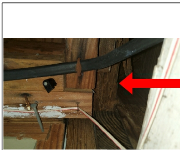
Picture is looking up at the right side just inside the west garage entry, there appears to be previous wood destroying insect damage
