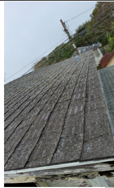
Shingles have suffered from extensive granule loss
