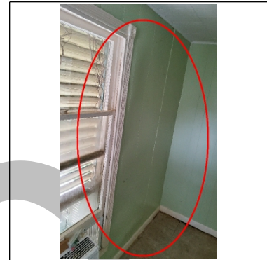
Damage at the south wall
