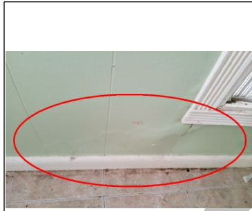
Damage under the south window
