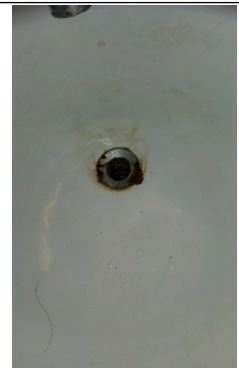
Sink missing drain stop
