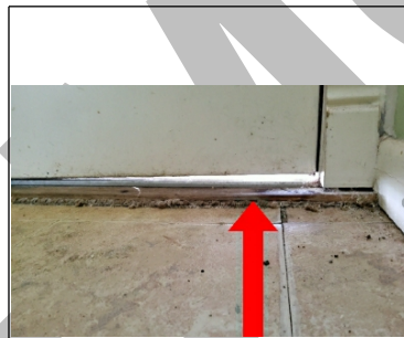
Door at the area above the damage from the wood destroying insects or moisture, you can see there has been a significant drop in the area
