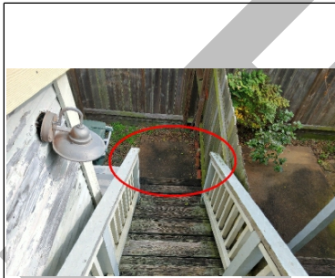
Handrail did not quite reach all the way to the bottom of the stairs
