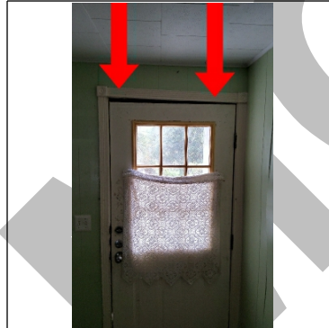
Front entry door is not square and catches the frame when opened
