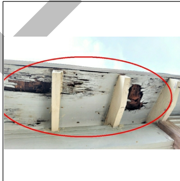
Roof decking at the southeast corner is deteriorating
