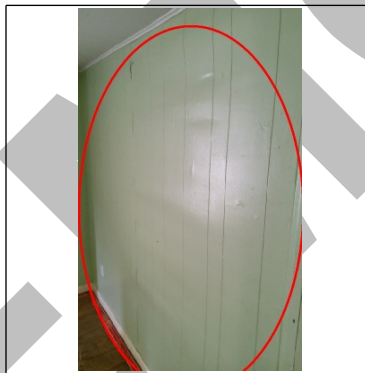
North wall has damage behind paneling
