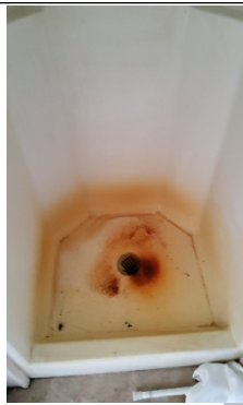
Rust stains all over the stand up shower
