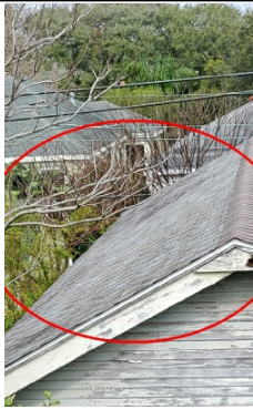
Tree limbs on the west side of the home have caused damage to the roofing materials
