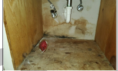
Significant moisture damage and fungal growth under bathroom sink
