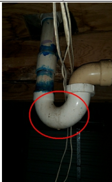
Active water dripping from trap
