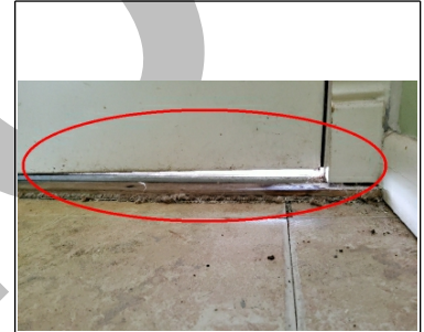
Gap at the front entry door
