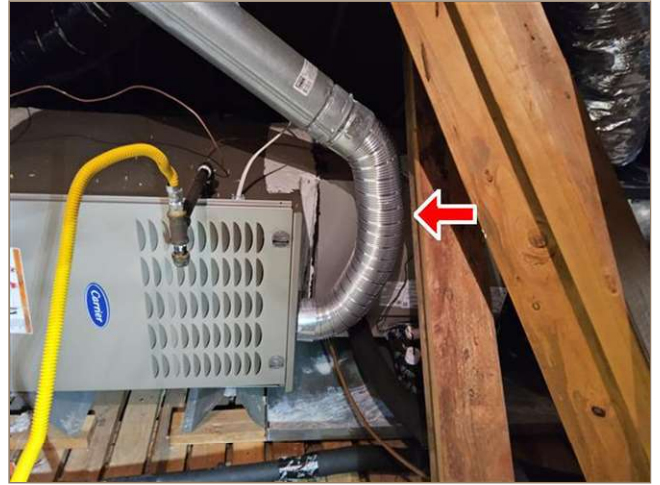
downstairs unit - missing B-vent
