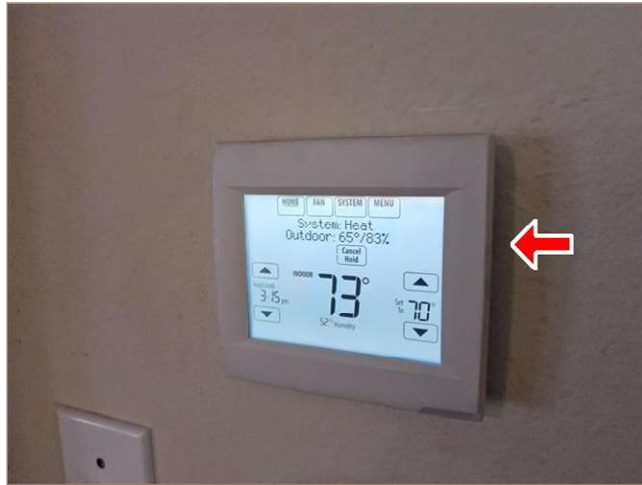
unable to test heater upstairs
