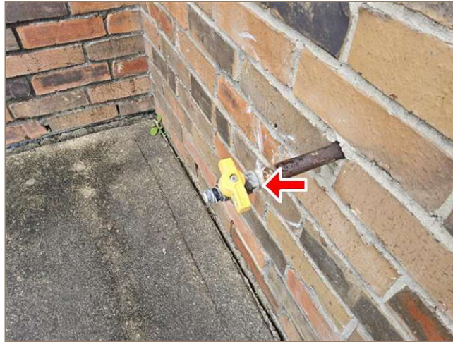
patio kitchen missing cap safety hazard
