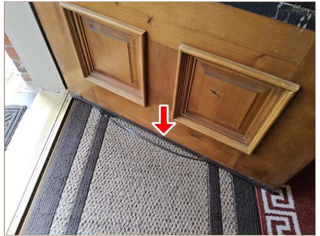
weather-stripping front entrance
