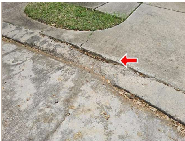
front tripping hazard
