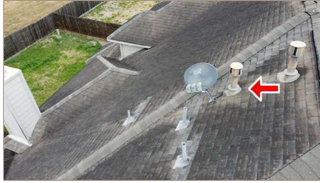
replace all pipe jacks and vents at next re-roof
