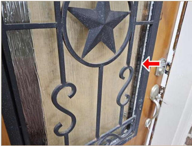
front glass panes broken front entrance
