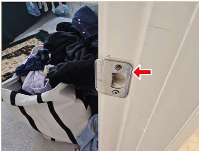
rear right bedroom missing screws
