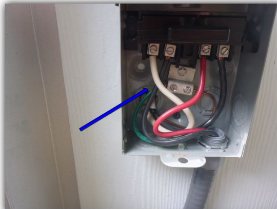
Incorrectly sized breaker - Unit recommends maximum 15 amp breaker and oversized 30 amp breaker is installed. Change to proper size as per manufacturer. Extend condensate drainline 3 to 5' away from foundation of house.
