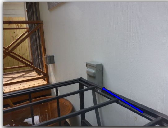
Incorrectly sized breaker -
