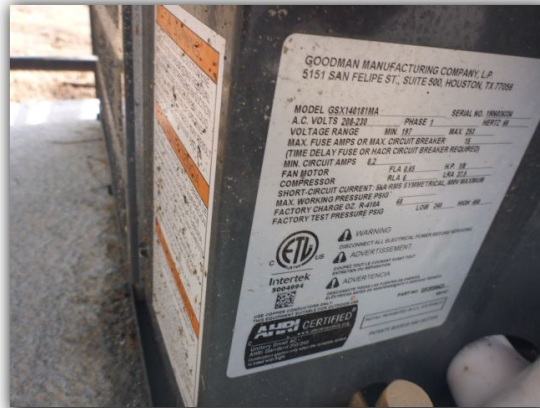
Evaporator coils are icing over at time of inspection, in need of repairs.
