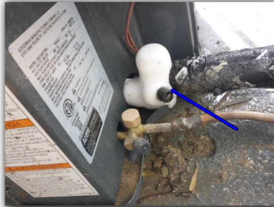
Disconnect - White wires used as hot legs need to be labeled as hot with black or red markings.
