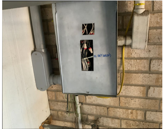
Abandoned old panel in garage
