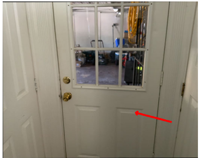
Fire rated door required from garage to home.
