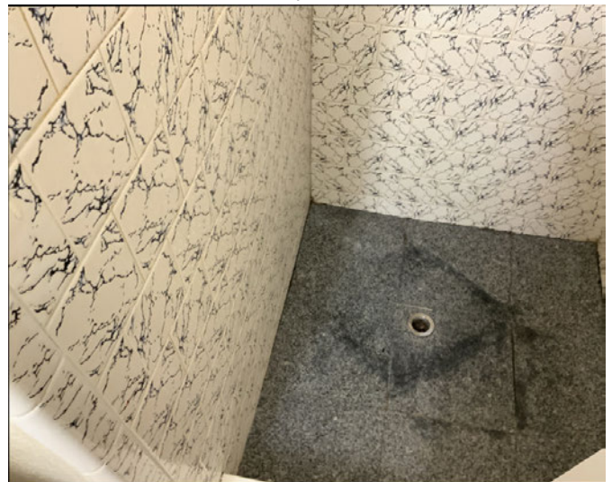
Caulking improvements needed at showers
