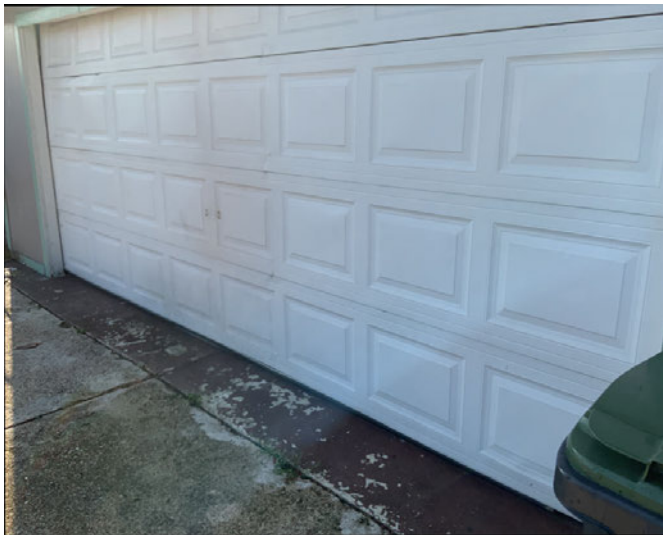
All panels are damaged
