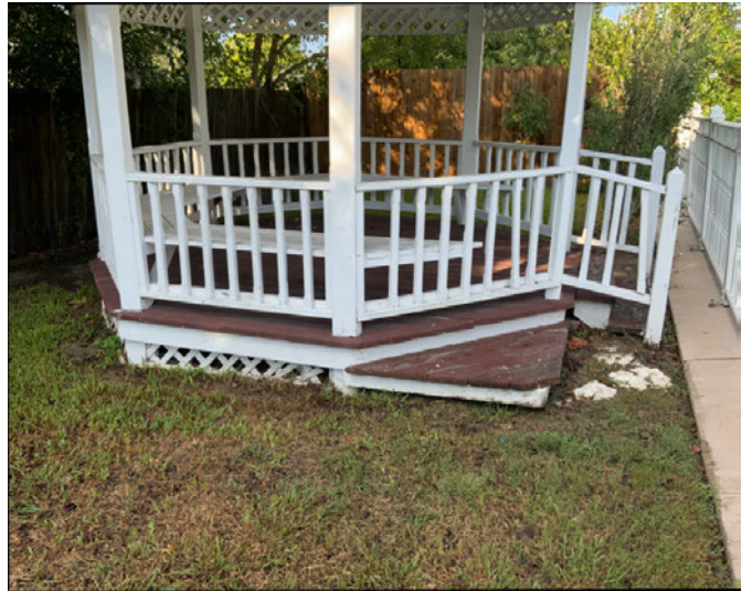
Damage pergola needs further evaluation by a professional to determine level of repairs needed
