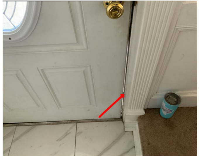
Door seals needed
