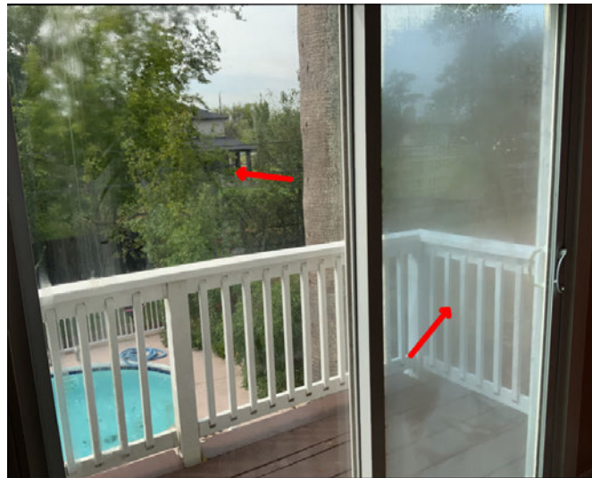
Lost seals at sliding glass doors. New glass is needed
