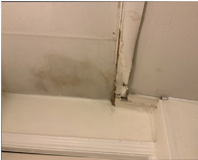
Water stains in outdoor bathroom ceiling
