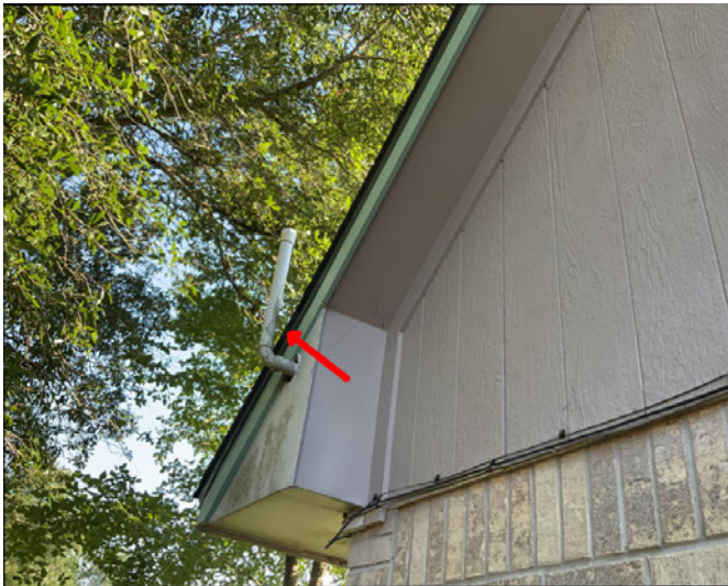
Proper venting required
