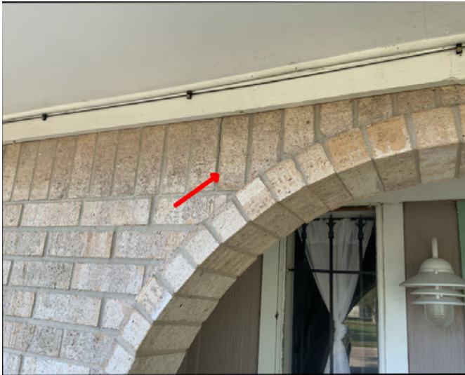
Settlement cracks in front
