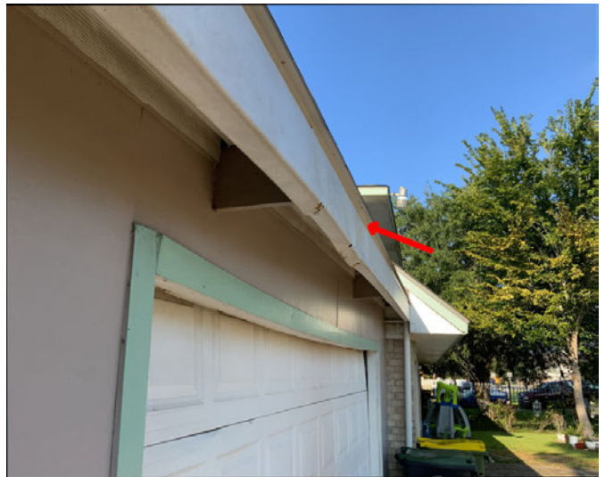
Damaged header over garage door
