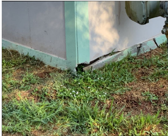
Damaged siding and trim boards
