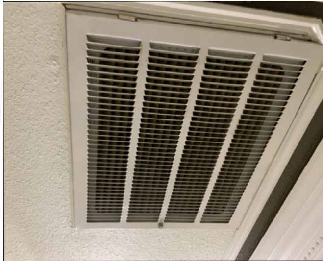
Dirty air filters
