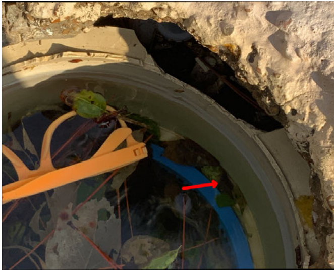
Damaged skimmer housing needs replacing
