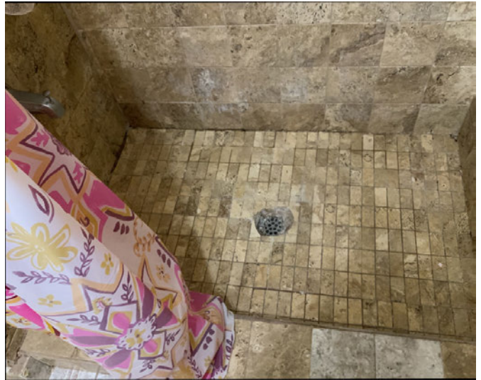
Recommend repairs at primary shower base
