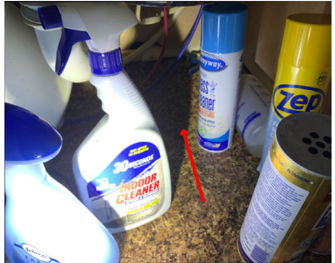
Evidence of past leaks under kitchen sink
