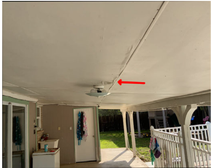
Further evaluation of patio cover needed. Leaks also observed at patio cover
