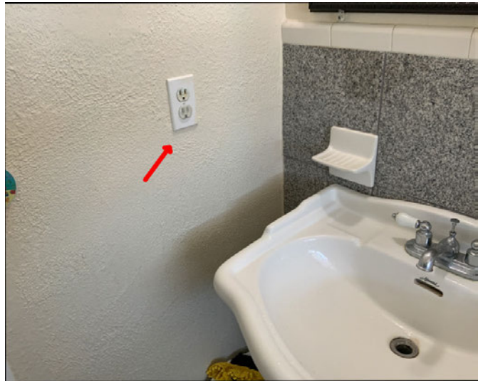
GFCI protection needed
