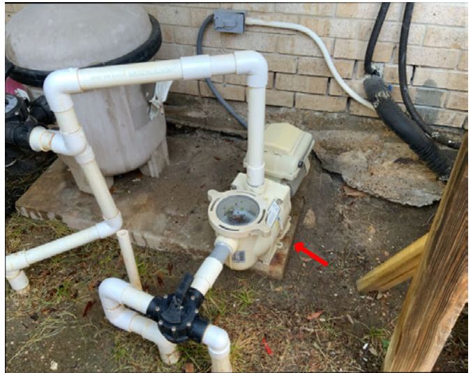
Pump bonding is required
