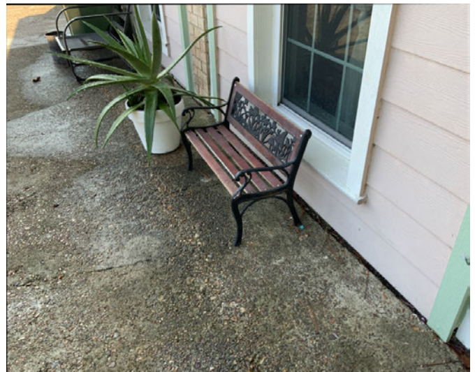
High soil blocking visual inspection of foundation
