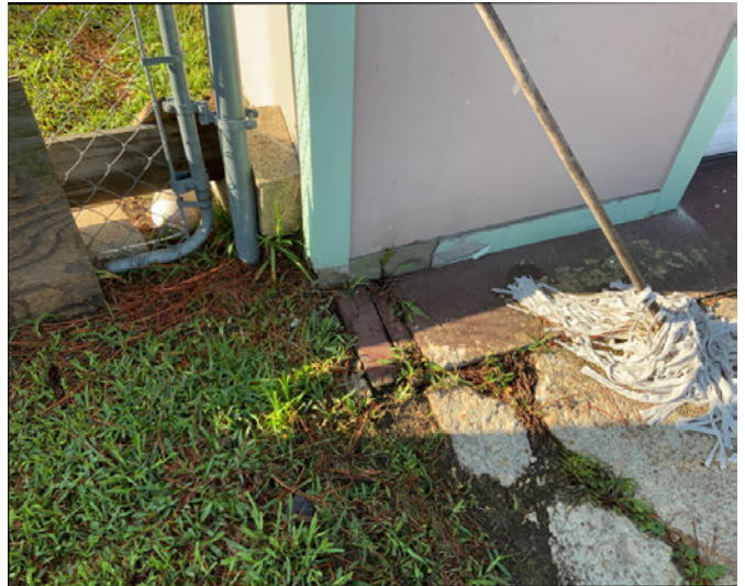
Damaged trim boards
