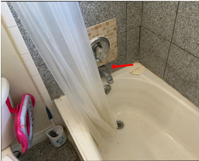
Faucet seals needed
