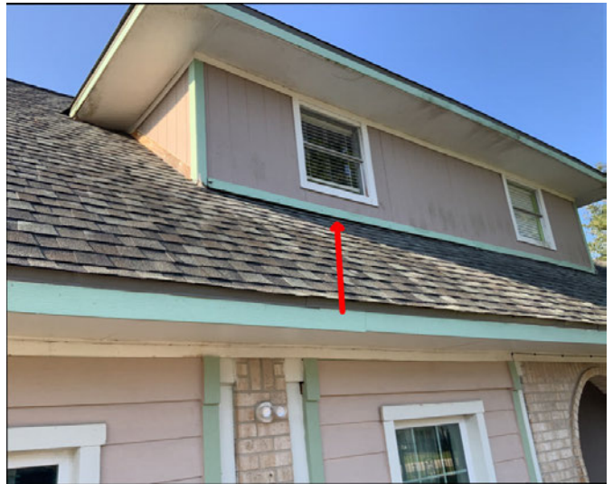
Decaying trim boards
