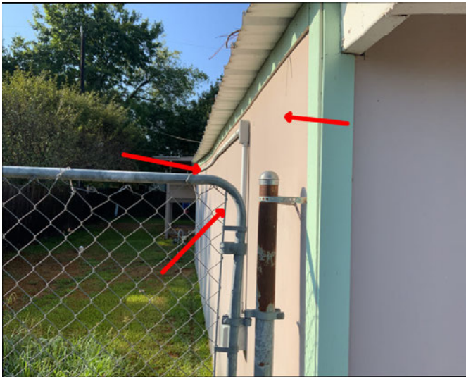
Damaged curved wall on left side
