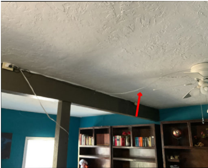
Extension cords used as permanent electrical supply is a potential hazard
