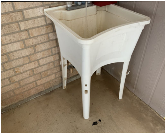
Laundry tub not mounted
