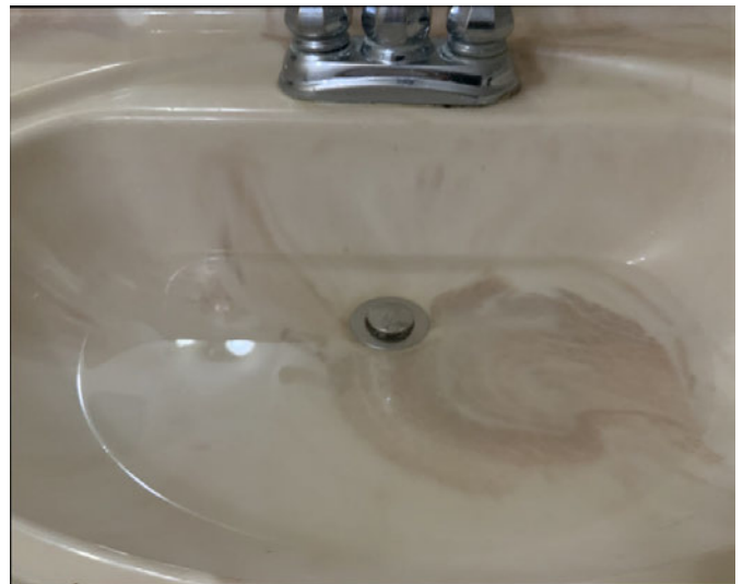
Slow drain at primary bathroom
