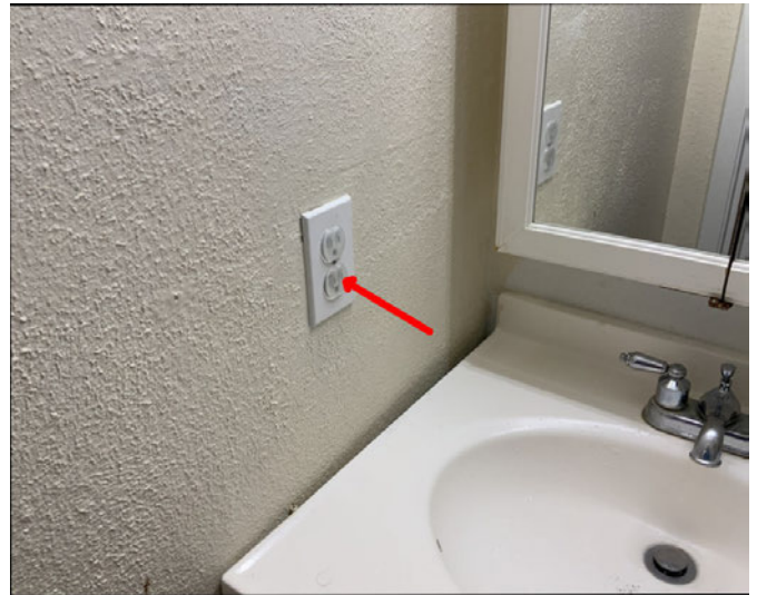
GFCI protection required
