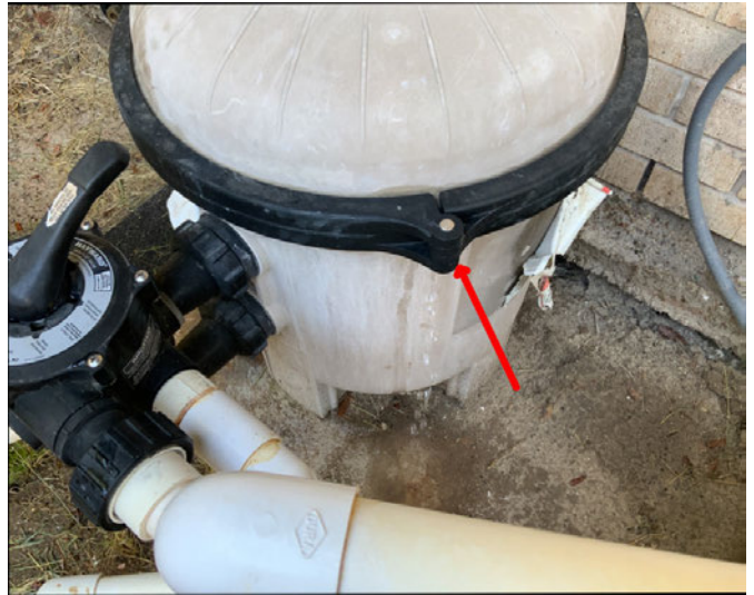
Leaking filter housing in 3 spots
