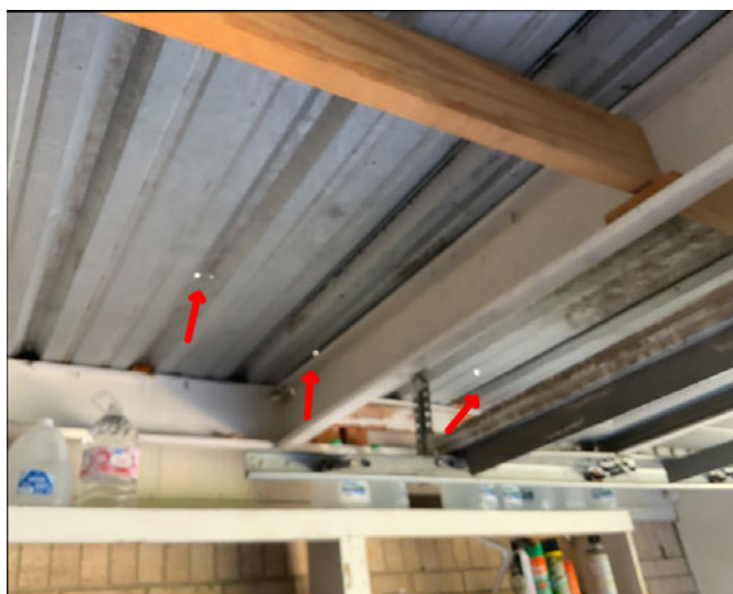
Holes in metal roof over garage. Further evaluation needed to determine level of repairs needed in this area and at leaking flat roof over patio.
