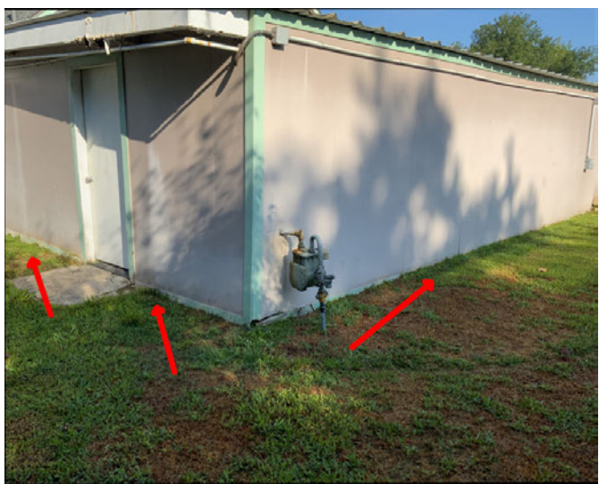
High soil blocking visual inspection of foundation
