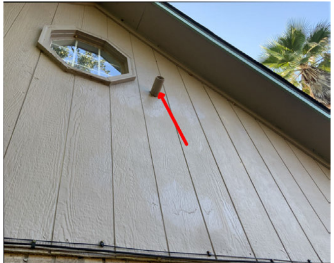
Proper venting required
