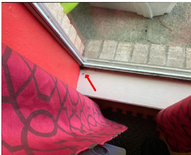
Moisture damage at sills and interior caulking needs improvements
