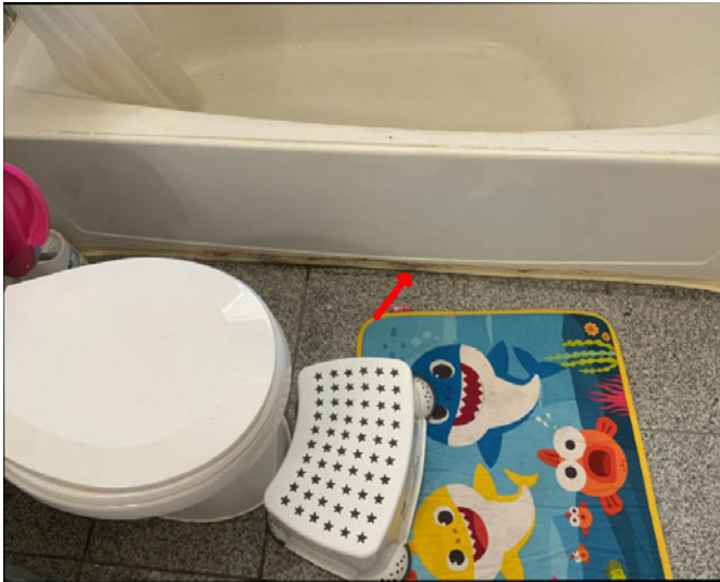
New base seal needed
