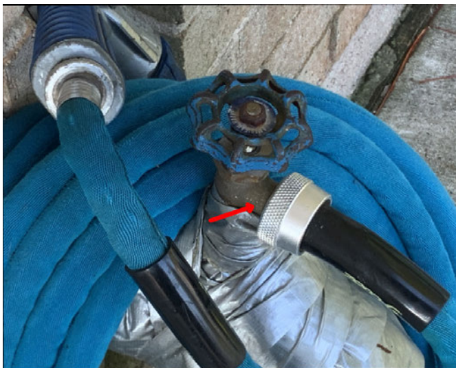
Anti siphon valves are required
