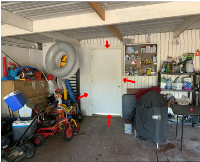
Door seals needed at garage door
