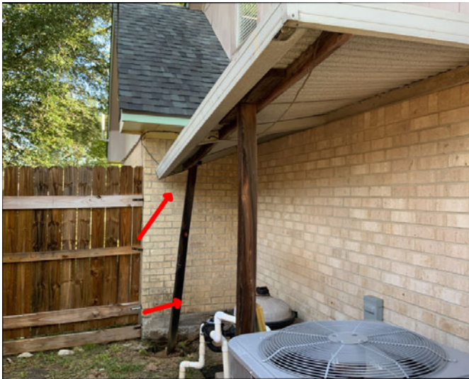
Recommend removing unsafe cover over equipment
