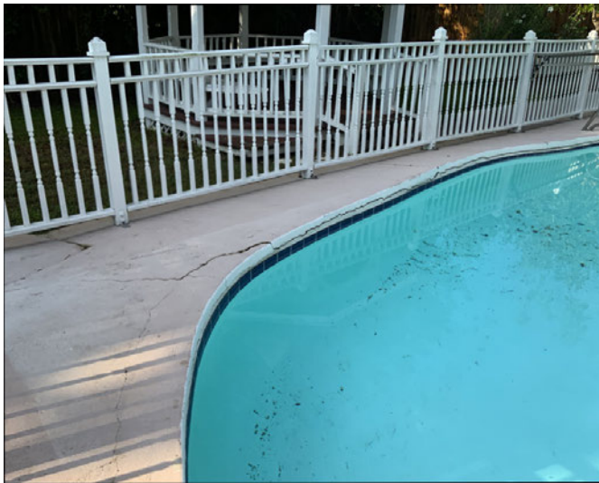
Major movement at pool deck surface and cracks at pool perimeter
