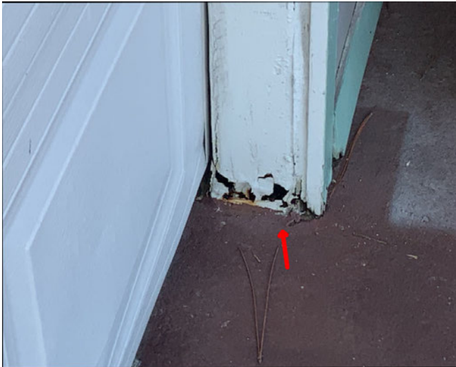
Decaying trim boards
