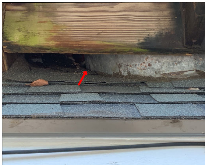
Correct clearance to combustibles is required
