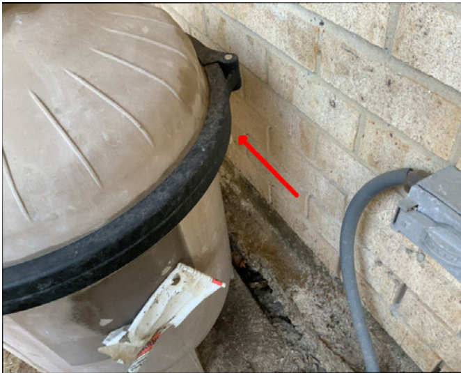
Leaking filter housing
