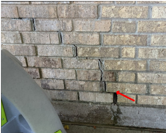
Large movement cracks at right front
