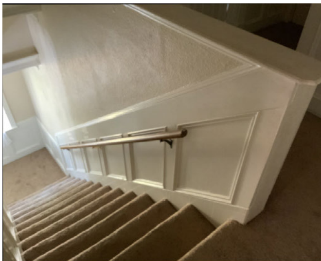
See handrail requirements and correct
