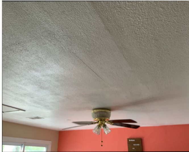
Patching in multiple areas throughout home
