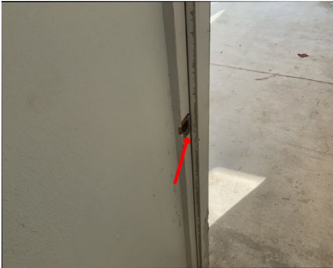
Missing hardware at outdoor bathroom
