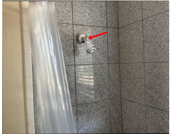
Loose supply line
