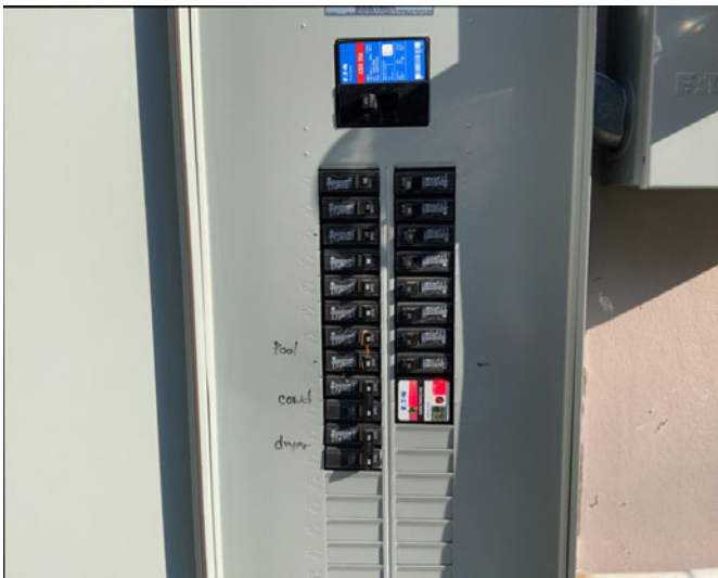
Labeling is required
