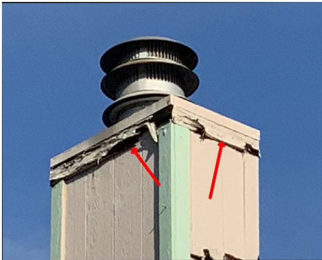
Replace all damaged and decaying trim boards and siding at chimney
