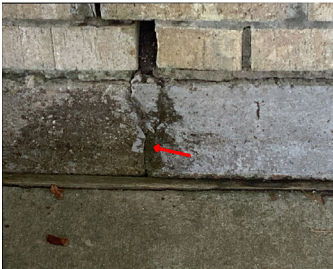
Large crack at right front
