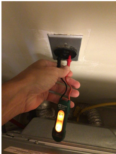
General Photos of Grounding System(s):
