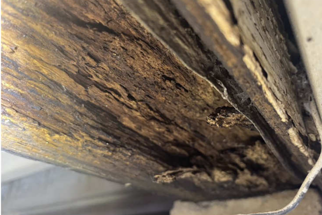
Rotten beam along east perimeter
