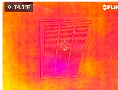
Cooling temperature reading at return
