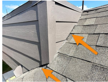
Joint between siding and shingles should not be sealed
