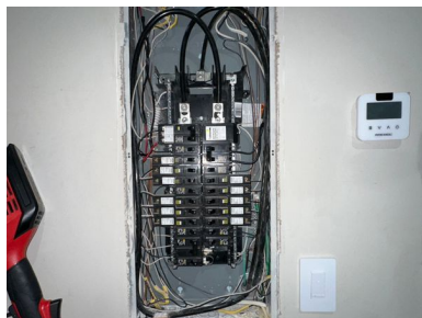
Breaker panel in garage
