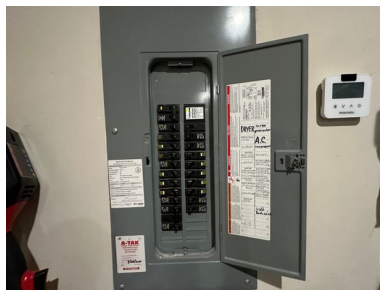
Breaker panel in garage
