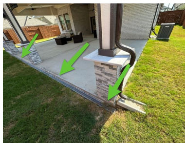
Keep drainage inlets clear of debris
