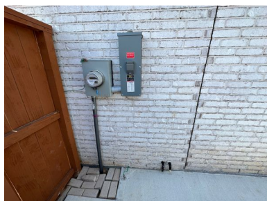
Main disconnect breaker and electric meter located at right exterior wall
