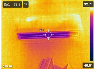
Cooling temperature reading at supply
