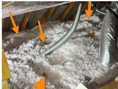
Left side of attic - insulation is uneven, compressed
