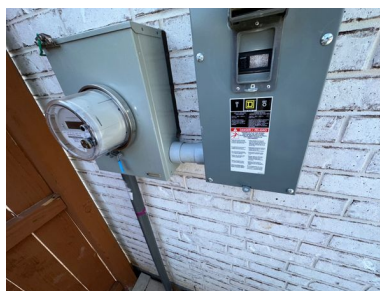
Main disconnect breaker and electric meter located at right exterior wall
