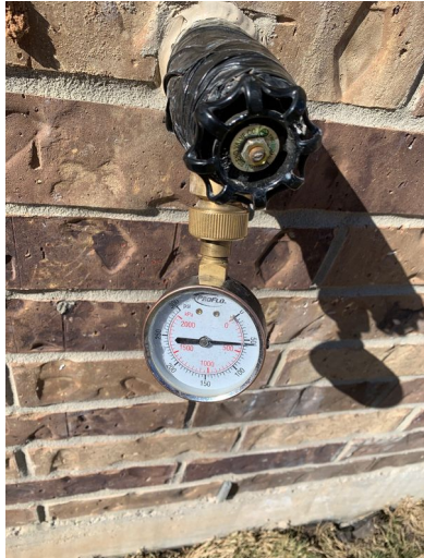
Type of Piping:: PEX
