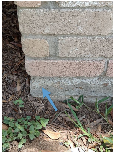
Shear Crack/ Front Exterior
