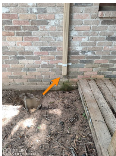
Missing elbow/ rear exterior
