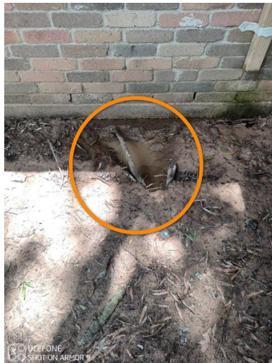
Negative grading / rear exterior
