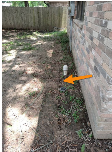
Soil erosion/ rear exterior
