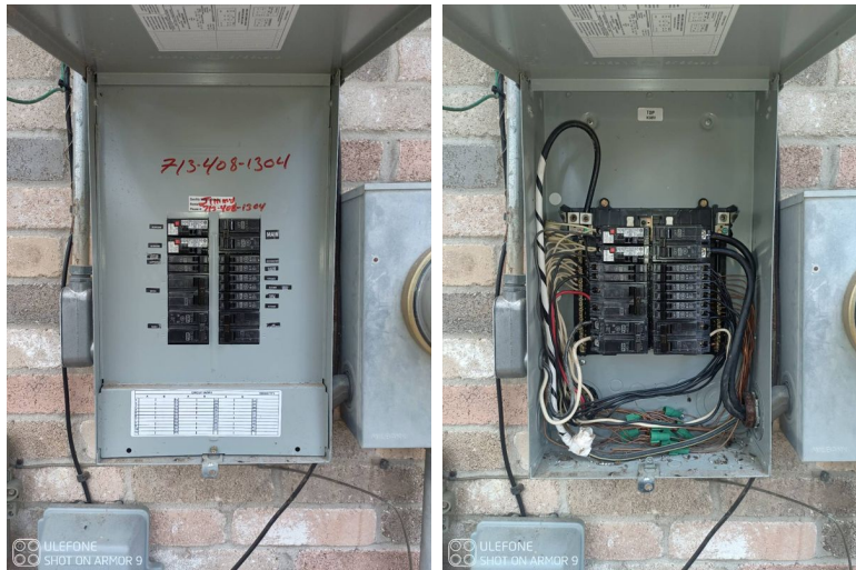
General Infrared Photos of Distribution Panels:
