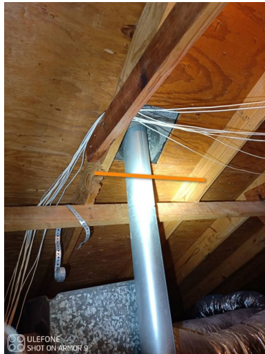
Missing vent strap
