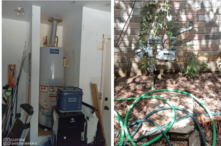
General Infrared Photos of Water Heating Equipment:
