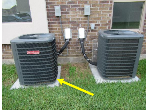
The compressor is not working on the ac unit on the left
