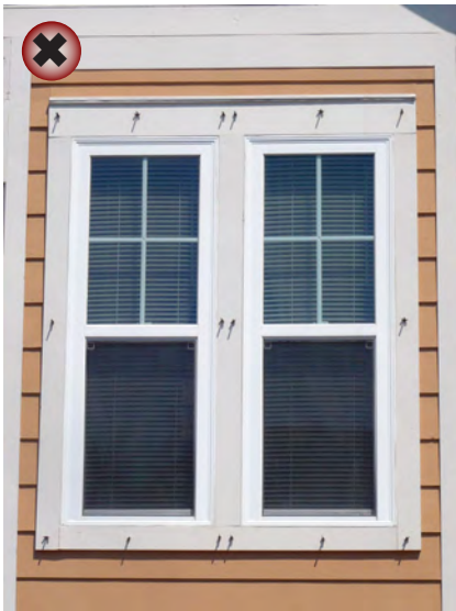
Minimize the visual impacts of anchor bolts on the historic character of the building.
