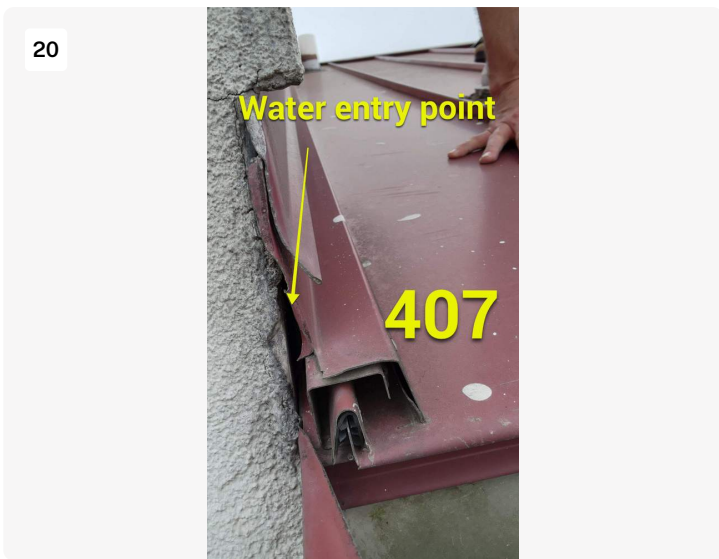
Improper termination of flashing at base of wall.
