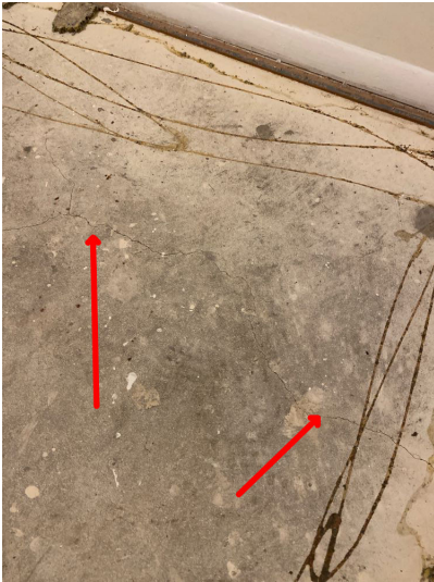
Small crack on the slab in the front middle bedroom
