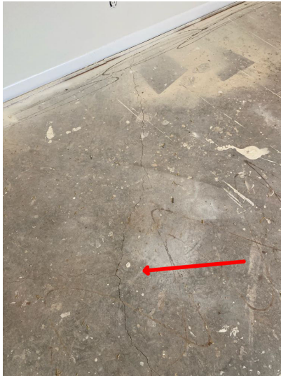
Crack on the slab in the right middle bedroom
