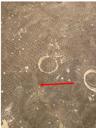
Small crack on the slab in the office
