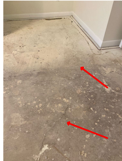
Small crack on the slab in the primary bedroom
