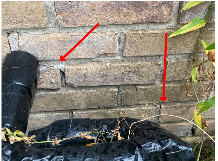
Mortar Crack - front right side of the house
