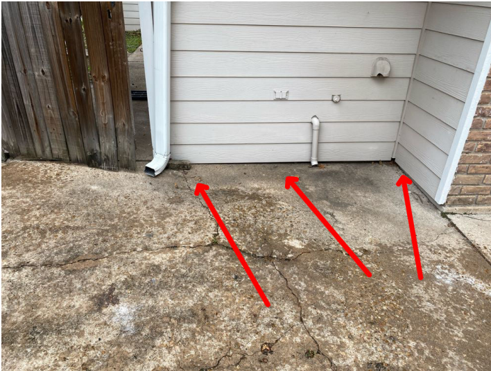
Insufficient Clearance from Ground and Wall Siding
