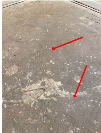
Small crack in the slab in the front right room
