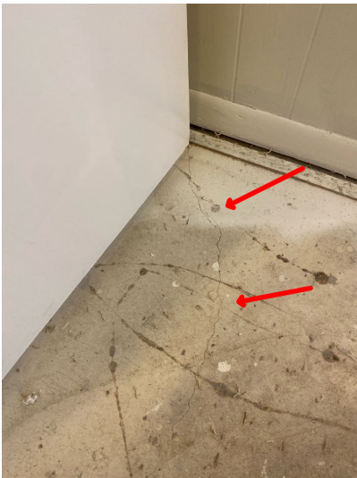
Crack on the slab in the front right bedroom
