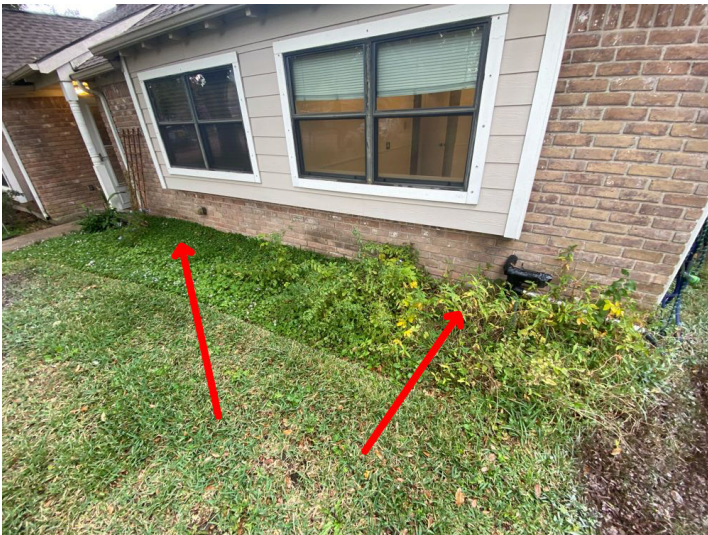
Insufficient Clearance from Ground and Wall Siding
