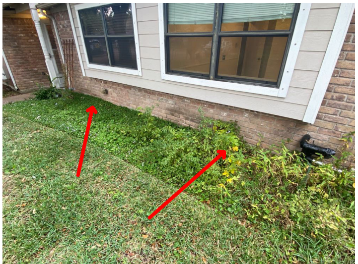
High Soil, Insufficieant clearance to siding
