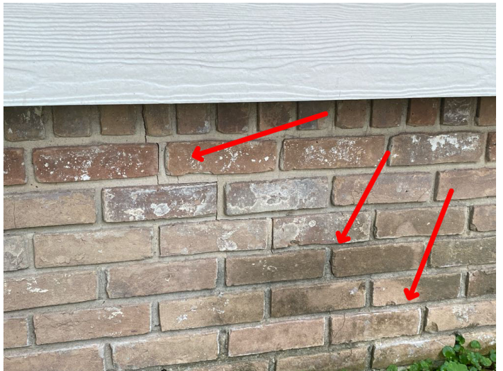
Crack on the brick siding at the front of the house
