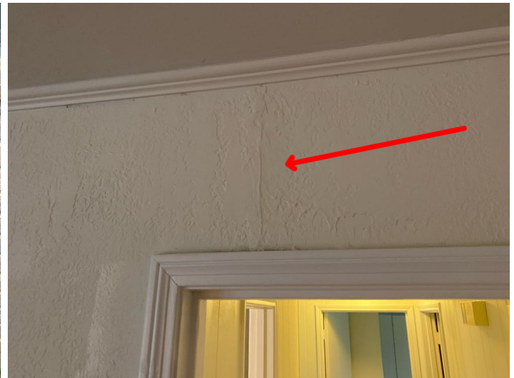
Crack on the drywall in the living room
