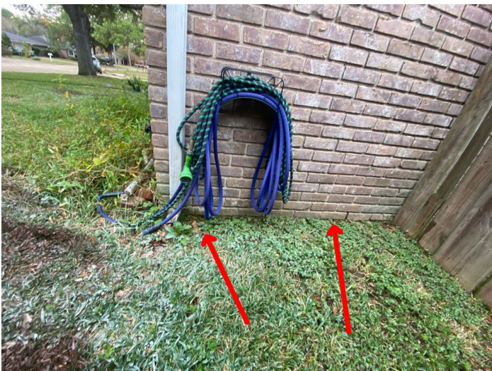
High Soil, Insufficieant clearance to siding
