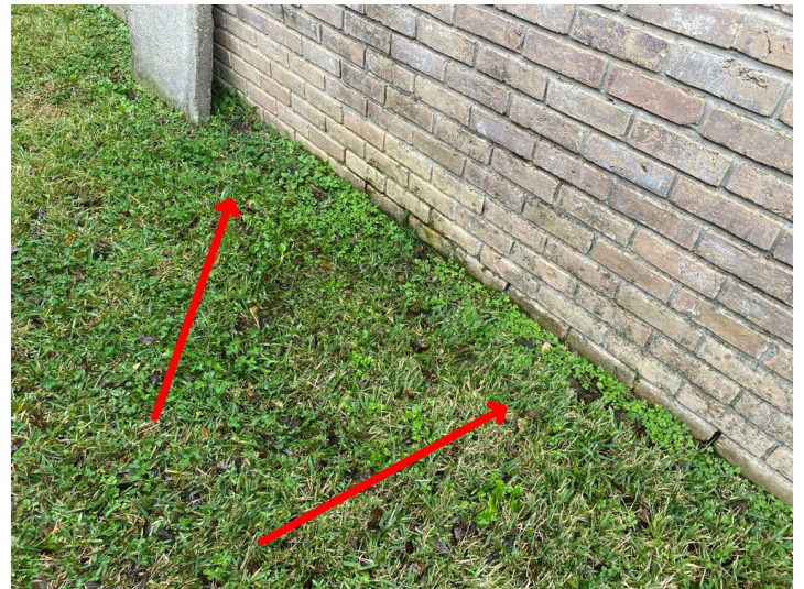
Insufficient Clearance from Ground and Wall Siding
