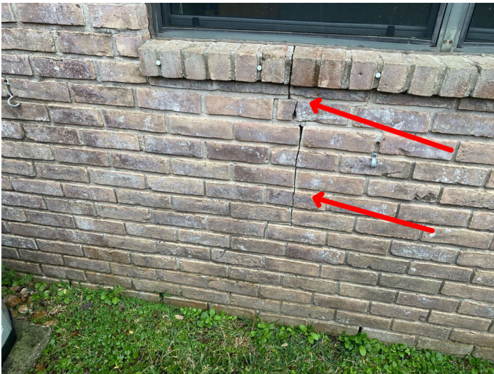
Crack on the brick siding on the right side of the home
