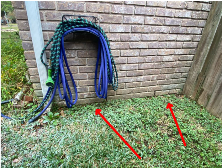
Insufficient Clearance from Ground and Wall Siding
