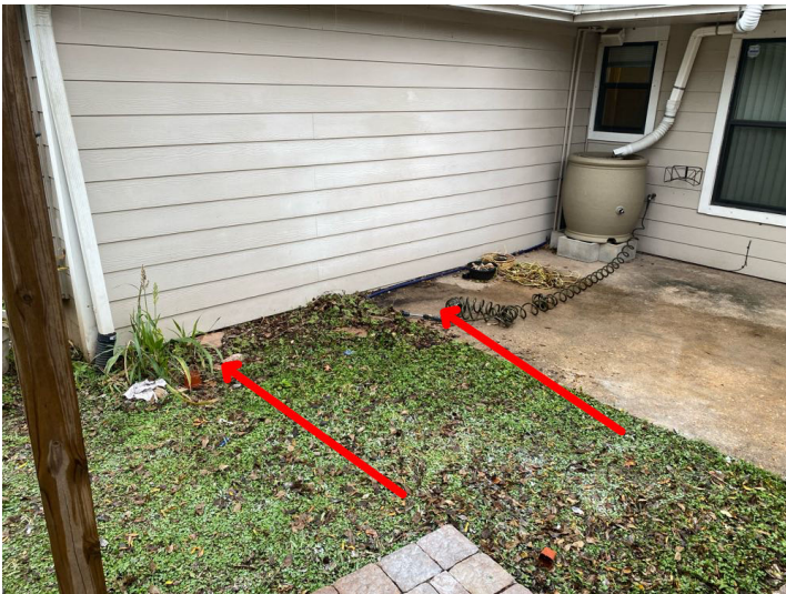
Insufficient Clearance from Ground and Wall Siding
