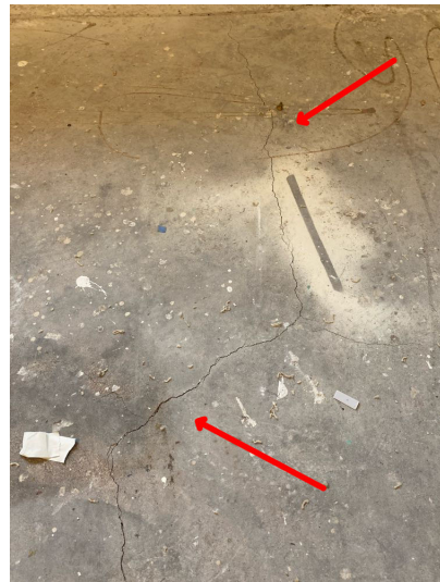
Settlement crack on the slab in the right middle bedroom
