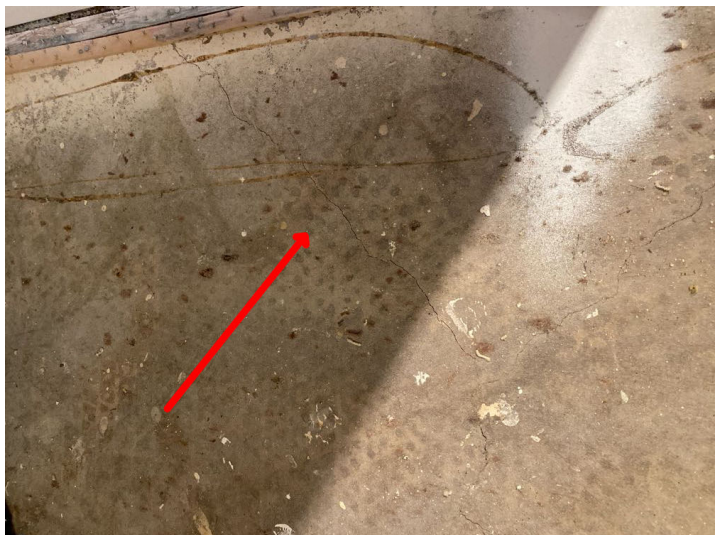
Small crack on the slab in the dining room
